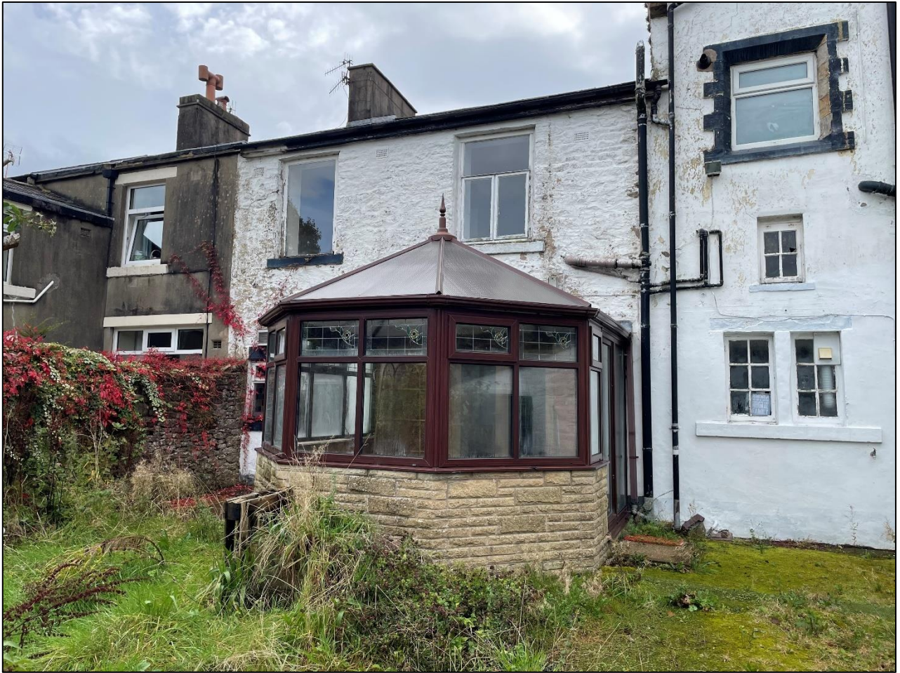
PL03: North west rear elevation of the north eastern half of the building.
