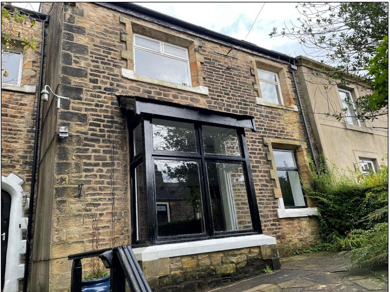
PL02: South east front elevation of the north eastern half of the building.
