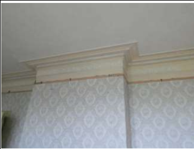
Plaster Cornice, Missing Picture Rail
