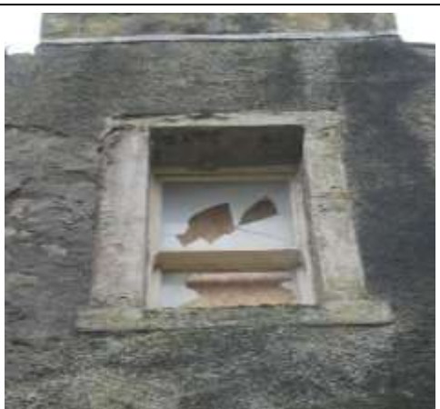
Timber Frame, Broken Pane
