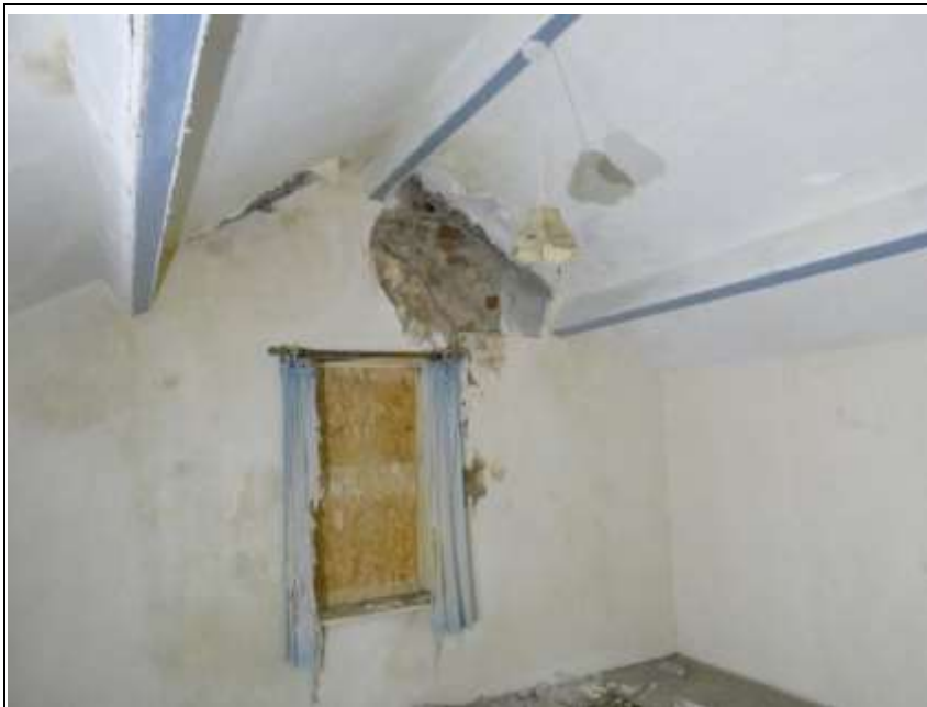
Boarded-up Window at the East Elevation
