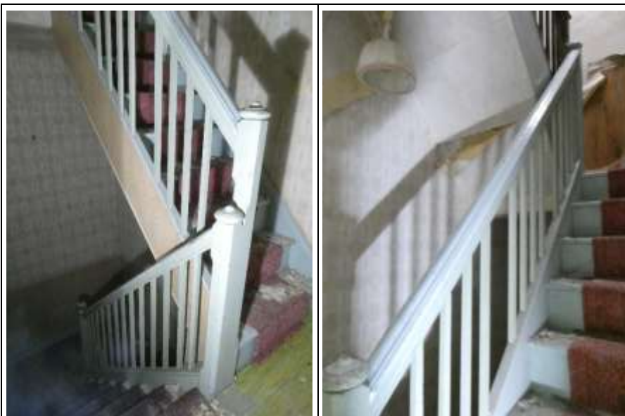
Slender Square Balusters, Some Missing
