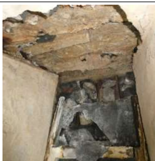
Damage to the Ceiling
