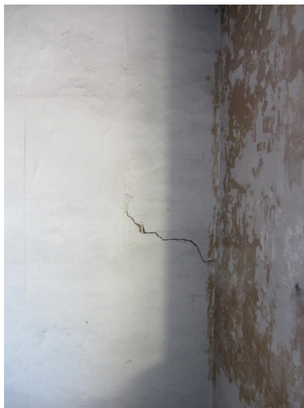
Photo 8 – Crack in internal wall
