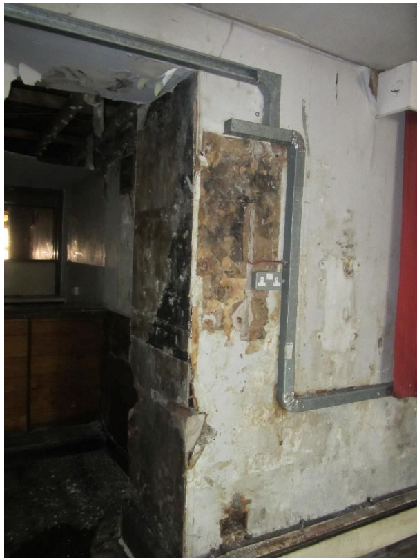
Photo 14 – Ground floor – water ingress
