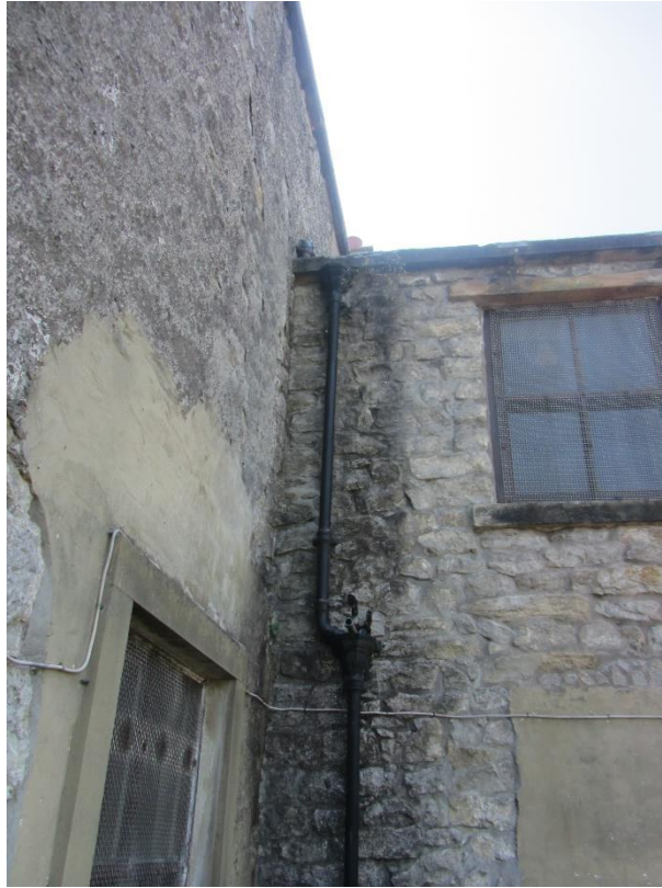
Photo 21 – Leaking gutters and downpipes
