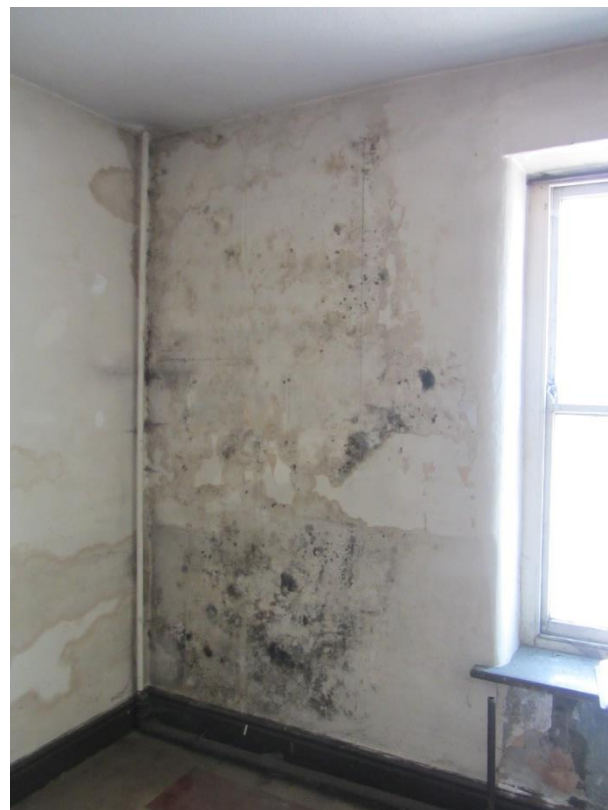
Photo 18 – Ground floor – penetrating damp in west wall
