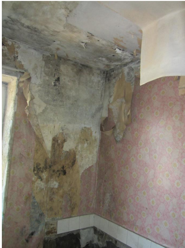
Photo 9 – Water ingress at internal corner
