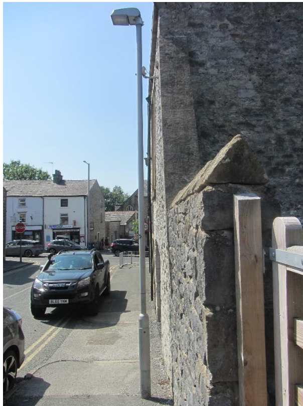
Photo 22 – Outward bow to south wall
