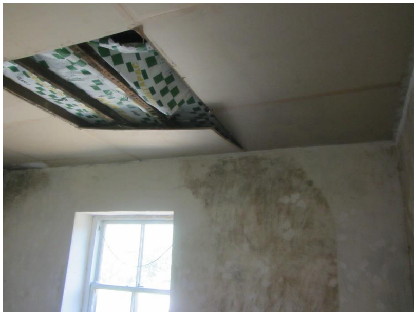
Photo 6 – Penetrating damp; ceiling replaced
