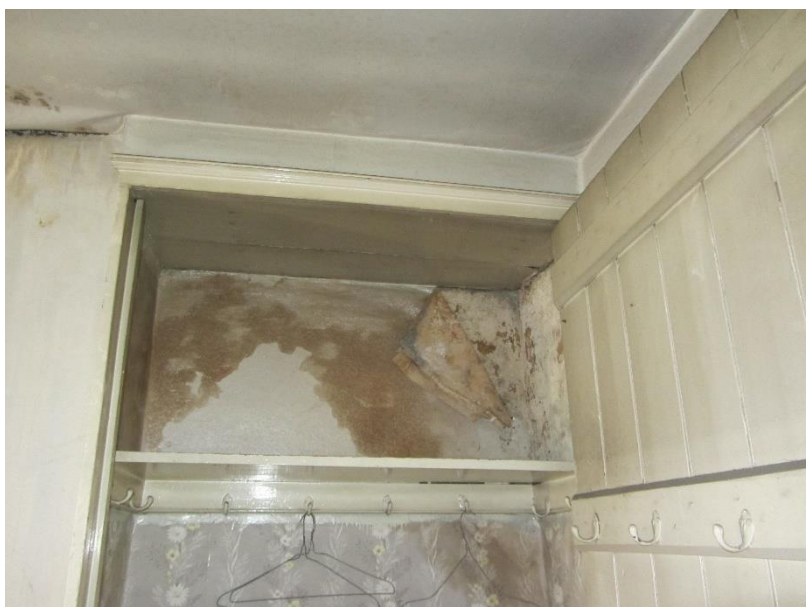
Photo 4 – Damp around chimney breast
