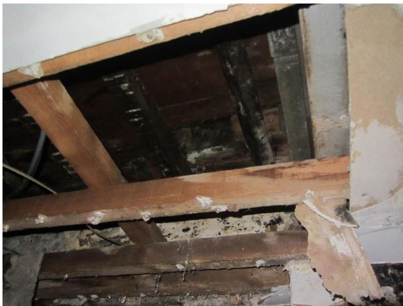
Photo 15 – Ground floor – decayed first floor timbers
