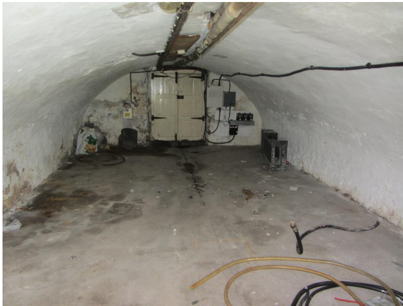
Photo 19 – Cellar – damp patches on floor and walls
