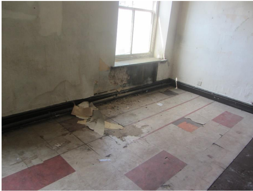
Photo 17 – Ground floor – penetrating damp in west wall
