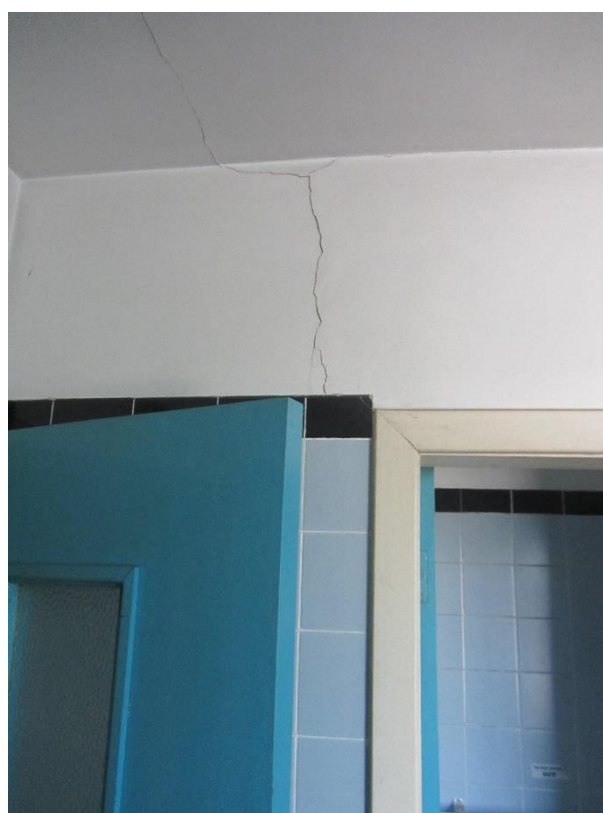
Photo 16 – Ground floor toilets – crack in wall
