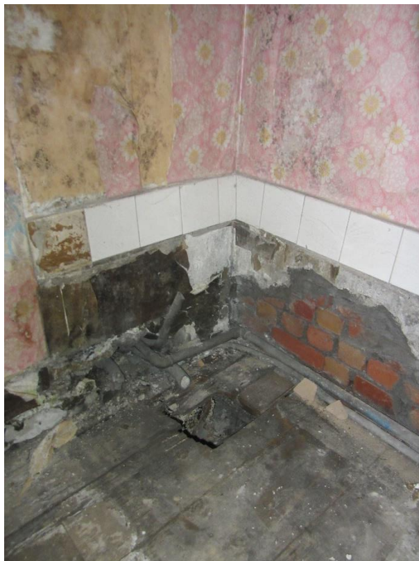
Photo 10 – Decayed floor timbers
