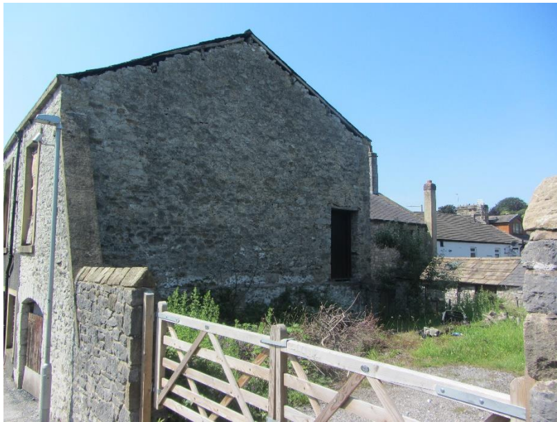
Photo 23 – East wall – gap along roof verge
