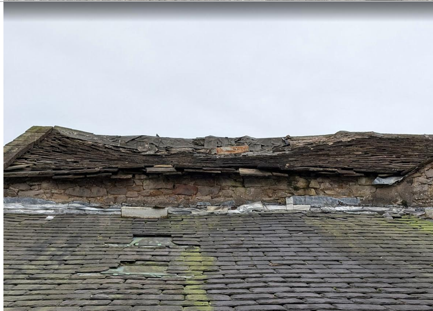
Photo 5. Collapsing barn roof
