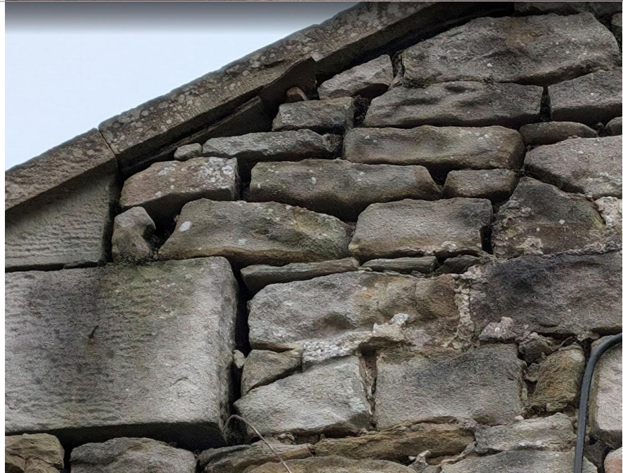
Photos 2a & 2b Examples of gaps in stonework of barn on corner of north- east elevation and along main wall.
