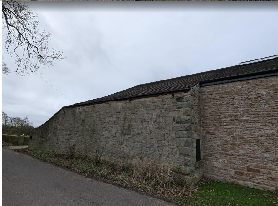
Photos 4a & 4b South-east aspect with gaps under roof verge tiles.
