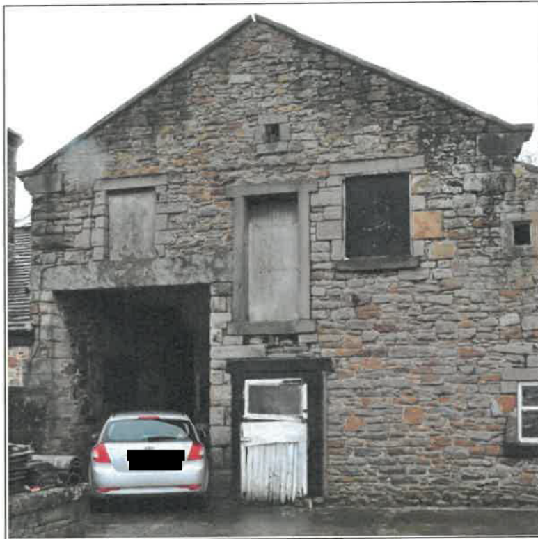
Photo 3: Gabled wing in north-west elevation of barn, containing cart entrance and doorways to stable and hayloft
