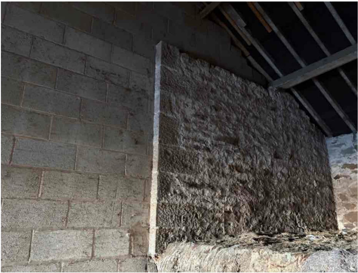
Photo 27 - Loft area adjacent to south east elevation with old and new sections of north east elevation
