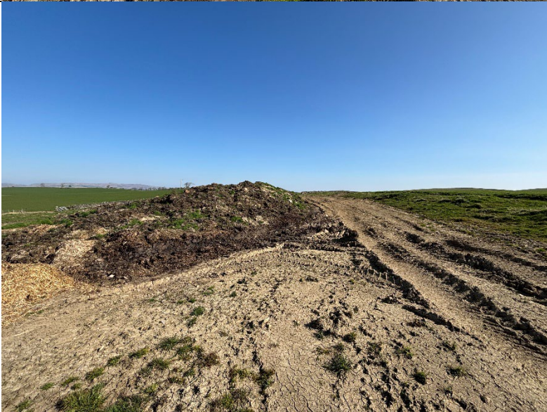
The core development area is heavily tracked/rutted and topped with a muck heap
