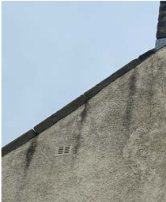
Photo showing open joints to gable copings, with resulting running water down and behind render and poor condition of coping where abuts chimney.
