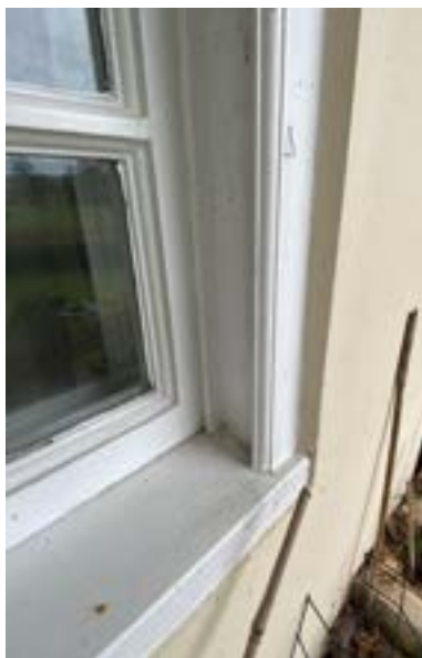
Photo 12: Typical external view of kitchen window proximity to front render face.
