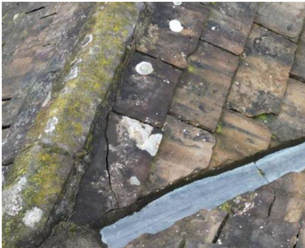
Photo 5 – Broken apex tile.
