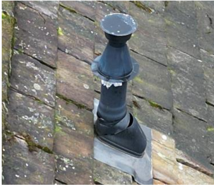
Photo 6 – Slipped flue housing
