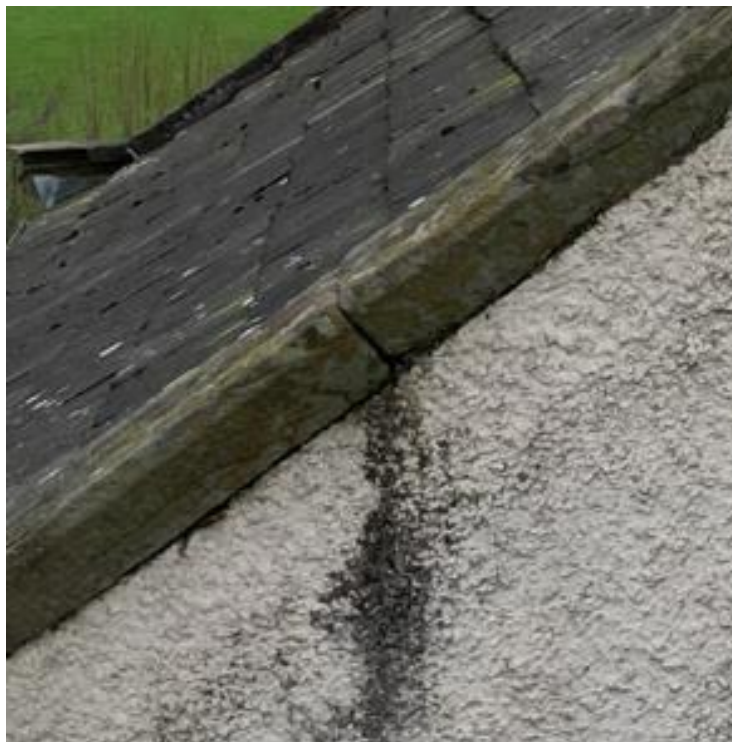
Photo 2 – Staining on render at coping stone joint
