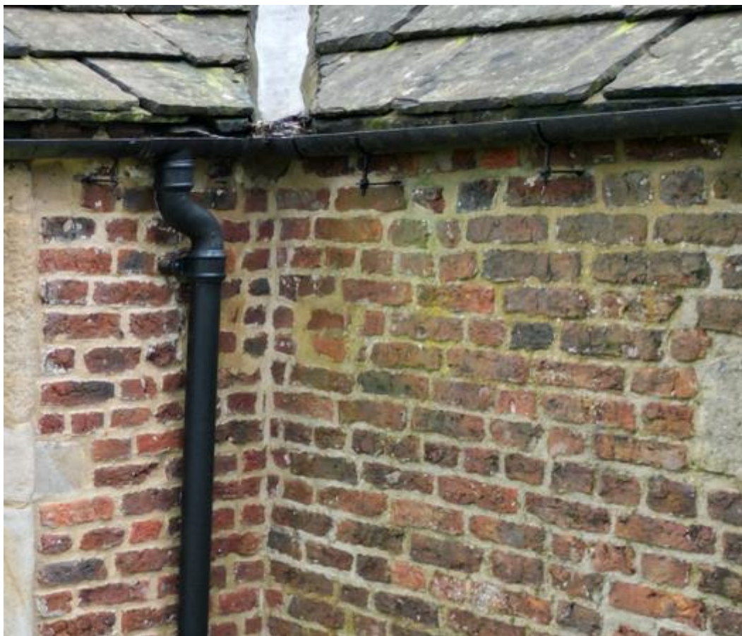
Photo 6 – Stained wall likely due to gutter overspill
