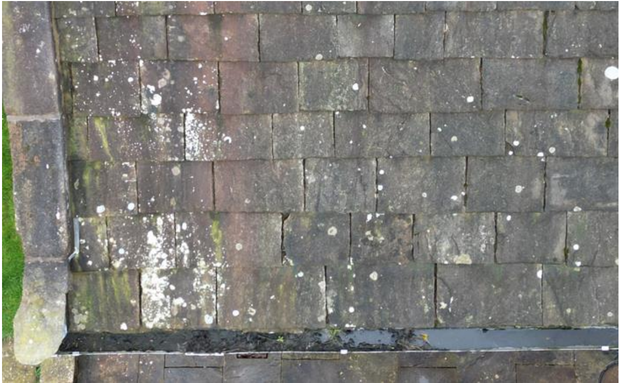
Photo 2 – Completely blocked water outlet in gutter
