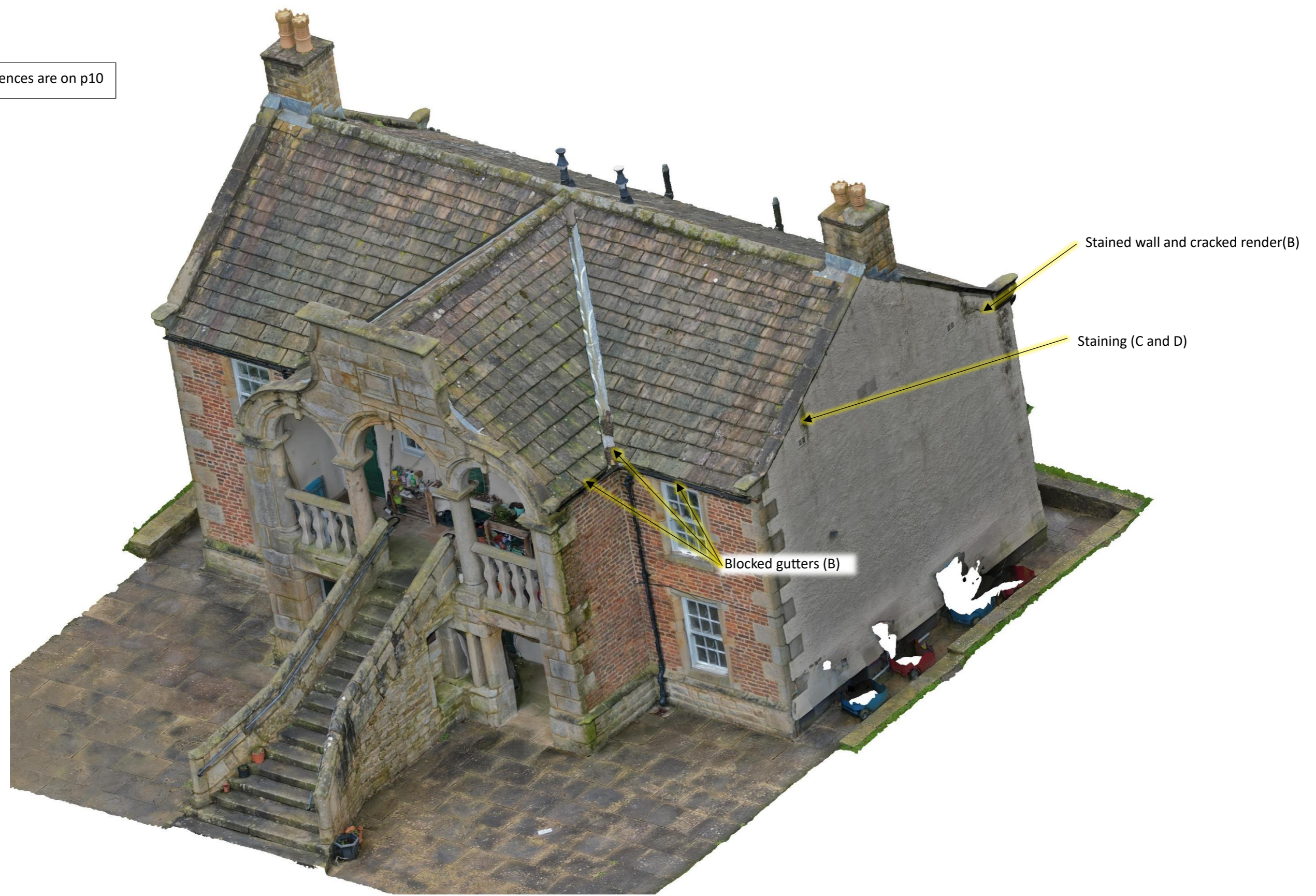
Photo 10 Visual summary of defects
