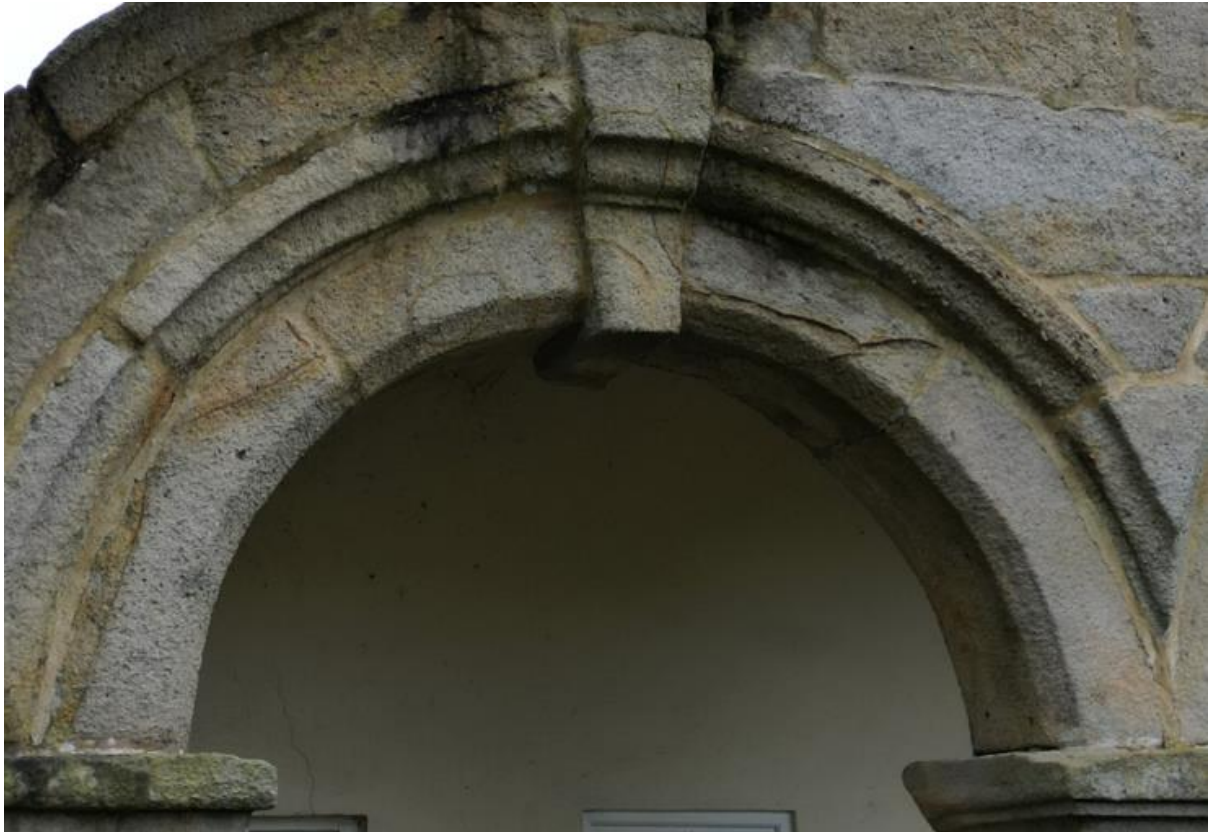
Photo 5 – Possible previous repairs and discolouration to sandstone
