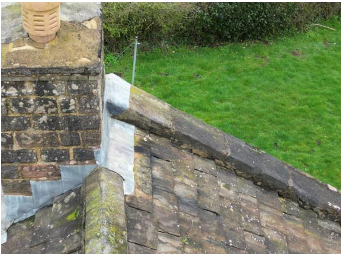
Photo 7 – Poor mortar condition beneath coping stones
