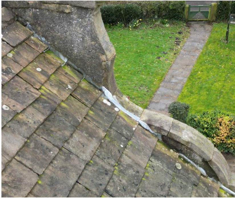
Photo 3 – Poor or missing lead soaker
