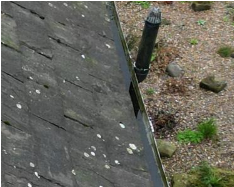
Photo 1 – Ponding water in gutter
