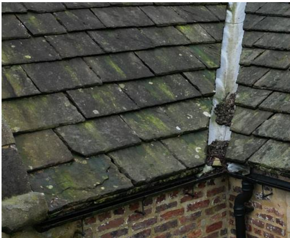
Photo 3 – Blocked valley gutter
