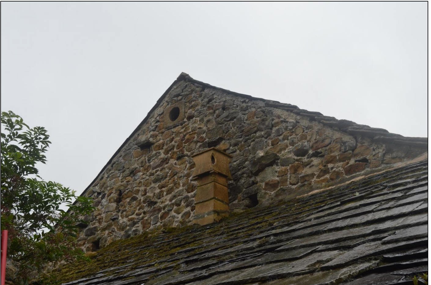
PL21: View of the exposed north east gable end of the barn from the north west.
