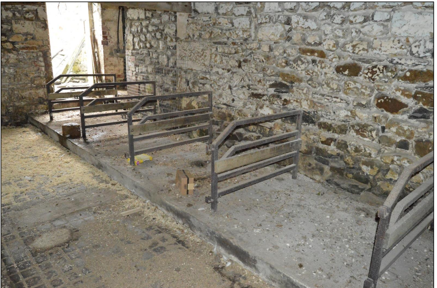
PL46: View of the stalls to the east side of the shippon [GF-03].
