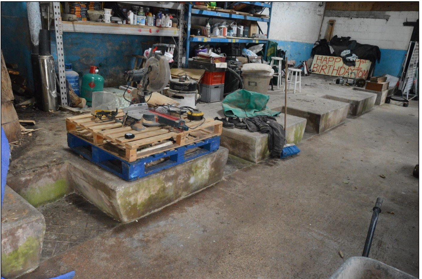
PL71: View of the concrete floor and milking step within the former milking parlour [GF-08].
