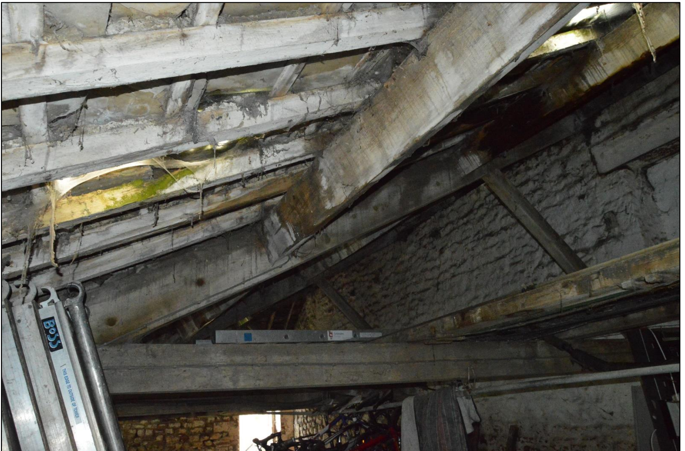
PL48: View of the lean-to roof trusses and associated roof structure to the shippon [GF-03].
