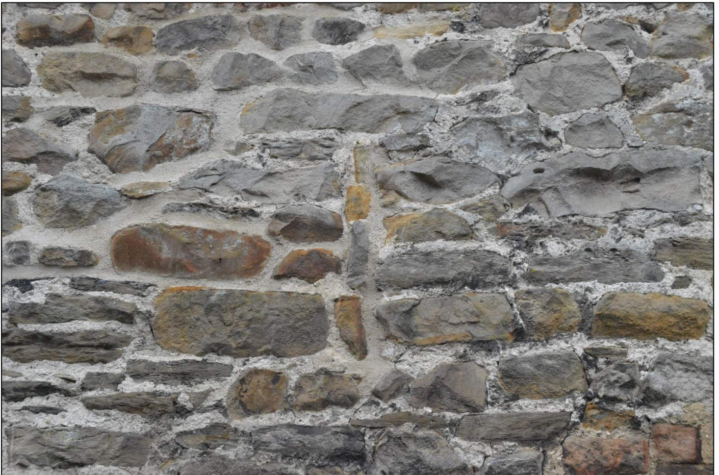
PL06: View of blocked breather to the south east elevation of the barn.
