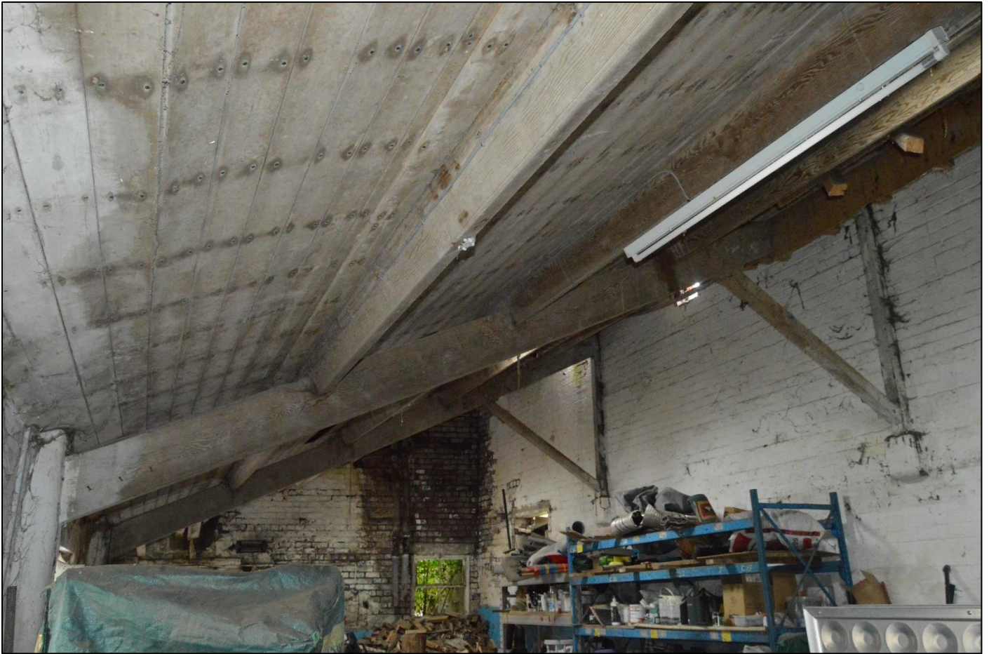
PL74: View of the timber roof structure over the former milking parlour [GF-08].
