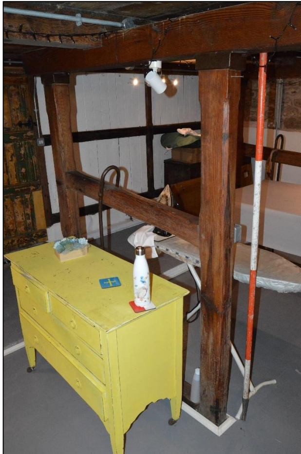
PL26: View of a timber boskin within the former shippon to the south end of the barn [GF-01].
