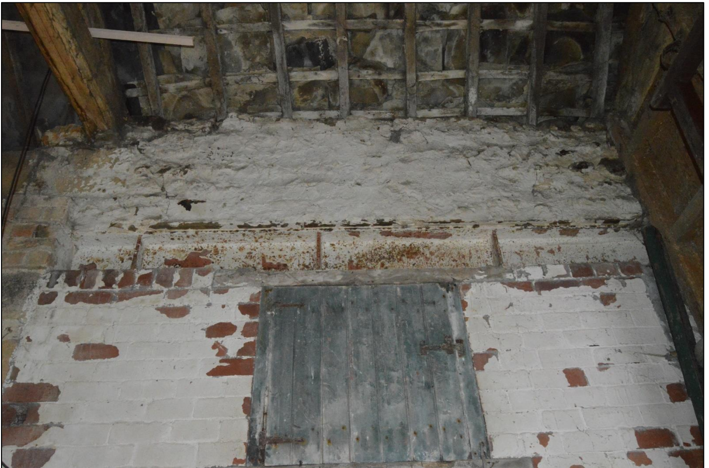
PL37: View of steel beam located above the possible forking hole to the north west side of the barn core.
