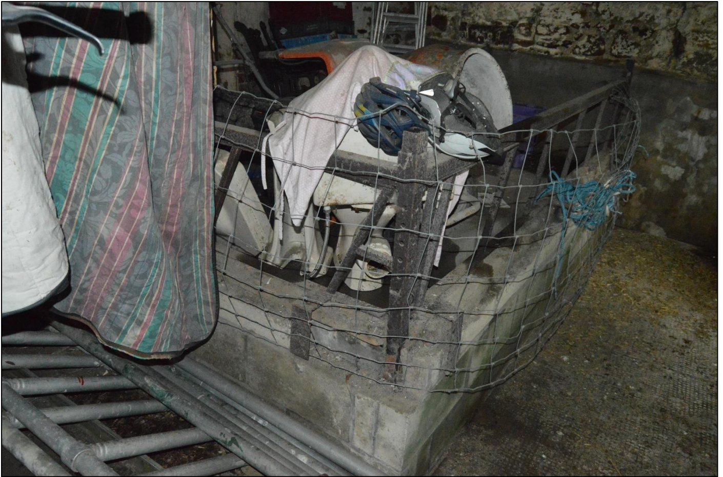
PL42: View of the raised concrete floor to the south end of the shippon [GF-03] leading from the core of the barn.
