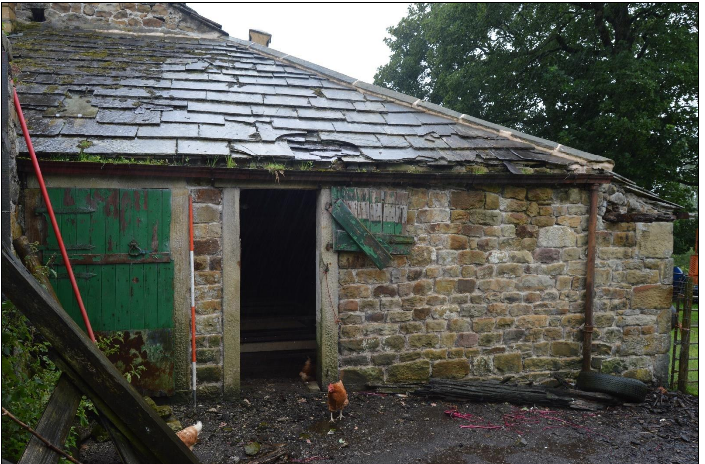
PL18: View of the north east elevation of the shippon to the north west side of the barn.
