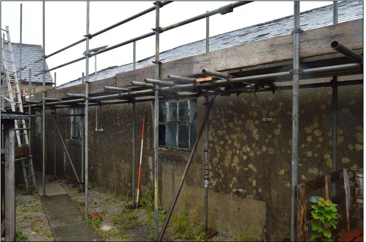
PL66: View of the south elevation of the former ming parlour [GF-08] and wood store [GF-09] from the east.
