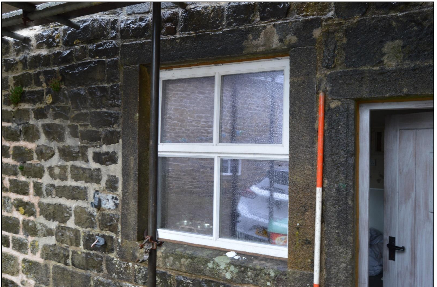
PL57: View of the window to the south west side of the wash house [GF-11].
