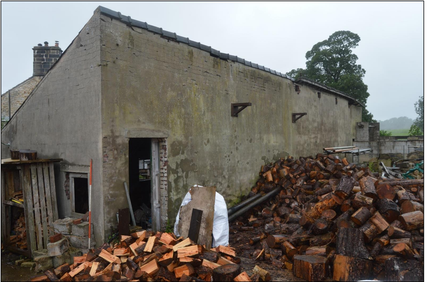
PL68: View of the north elevation of the former milking parlour [GF-08] and wood store [GF-09].
