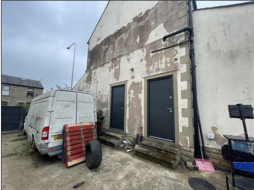
Plate 3 – Location of the proposed single-storey rear extension, noting the lack of PRFs to this elevation
