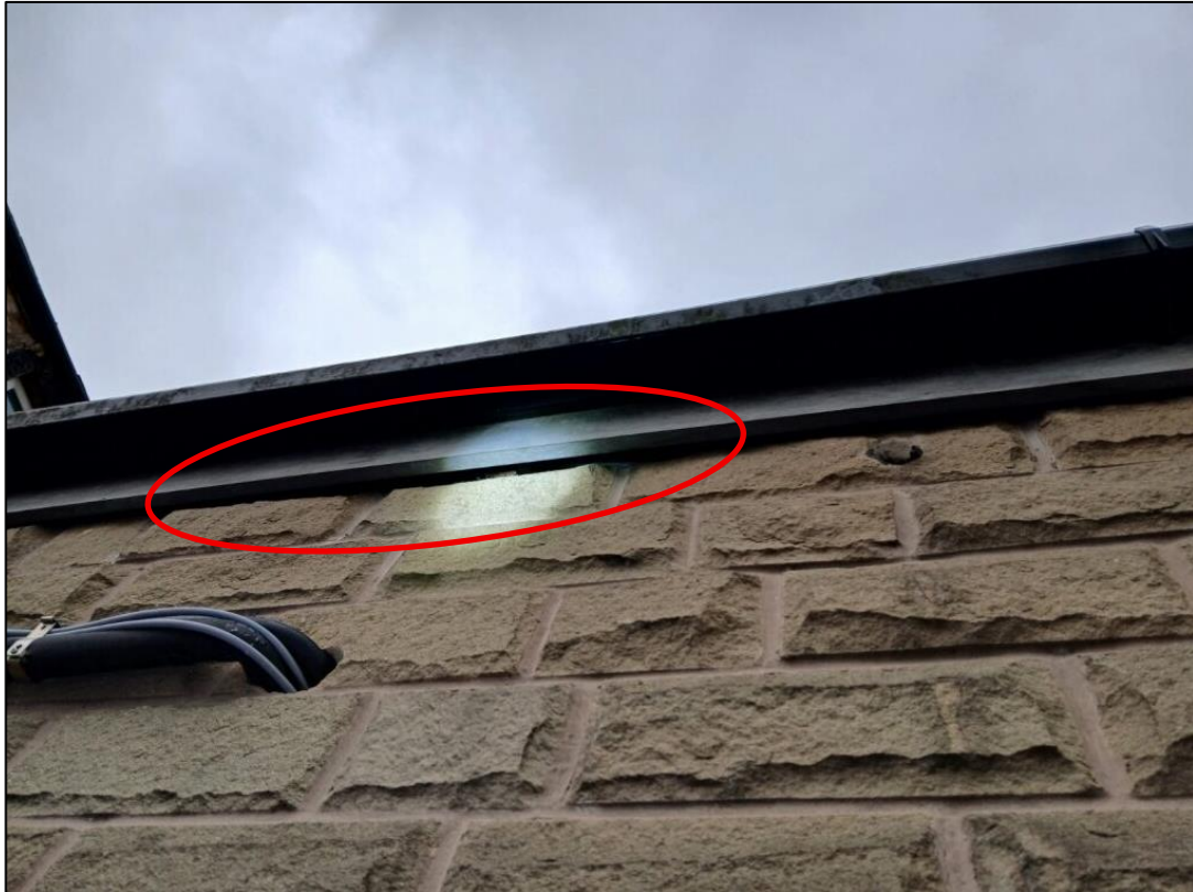
Plate 5 – Gaps under the barge board found on the south elevation of the side-extension; PRF highlighted in red
