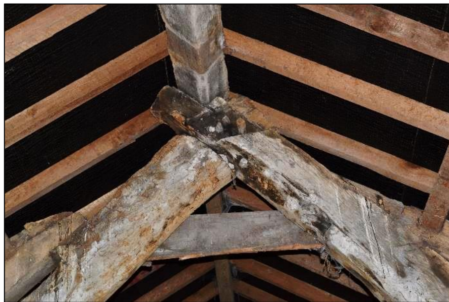
Plate 22. Showing pegs in cruck and ridge purlin
