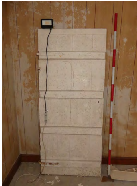
Plate 37: Loose door in G3 (farmhouse)
