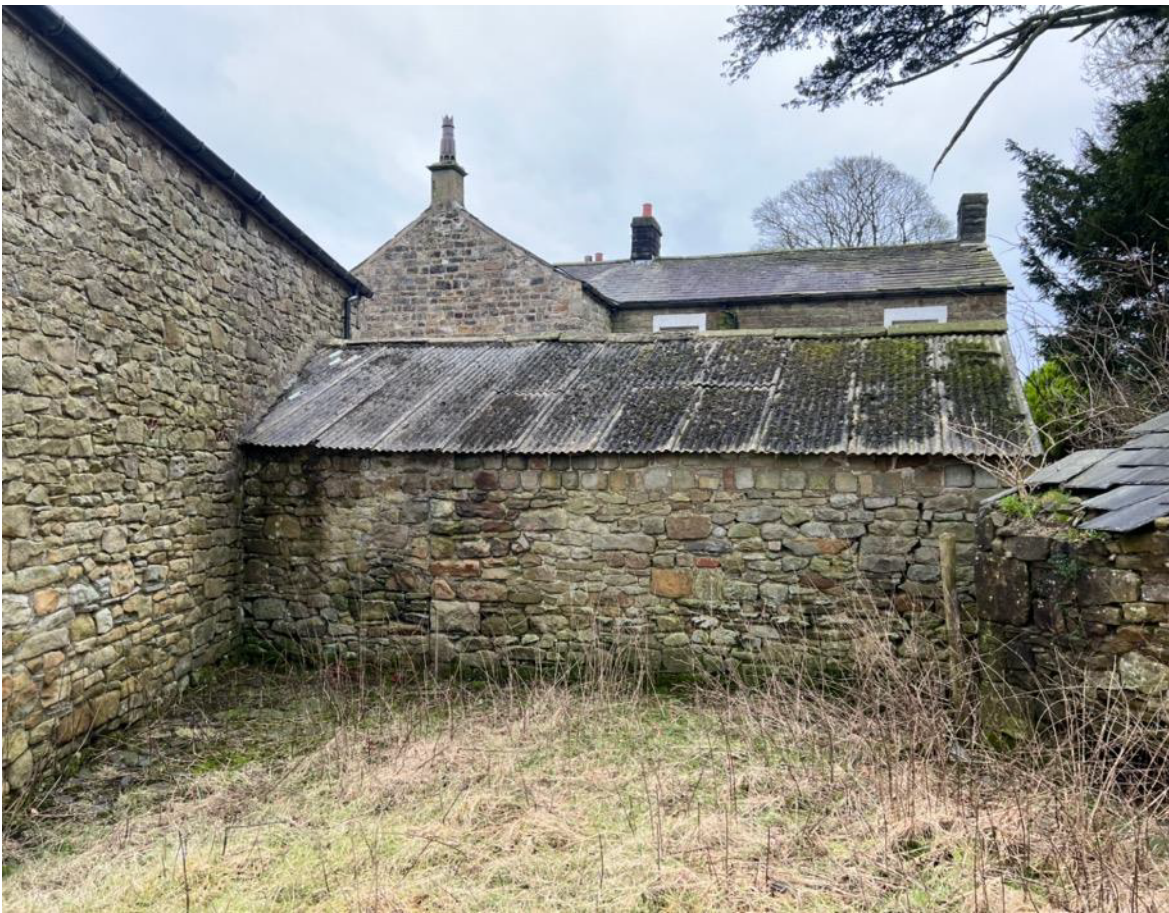
Photo 19 – North West of main barn and North East of outrigger with roof
