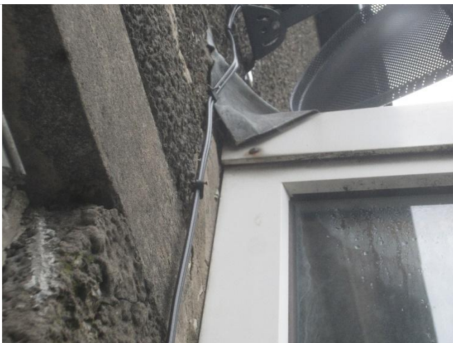
Photo 11: Gap at lead flashing at PVC conservatory
