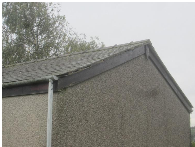
Photo 25: Gaps at roof verge on western elevation of garage
