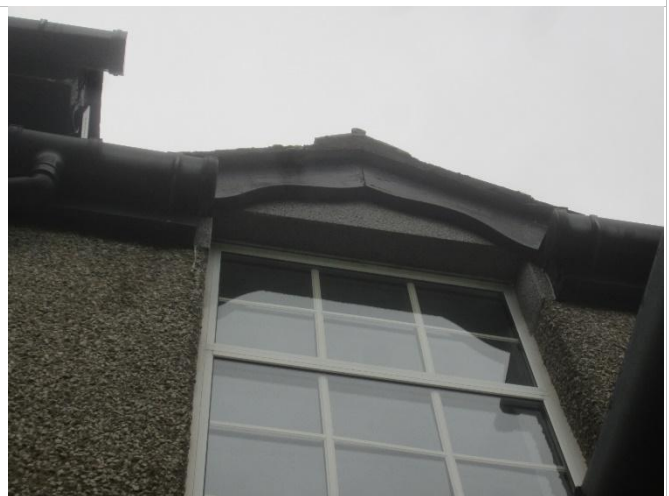
Photo 12: Gaps behind timber fascia at eastern section of farmhouse
