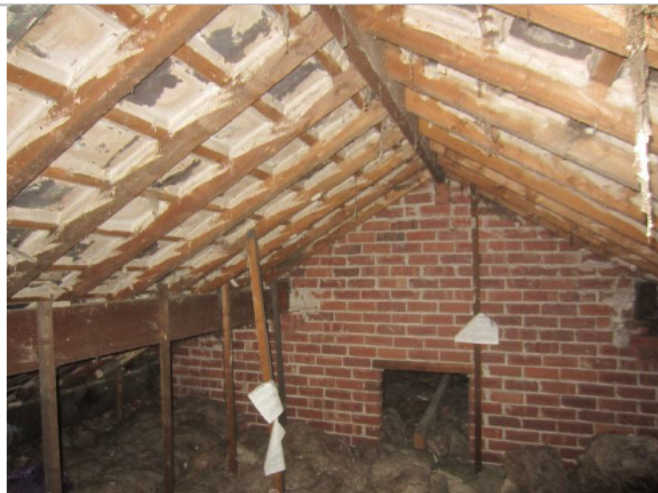
Photo 17: Roof void at the south-western end of the western section of the farmhouse
