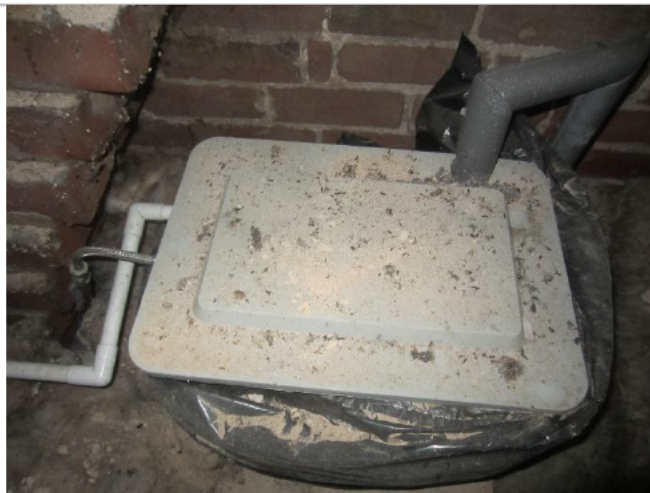
Photo 18: Bat droppings over hot water tank on internal side of fascia and wall at Roost 1
