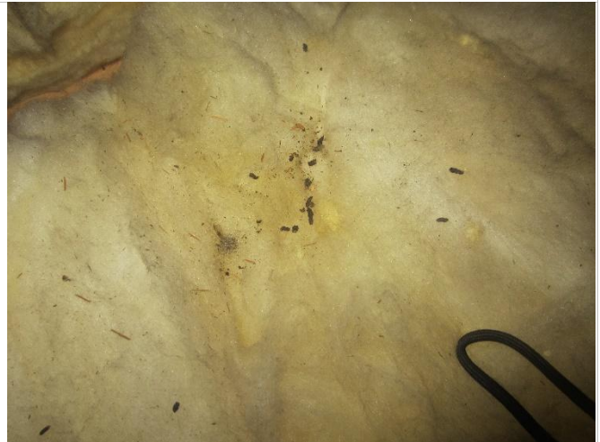
Photo 22: Bat droppings (common pipistrelle) on fibreglass insulation on floor of eastern election of roof void
