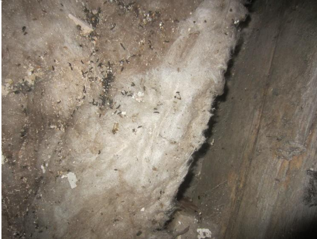
Photo 19: Bat droppings (common pipistrelle) on fibreglass insulation on floor of roof void at western section of farmhouse
