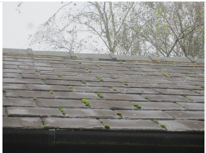
Photo 8: Slate roof over utility area with sections of missing bedding mortar beneath the ridge copings
