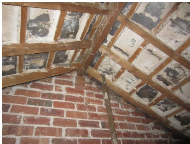
Photo 15: Roof void at north-eastern end of the western section of the farmhouse
