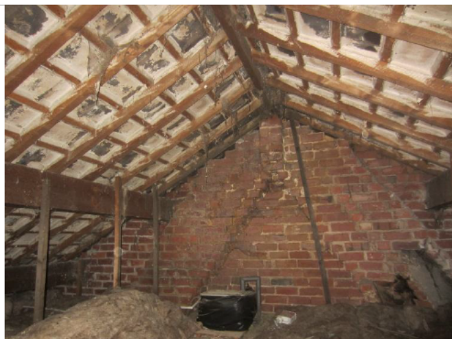
Photo 15: Roof void at north-eastern end of the western section of the farmhouse
