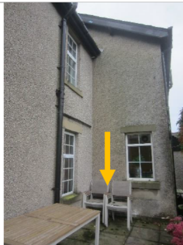
Photo 14: Scattered bat droppings over chairs beneath the north-eastern elevation of the western section of the farmhouse and assumed roost access to Roost 1
