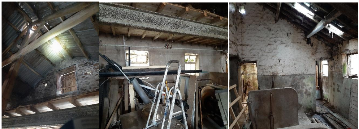
Figures 6-8: From left to right, upper space in main barn area, lower space in main barn area, and internal space in lean-to area.
