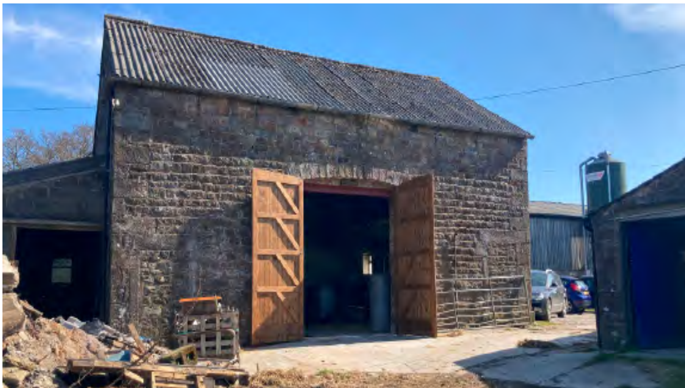
Main south elevation of the barn; showing recent threshing doors in the original opening and stoned up byre doors to either side. Consent for threshing doors included retrospectively.
