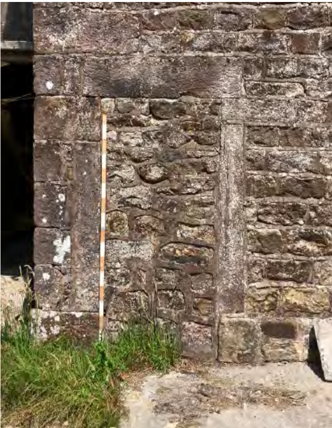
Blocked left hand / west byre door
