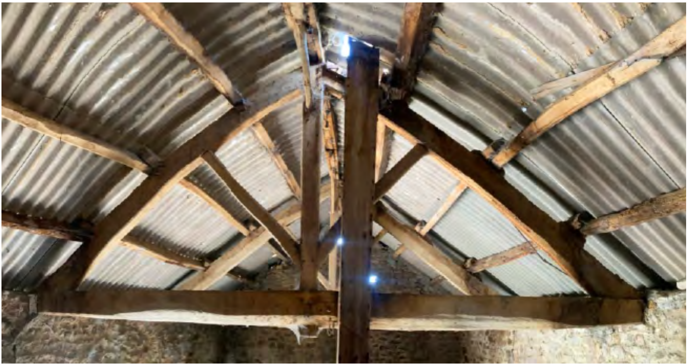
East and west king post trusses viewed from the east with remaining purlins and asbestos and fibre cement sheet roofing over.
