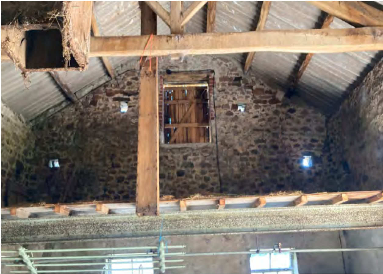
View to east side of the main barn from the central threshing floor. C20th hayloft over on steel beam. Note C20th plasterwork to the walls of the byre and exposed rubble work above, with diagonal crack to upper left hand side reflecting crack externally.
