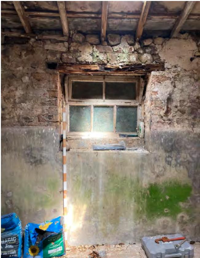
Window to north wall of north shippon with lower cementitious plaster and limewash above. Also note decay to the timber lintel.
