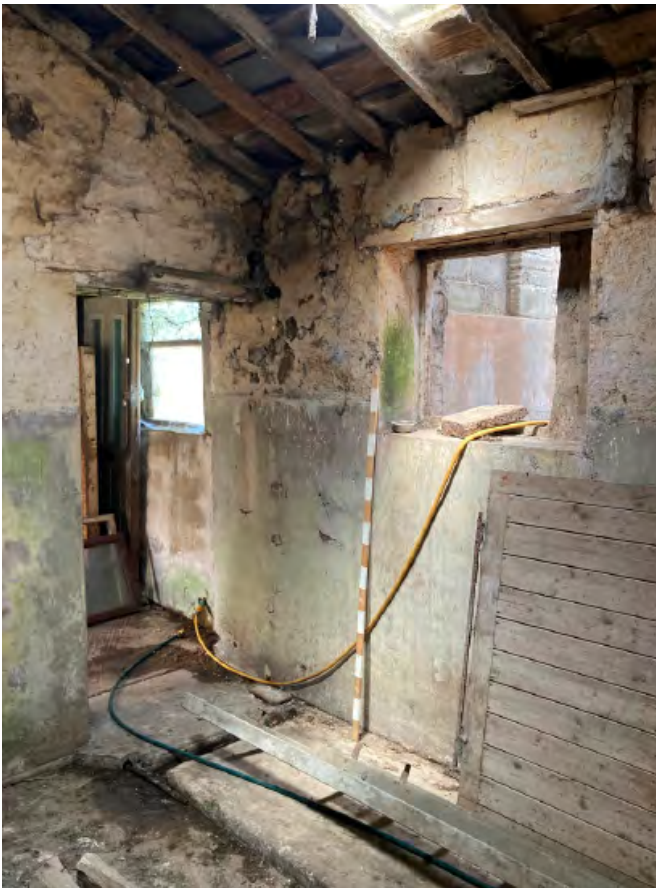
Northwest corner of north shippon, with doorway to C20th shippon to left and window opening to modern barn to the north. Note mix of cementitious plaster and earlier layers of limewash to the walls.
