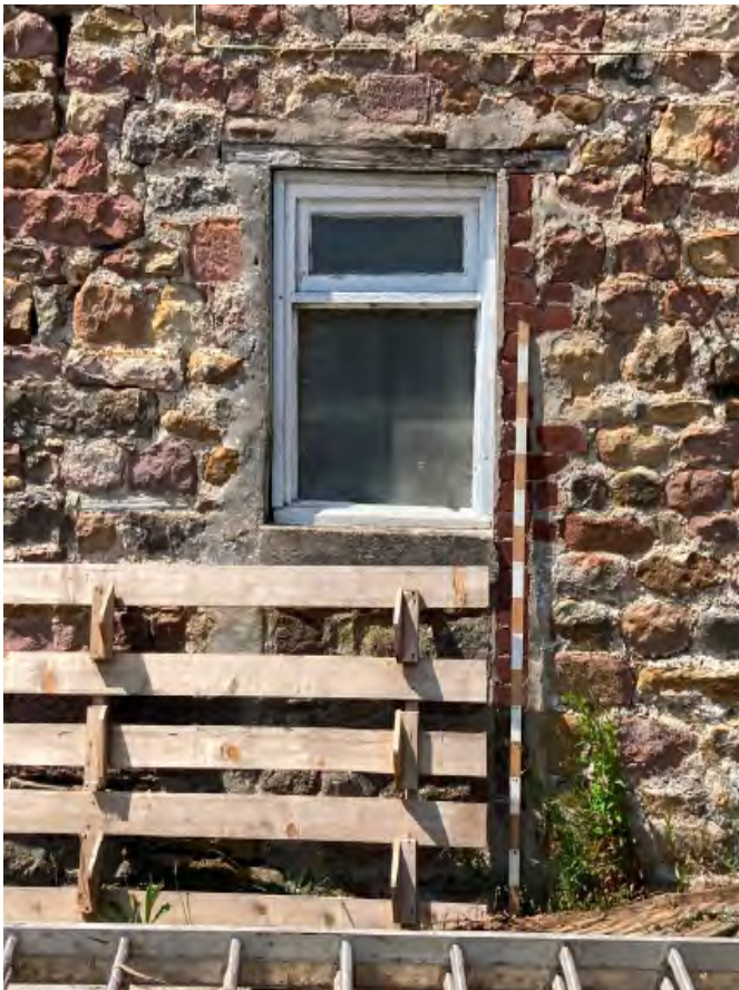
North window to east elevation within earlier door opening. Concrete cill and cement render over brick jambs and timber lintel.
