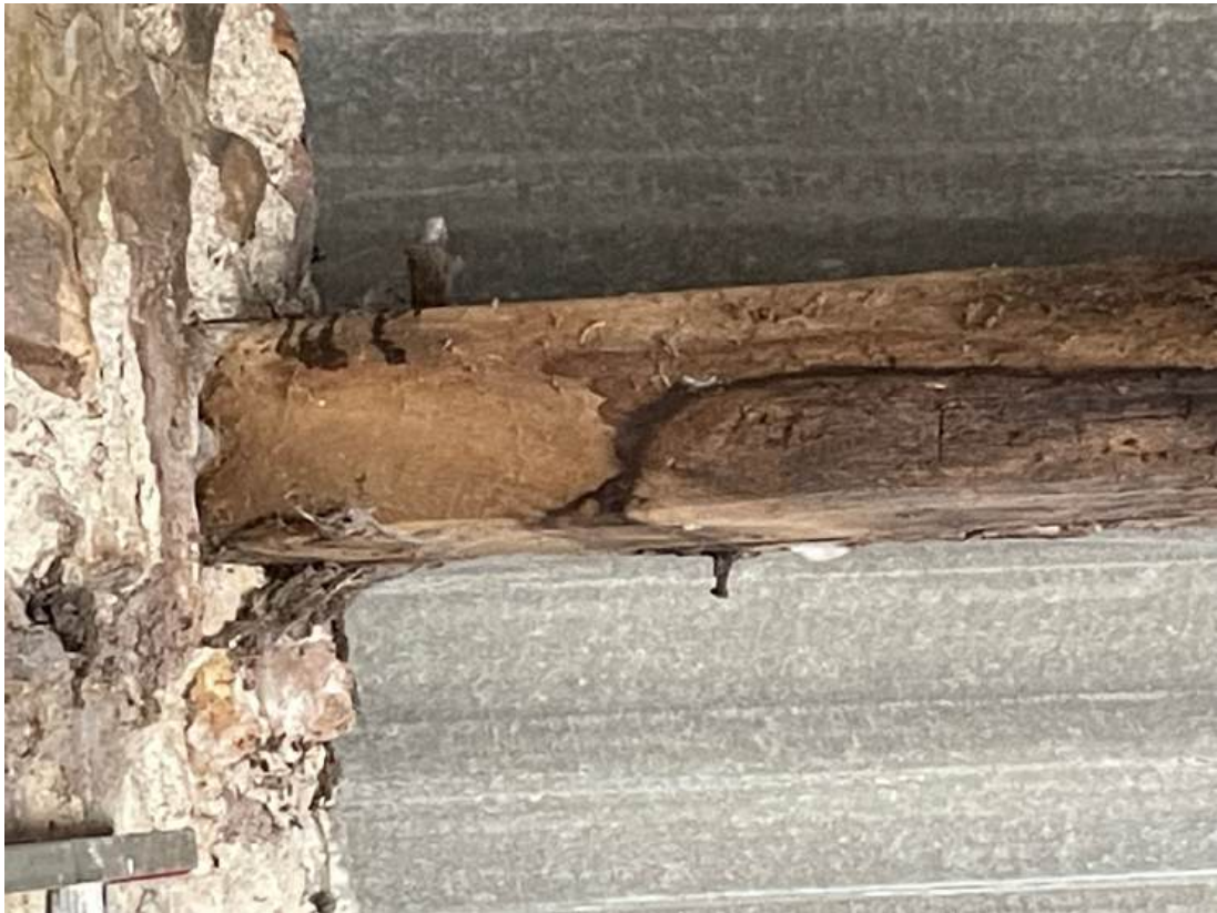
Photo Four: Main Barn – Split in Oak Truss
