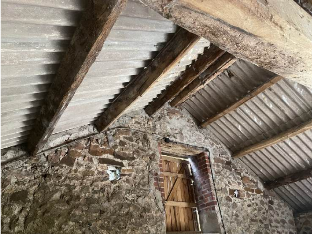
Photo One: Main Barn - Righthand Side of Roof
