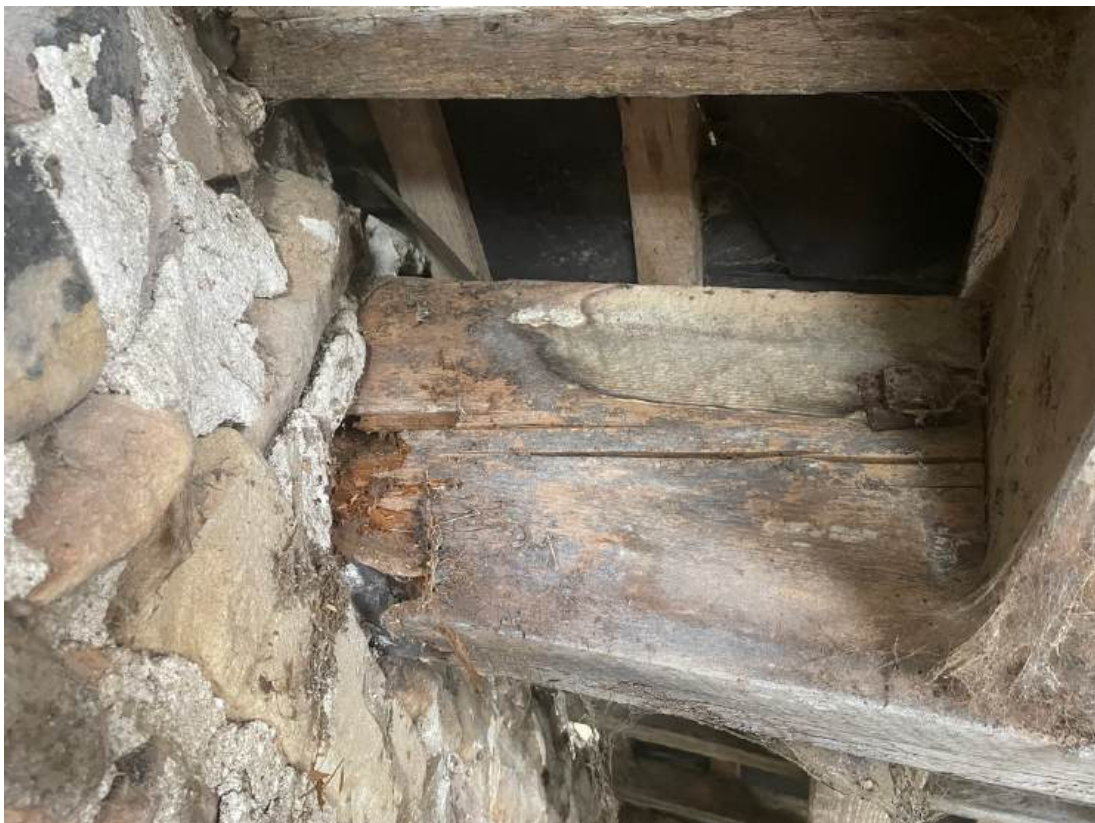
Photo Six: Shippon – Rotten End of Truss
