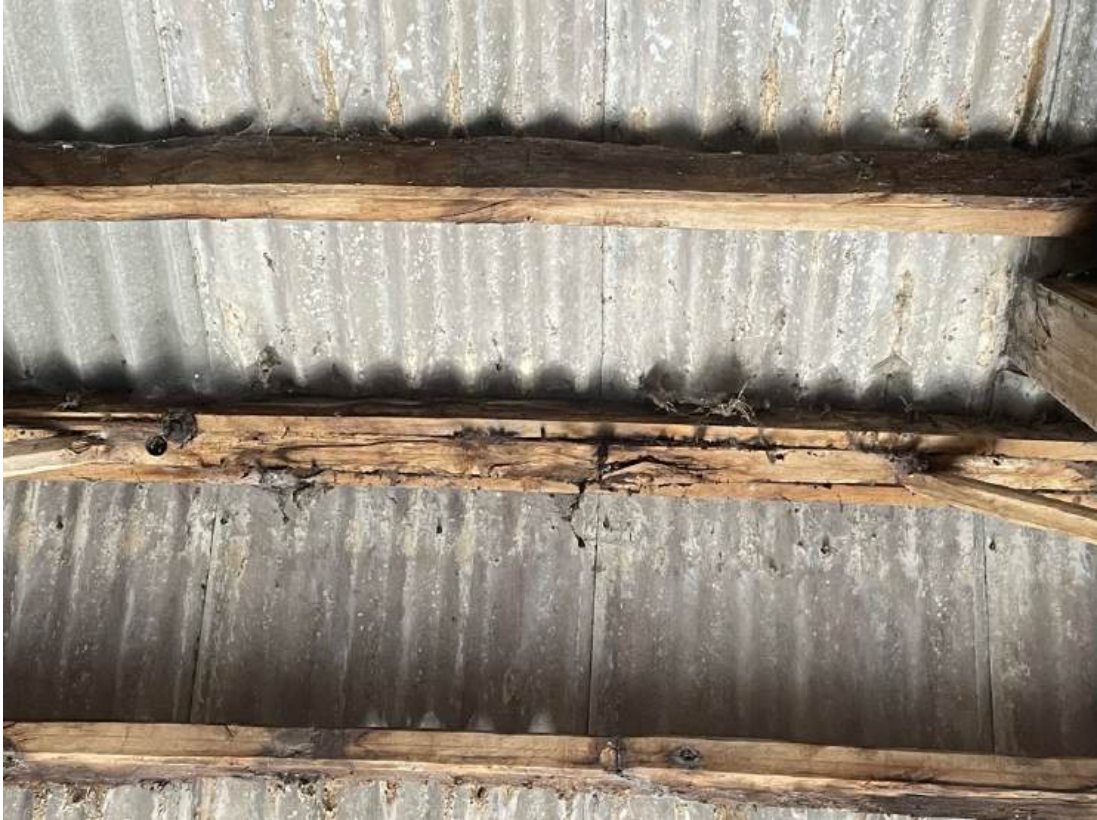
Photo Three: Main Barn – Rotten Ridge
