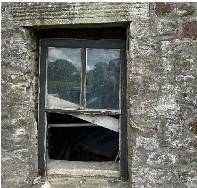
Figure 13 Rubble cavities accessible through dislodged window frames
