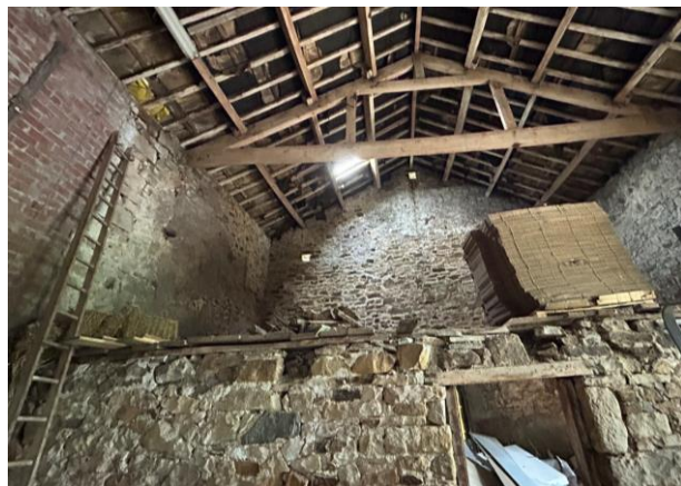
Figure 10 Interior of B3 supporting numerous PRF's
