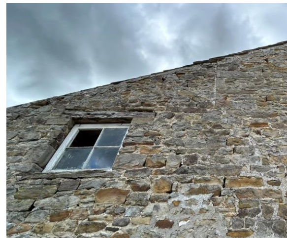
Figure 12 PRFs in B3, broken windows and missing mortar
