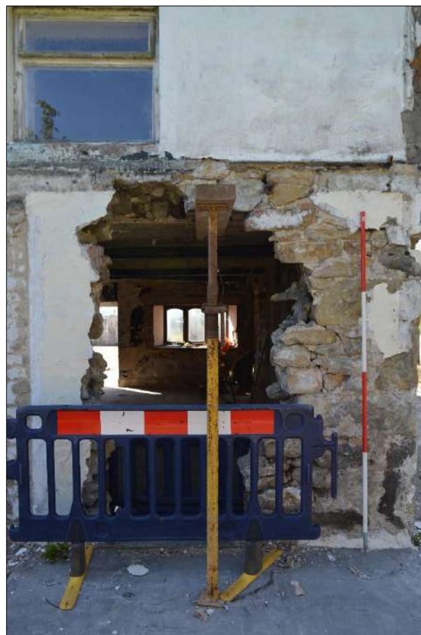
Plate 8 (shot 33): Damaged entrance in northwest elevation of farmhouse, looking southeast, 2m scale
