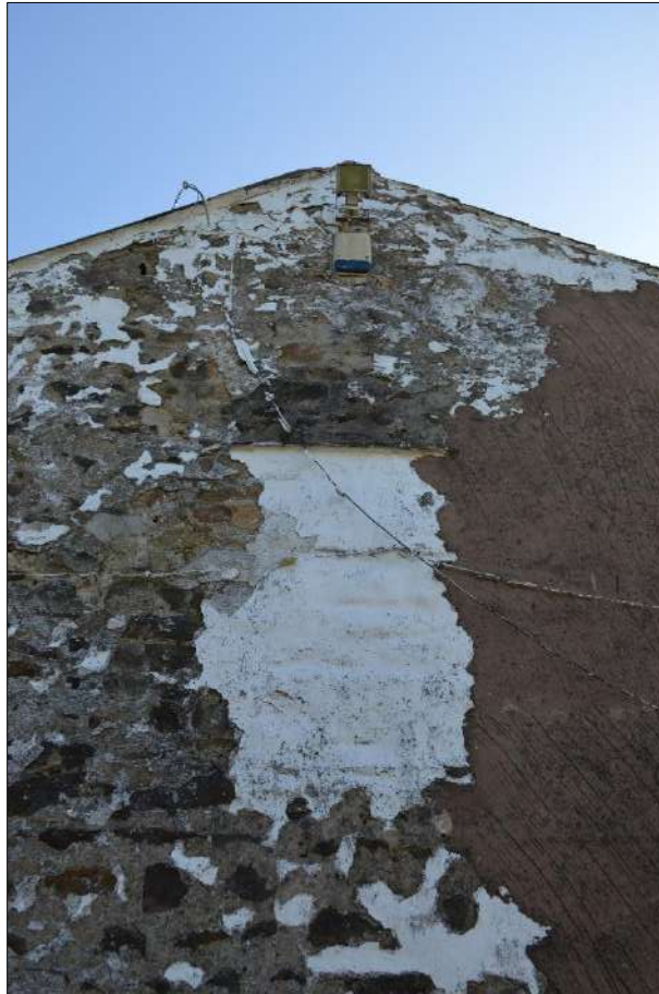
Plate 6 (shot 38): Blocked first floor window in southwest-facing elevation of farmhouse, looking northeast, no scale
