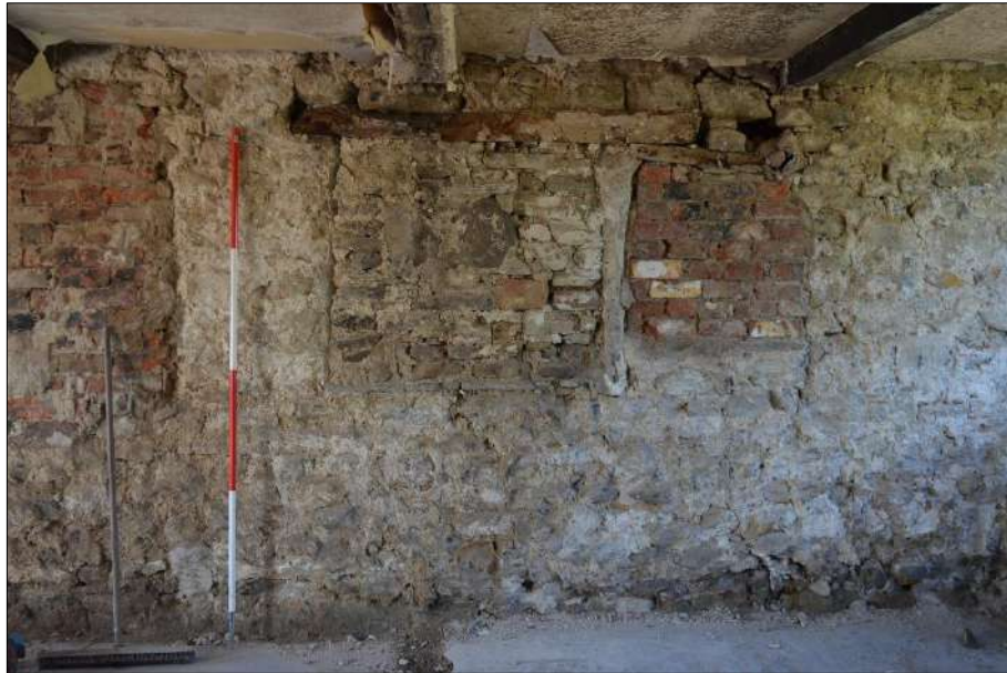
Plate 19 (shot 44): Detail of blocked windows in southwestern wall, Room 1, 2m scale
