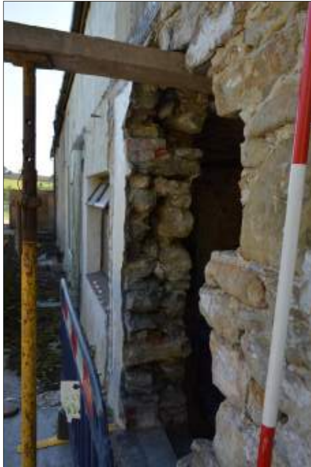
Plate 9 (shot 35): Damaged entrance in northwest elevation of farmhouse showing structure of masonry, 2m scale
