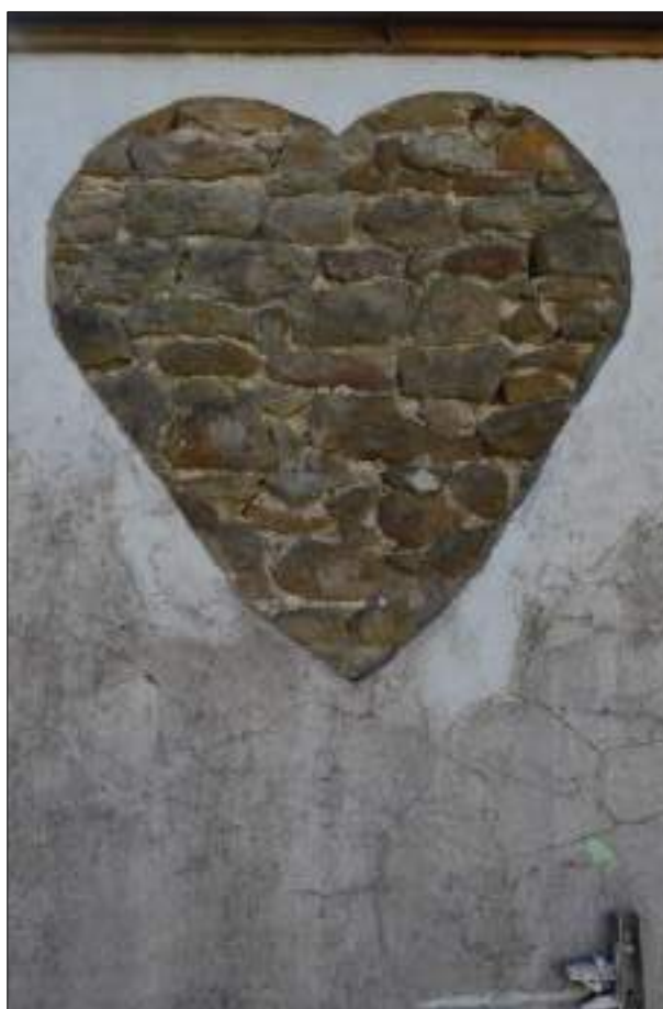
Plate 110 (shot 136): Heart shaped patch of exposed masonry in northwestern elevation of outbuilding, no scale
