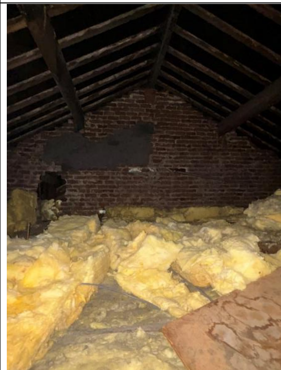
Photograph 7: View of the loft space in good condition. No light seen penetration through eaves or roof felt.
