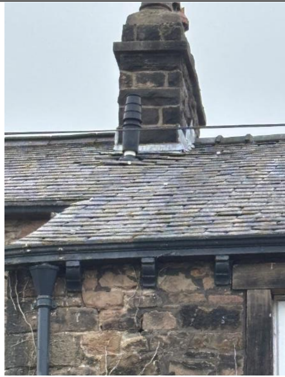
Photograph 6: View of the loose roof tiles around chimney on north facing elevation.
