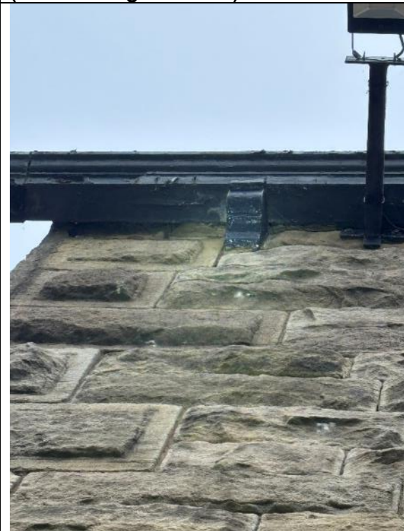
Photograph 3: View of the small gaps between fascia and wall plate on south facing elevation.
