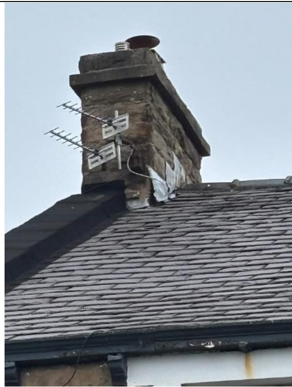
Photograph 2: View of the loose lead flashing around the chimney on south facing elevation.
