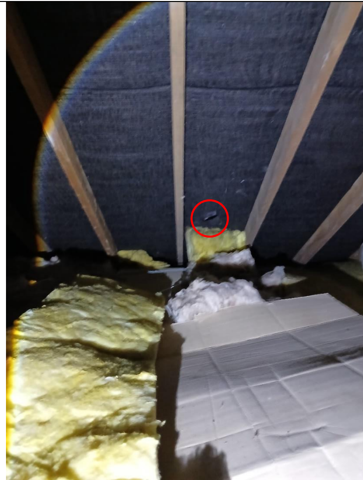
Slight tear in membrane to the east.
