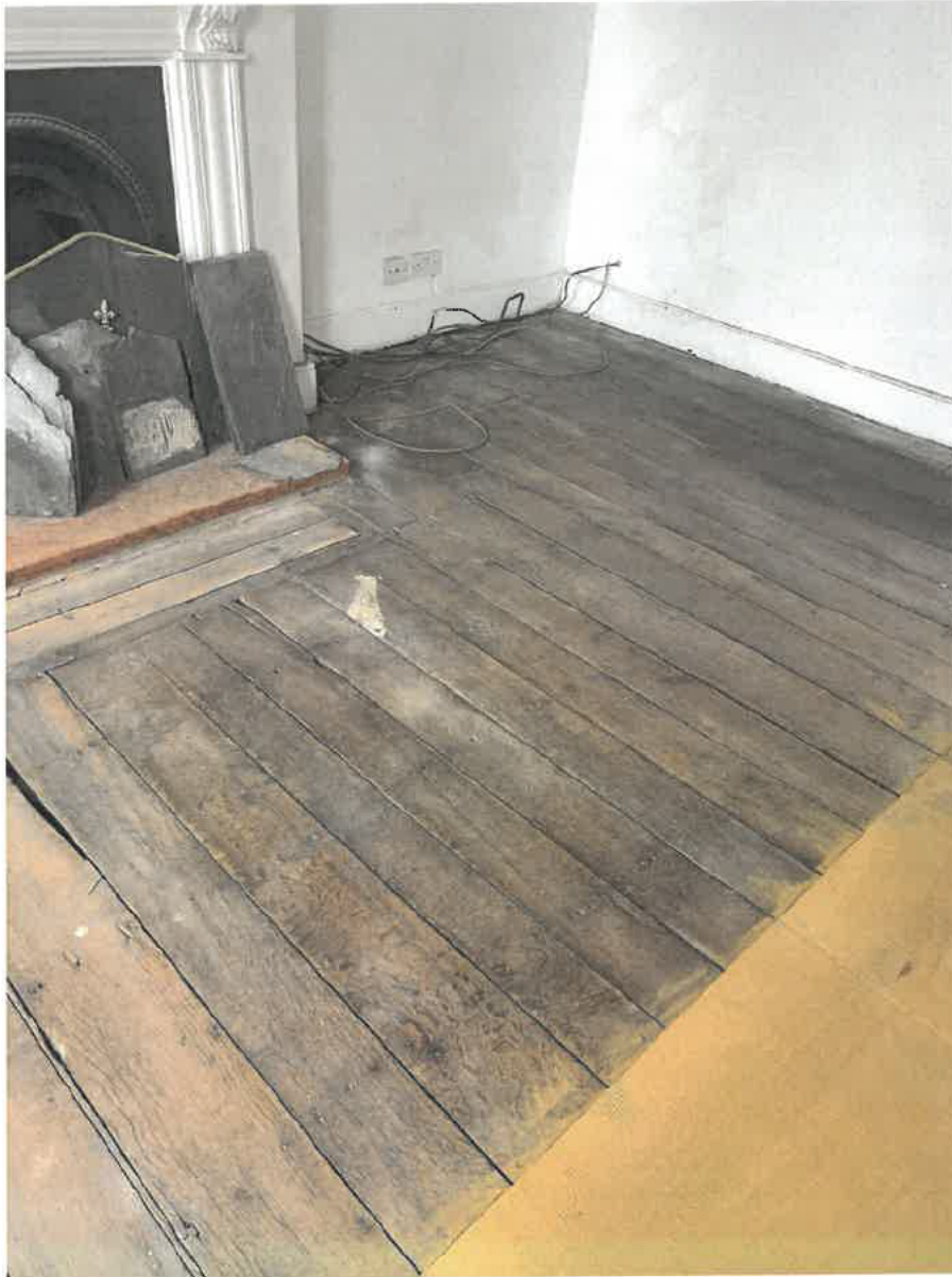
Observation: Additional view highlighting irregular board levels and settlement.
