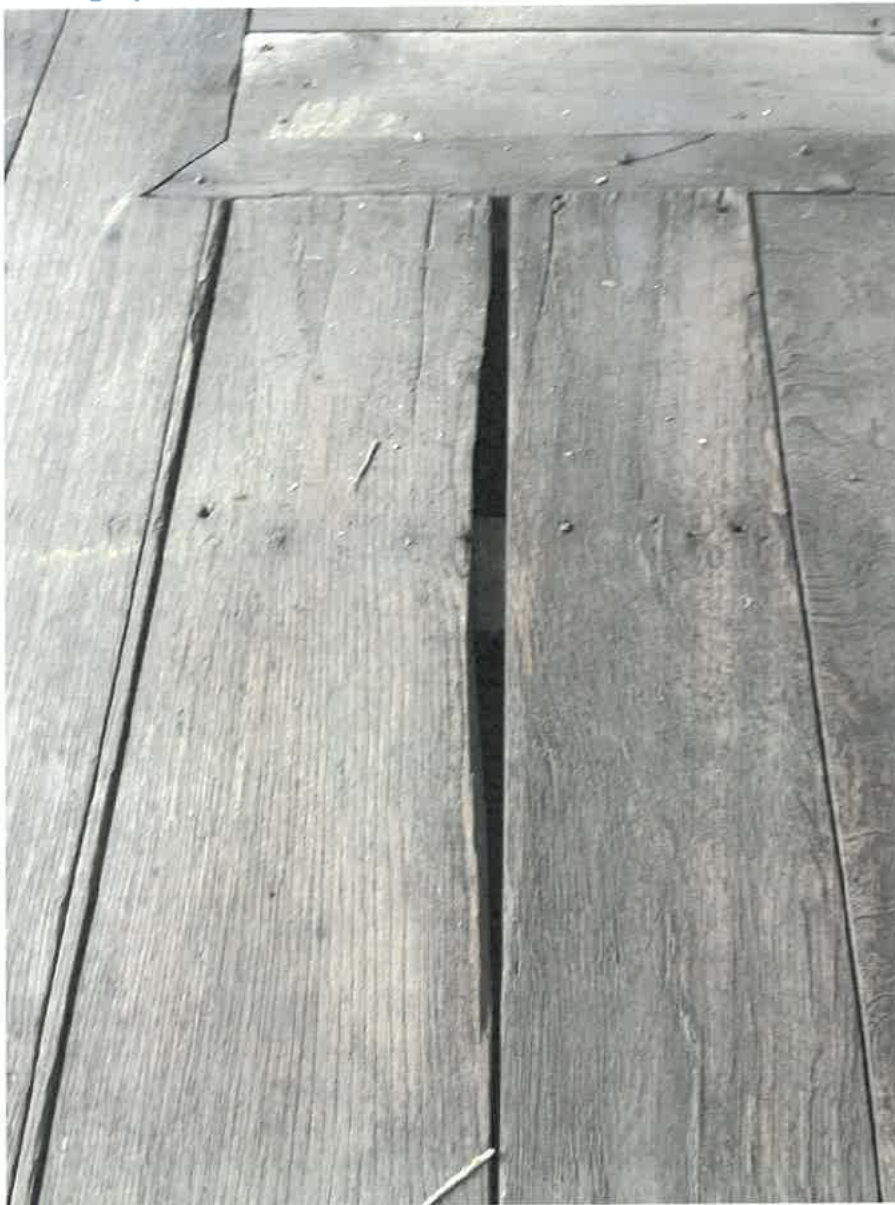
Photograph 4 – Excessive Gaps Between Boards
