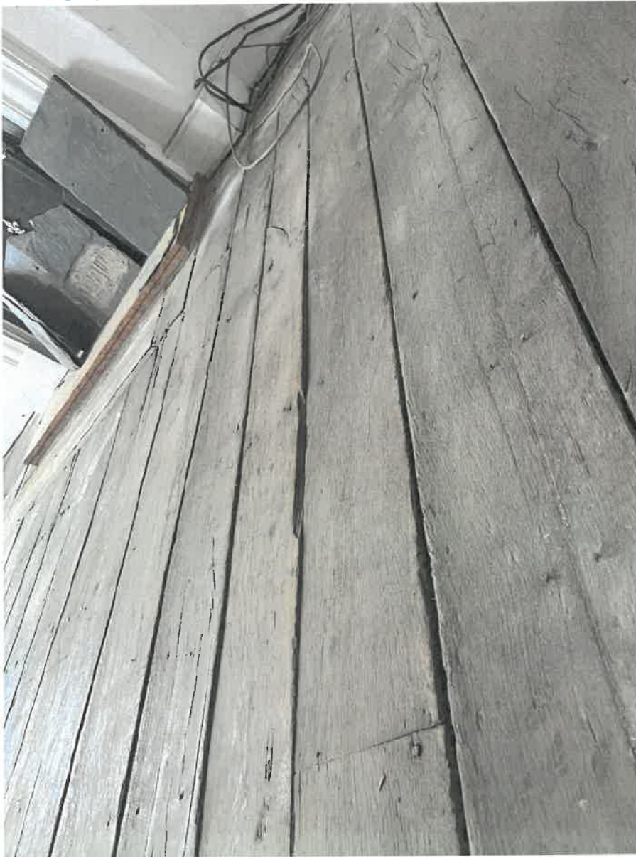
Photograph 2 – Evidence of Floor Deflection
