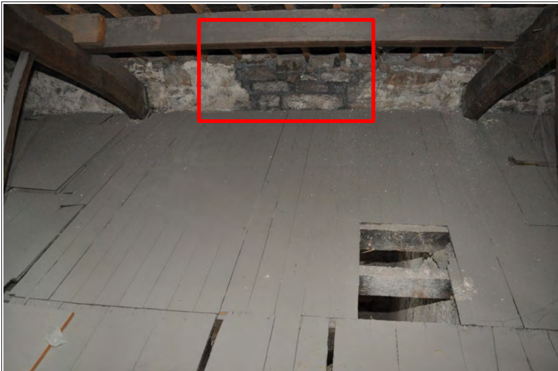
Photo 3: Window infill and position of former stair (to be reinstated) on second floor
