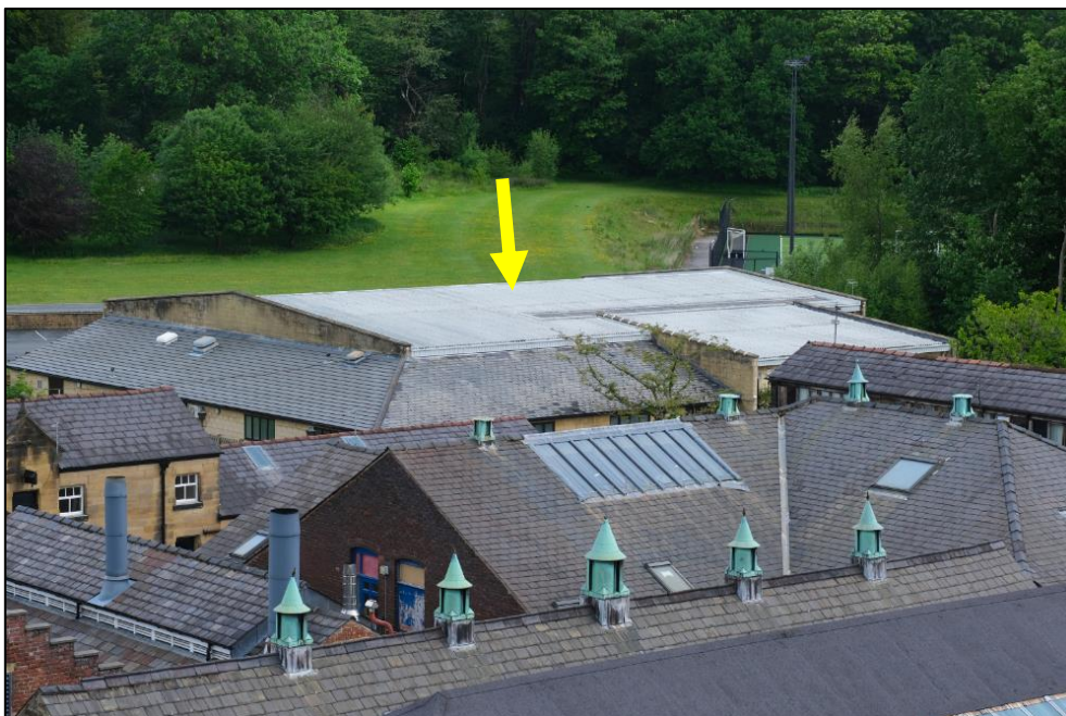
Image showing (external) roof covering of Building 2 (yellow arrow) and its context, with other buildings and vegetation in close proximity
