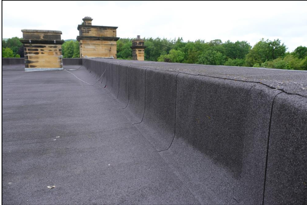
Image of roof top showing sealed liner and stone chimney stacks on Building 4
