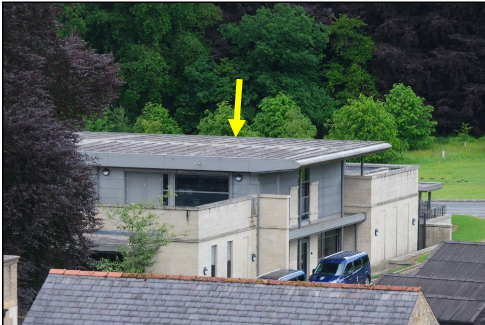
Image 1 – View of Building 1, New Refectory comprises a flat metal sheet roof on steel roof supports with lower-level, flat roof sections on the north and south elevations covered with a sealed membrane, May 2025.
