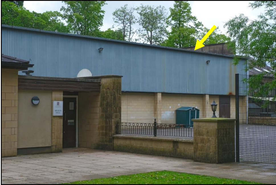
Image 3 – View of Building 3, St Marys Hall Sports Hall comprises a shallow pitched metal sheet roof on steel roof supports and roof lights, May 2025.
