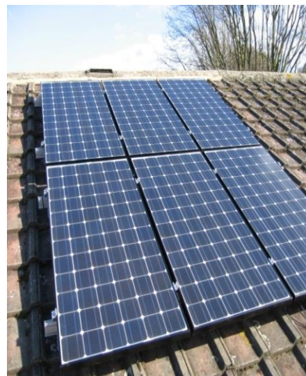
Figure 7 - Photovoltaic array on a pitched roof
