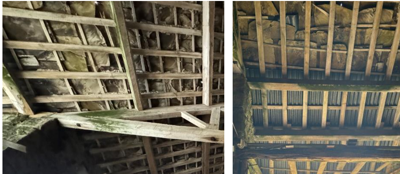
Figure 3 Weathered timber truss and beam in main entrance
