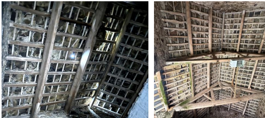
Figure 4 Light shining through roof in areas
