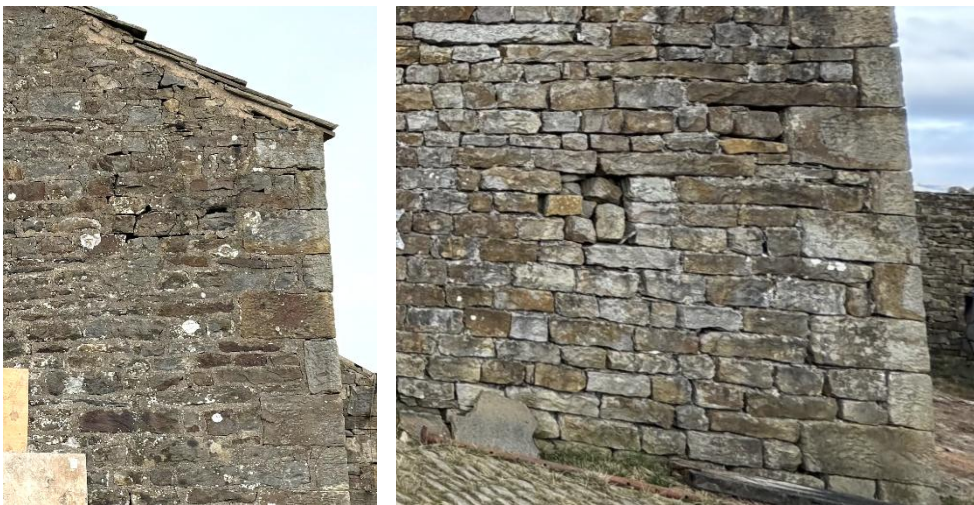
Figure 1 Missing mortar and loose stone externally
