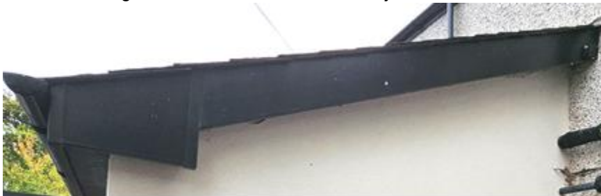
The main roof is a hipped blue slate structure. With a dormer formed in the hipped side of the roof.
