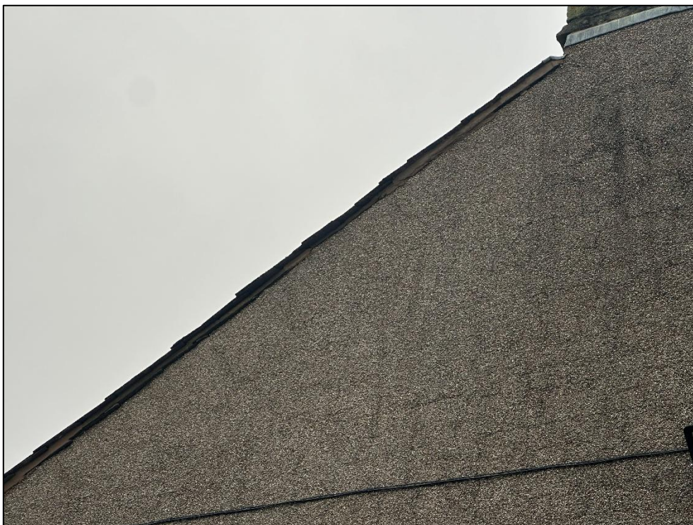
Plate 4: The water tabling will occur along the verge, so the roof edge and chimney and whether they offered any PRFs were the key area for inspection.
