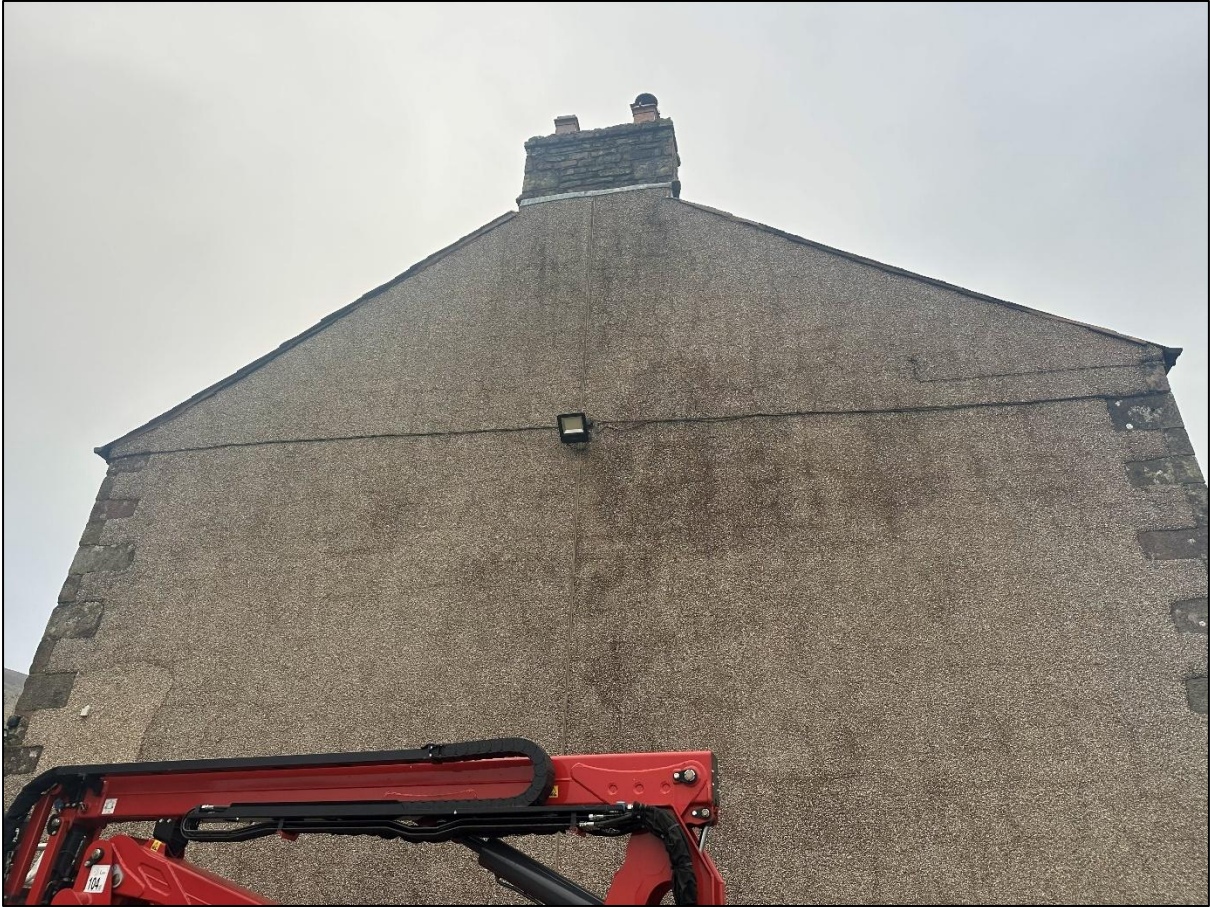
Plate 1: General view of the west-facing elevation of the property (with MEWP in foreground).
