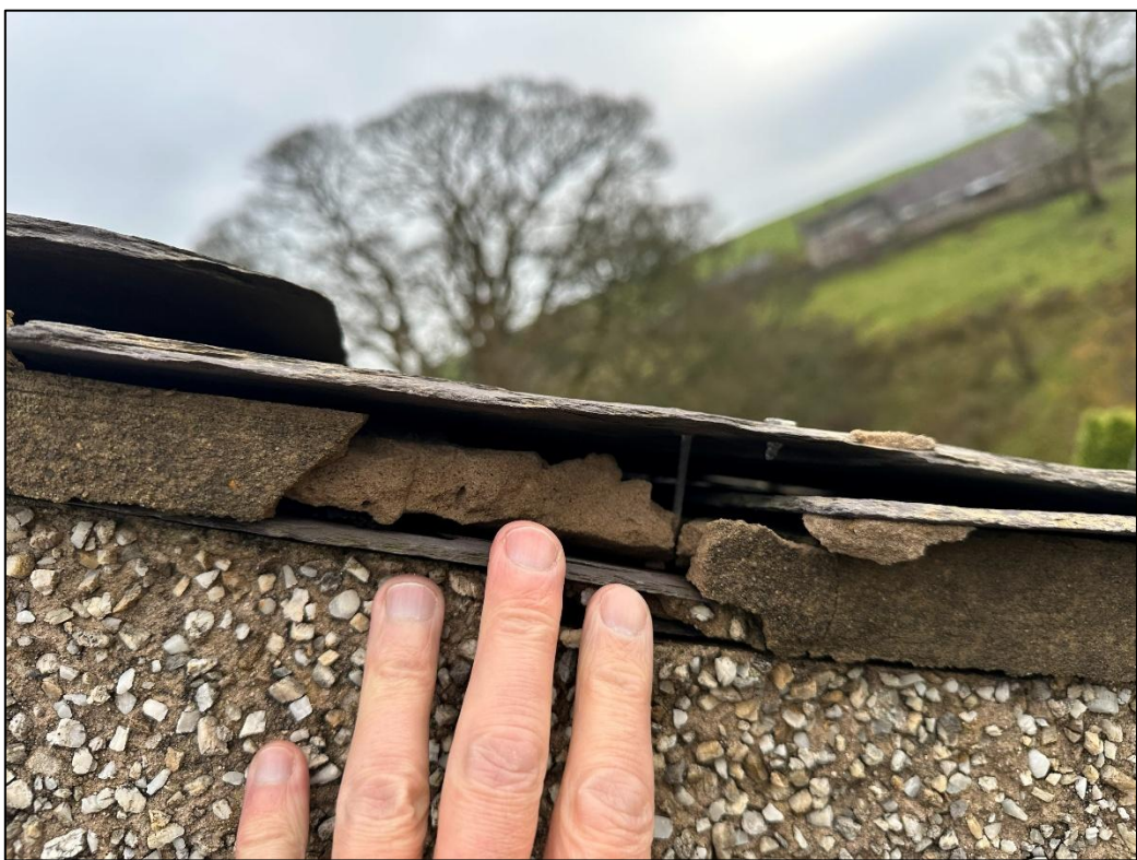
Plate 10: The larger gaps between the two layers of slate offered no access to the roof battens and the gap did not offer a suitable crevice for bat roosting.
