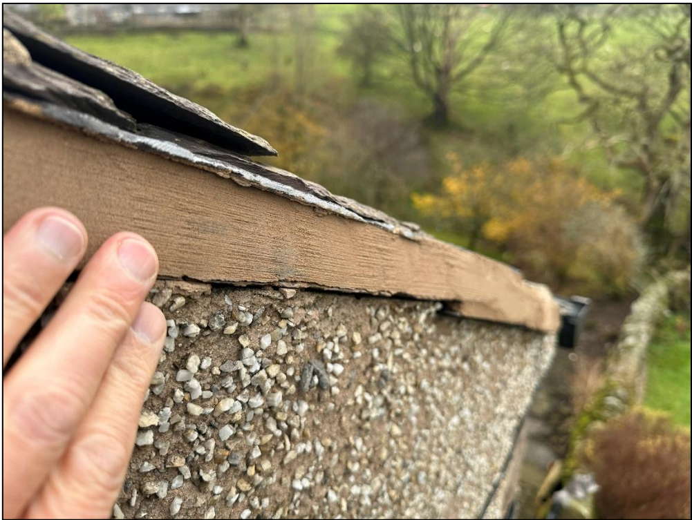
Plate 7: The close-up inspection found that the verges were generally well sealed, and large parts of the mortar offering nil roosting potential.
