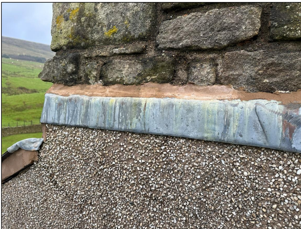
Plate 5: The survey started by inspecting the chimney. Lead flashings around the chimney were intact and offered no roosting potential.
