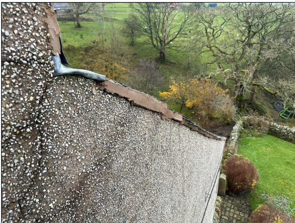
Plate 6: Once up at height in the MEWP, it was clear that the mortaring along the verges was patchy/inconsistent.
