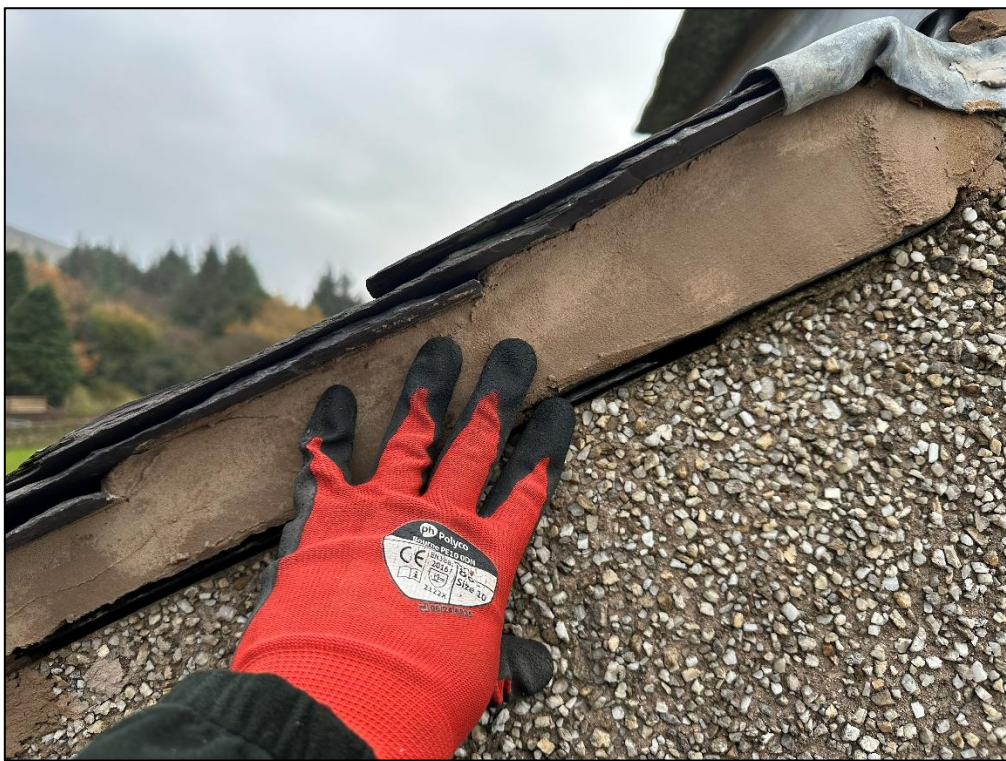
Plate 8: A thick bed of mortar was present between the pebbledash and the slates, and mostly had no roosting potential.
