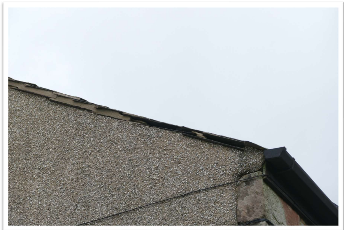
2. Poor verge detail
