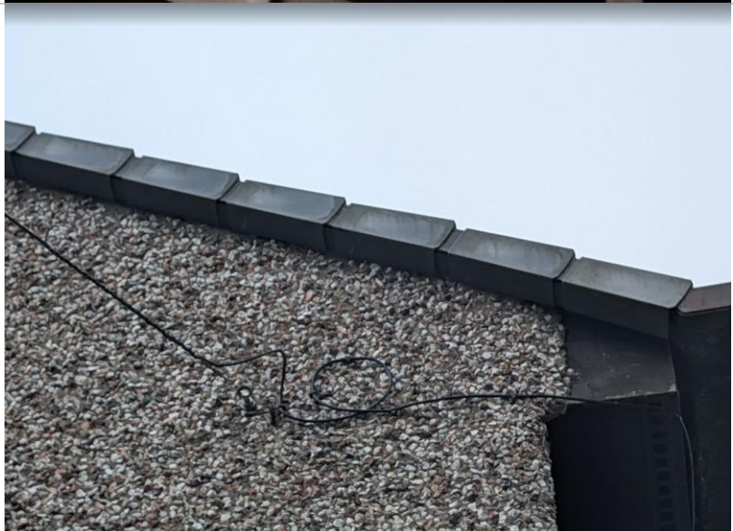
Photo 6. Example of slight gap under the roof verge on the gable.
