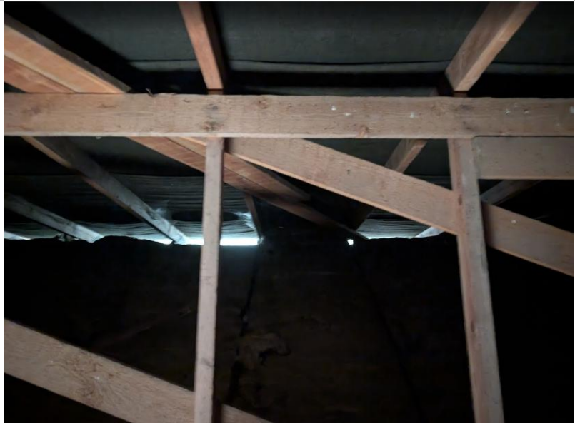
Photo 5. Light gap in loft from roof verge at frontage.
