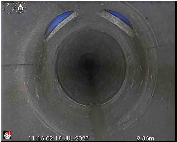
S16X_b406b9c5-5266-463f-8d7f-39144229c92f_20230719_084132_259.jpg, 00:00:42, 9.86 m Connection other than junction at 01 o'clock, 150mm dia
