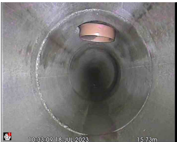
S15X_83803eba-5f3c-427b-a586-ab6f81f50a07_20230719_083737_463.jpg, 00:01:12, 15.73 m Connection defective, connecting pipe is intruding at 12 o'clock, 150mm dia, intrusion: 10%
