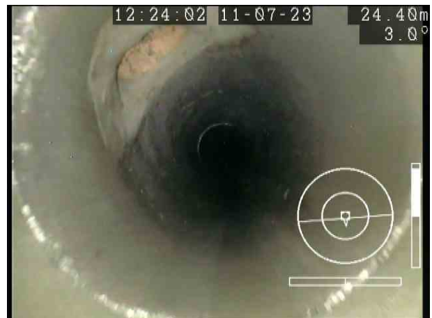
S3X_c6c7fd8f-4725-4563-99ff-85b4c7b35617_20230717_123310_143.jpg, 00:01:22, 24.40 m Connection other than junction at 10 o'clock, 150mm dia
