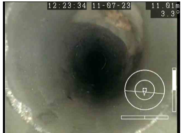
S3X_98c9a4b4-a209-4956-9b42-1767c74ca4a3_20230717_123240_424.jpg, 00:00:55, 11.00 m Connection other than junction at 01 o'clock, 150mm dia
