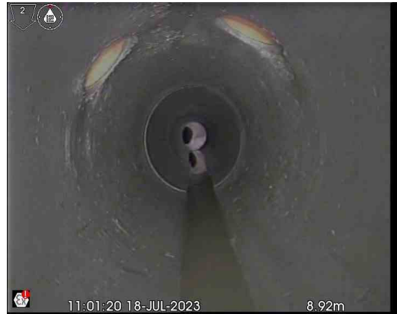
S6X_551f594b-43de-430f-9638-d64102814dd4_20230719_084042_289.jpg, 00:00:38, 8.92 m Connection other than junction at 10 o'clock, 150mm dia
