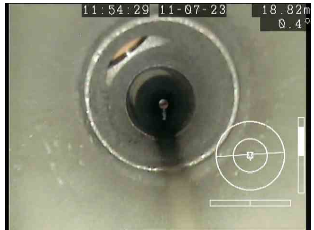
S2X_8f0c81a6-8968-4cf2-b07d-1b411f1828a0_20230717_12 2925_635.jpg, 00:00:58, 18.82 m Connection other than junction at 11 o'clock, 150mm dia
