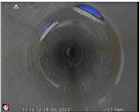
S16X_b6dadf70-05bf-4ba6-aeb6-a05bbb3c8f39_20230719_084200_104.jpg, 00:01:33, 25.96 m Connection other than junction at 01 o'clock, 150mm dia
