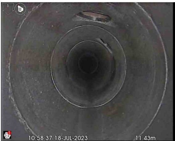
S5X_464e9282-bcda-4122-a6a9-0c10dc12b58a_20230719_083904_800.jpg, 00:00:49, 11.43 m Connection other than junction at 01 o'clock, 150mm dia
