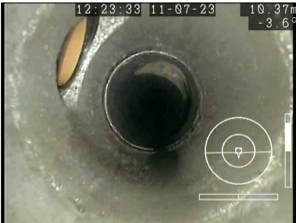
S3X_816e11e9-31f4-4a41-8603-53dc22ac2779_20230717_123231_169.jpg, 00:00:53, 10.37 m Connection other than junction at 10 o'clock, 150mm dia
