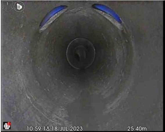
S5X_aa5db9e7-ef72-4a2f-8741-cb38c19b37ec_20230719_083947_037.jpg, 00:01:31, 25.40 m Connection other than junction at 01 o'clock, 150mm dia
