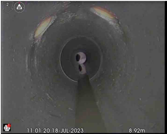
S6X_f8838de4-89cb-4f05-95ca-006372961c53_20230719_084033_836.jpg, 00:00:38, 8.92 m Connection other than junction at 01 o'clock, 150mm dia
