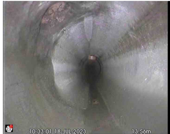
S15X_b453d0a2-4c1b-432a-ad0f-cc587732be68_20230719_083720_022.jpg, 00:01:03, 13.56 m Connection other than junction at 11 o'clock, 150mm dia
