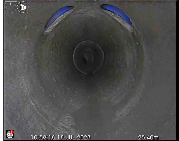
S5X_97b800b8-6e34-46ba-a3b3-74080f5063b7_20230719_083955_518.jpg, 00:01:31, 25.40 m Connection other than junction at 11 o'clock, 150mm dia
