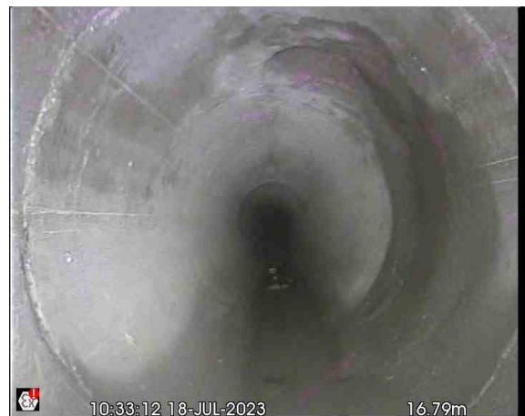
S15X_3a217687-8e4a-422f-986b-ab51f2207361_20230719_083801_945.jpg, 00:01:15, 16.79 m Connection other than junction at 01 o'clock, 150mm dia
