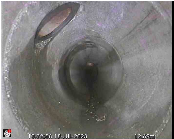
S15X_3e7e19de-77be-4fa0-ac92-c44a97039f94_20230719_083708_111.jpg, 00:01:01, 12.69 m Connection other than junction at 10 o'clock, 150mm dia
