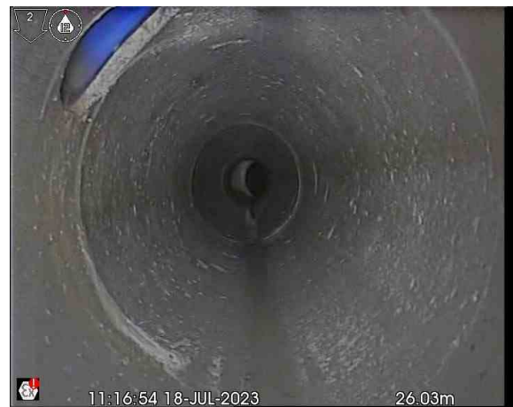
S16X_f207fe33-9c05-4af9-95d4-4b80a2fbc68d_20230719_084225_257.jpg, 00:01:34, 26.03 m Connection other than junction at 11 o'clock, 150mm dia
