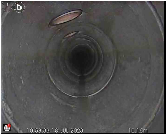
S5X_69482780-32c4-47c2-a862-55adb0e7964c_20230719_083845_973.jpg, 00:00:45, 10.16 m Connection other than junction at 11 o'clock, 150mm dia
