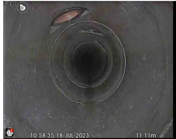
S5X_933ea363-1bea-4514-a186-d870029a2deb_20230719_083855_801.jpg, 00:00:46, 11.11 m Connection other than junction at 11 o'clock, 150mm dia
