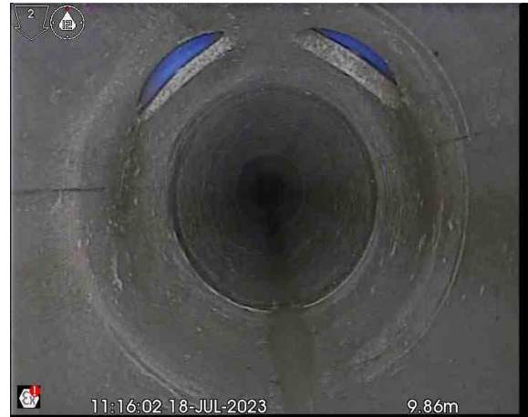
S16X_c7a32aba-50f1-48eb-b9cd-40a971cfac98_20230719_084141_165.jpg, 00:00:42, 9.86 m Connection other than junction at 11 o'clock, 150mm dia
