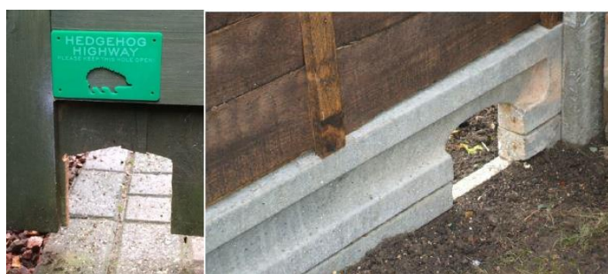
Insert 4: Showing wildlife access gap within fencing
