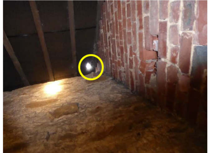
Hole in roof alongside chimney breast.
