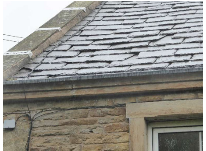
SE front elevation showing multiple gaps under slates at western end.
