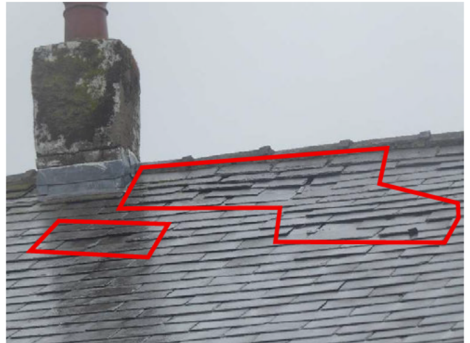
Rear NW elevation showing slate gaps.
