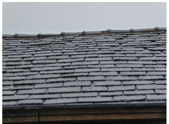
SE front elevation showing multiple gaps under slates in the middle roof section
