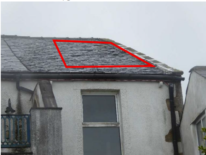
Rear NW elevation showing slate gaps.
