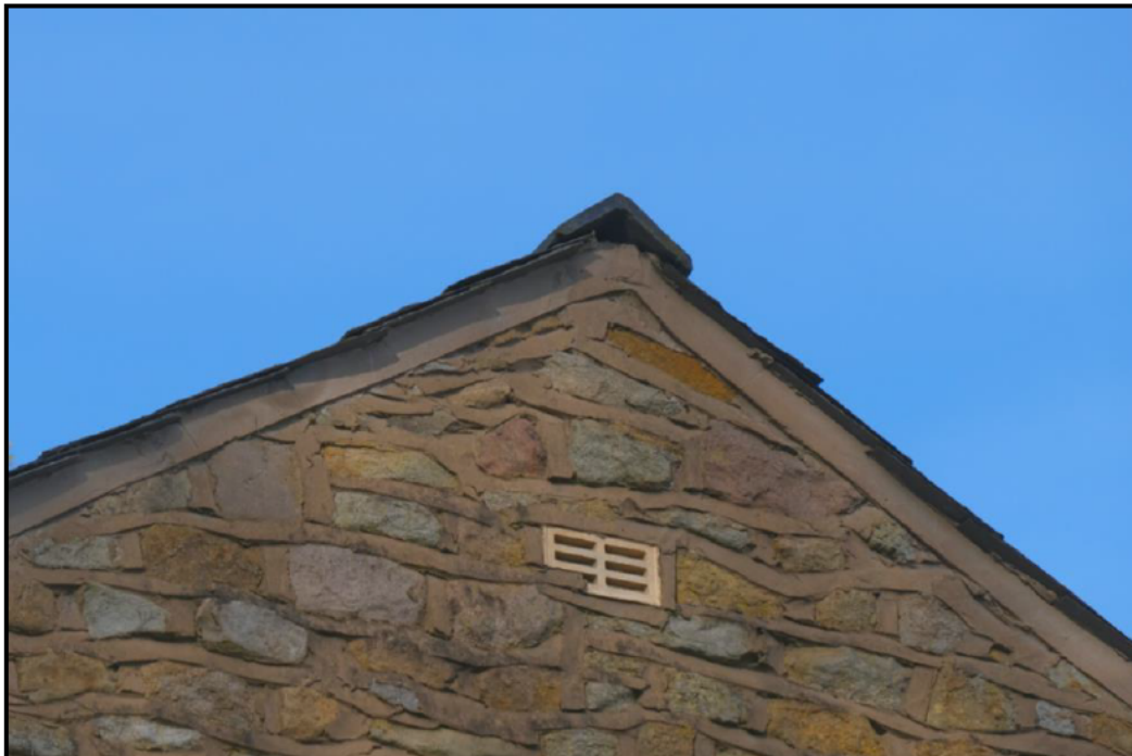
Image of east gable, verge is mortared and sealed but single gap present at the apex
