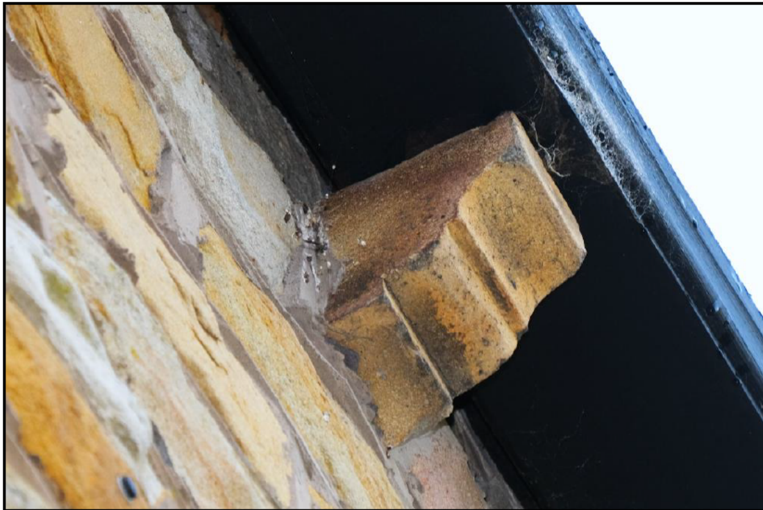
Image showing bird droppings below wall top gap north elevation. Wall top gaps have potential for use by bats.
