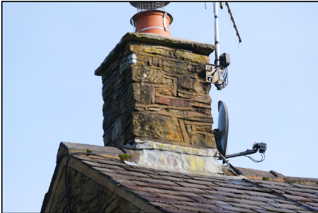
Image of west gable showing chimney, ridge and roof coverings. Roof verge and apex sealed but suitable gaps are present in roof coverings and along adjacent ridge
