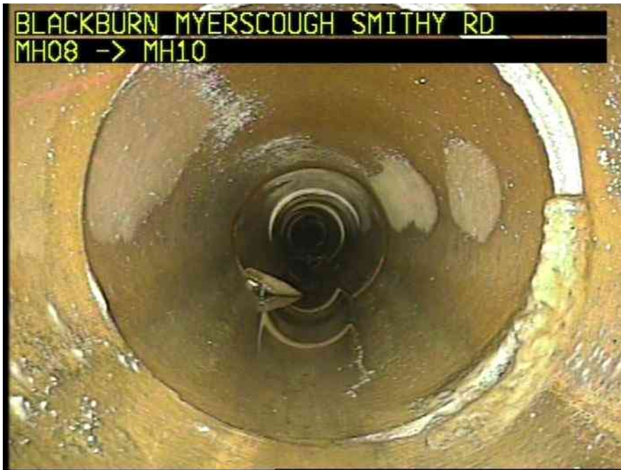
MH08X_D_14082025_1244_078.jpg, 00:03:33, 14.43 m Attached deposits, encrustation from 3 o'clock to 5 o'clock, 5% cross-sectional area loss
