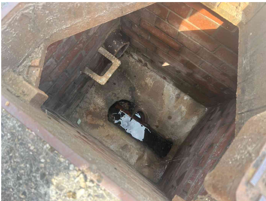
MH04X_D_13082025_1054_032.jpg, 00:01:33, 14.17 m Finish node, manhole, reference: MH05, MANHOLE LOCATED ADJACENT TO FIRE EXIT
