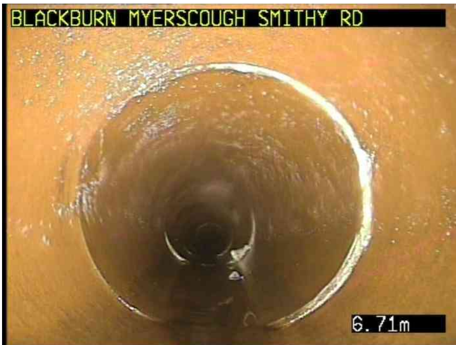
MH04X_D_13082025_1054_028.jpg, 00:00:46, 6.69 m Crack, circumferential at joint from 9 o'clock to 10 o'clock
