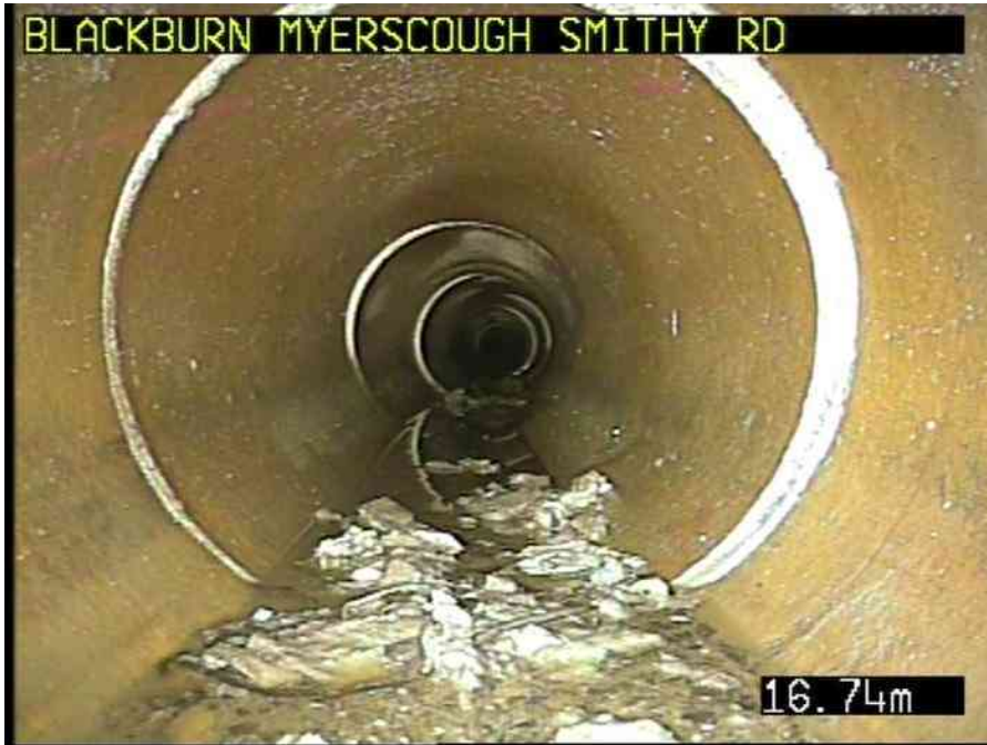
MH08X_D_14082025_1244_080.jpg, 00:04:27, 16.74 m Settled deposits, coarse, 5% cross-sectional area loss
