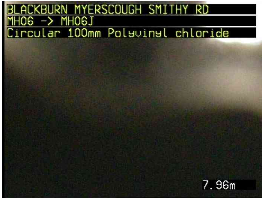
MH06X_D_13082025_1145_037.jpg, 00:00:56, 7.91 m Settled deposits, fine, 60% cross-sectional area loss, finish
