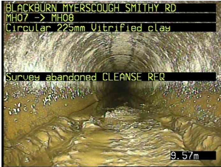
MH07X_D_14082025_1308_062.jpg, 00:01:37, 9.57 m Survey abandoned, CLEANSE REQ
