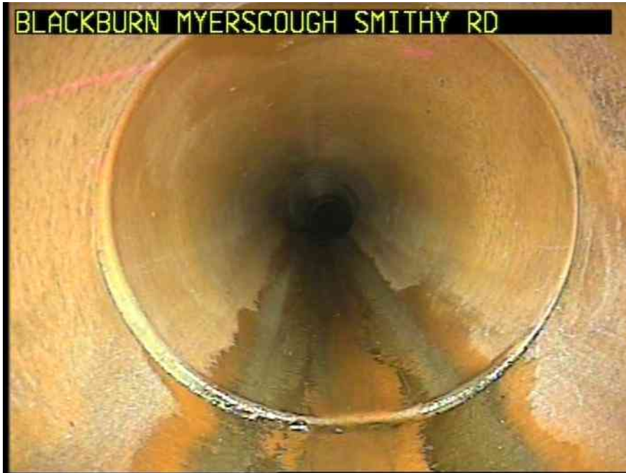
MH08AX_U_14082025_1232_065.jpg, 00:00:36, 6.28 m Crack, longitudinal at joint at 3 o'clock
