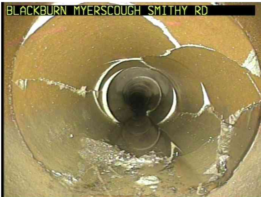
MH08X_D_14082025_1244_083.jpg, 00:06:41, 36.62 m Broken pipe from 12 o'clock to 12 o'clock
