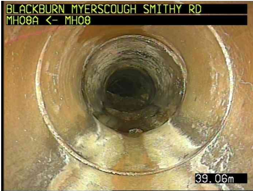
MH08AX_U_14082025_1232_069.jpg, 00:04:59, 39.06 m Crack, longitudinal at joint at 3 o'clock
