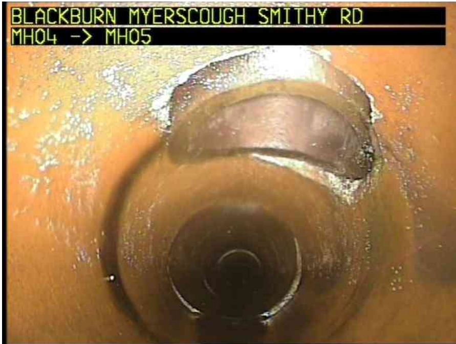
MH04X_D_13082025_1054_029.jpg, 00:00:54, 7.63 m Connection defective, connecting pipe is intruding at 12 o'clock, 100mm dia, intrusion: 5%
