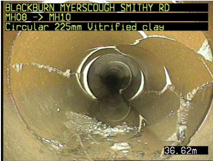
MH08X_D_14082025_1244_084.jpg, 00:06:45, 36.62 m Deformed sewer or drain, 10%
