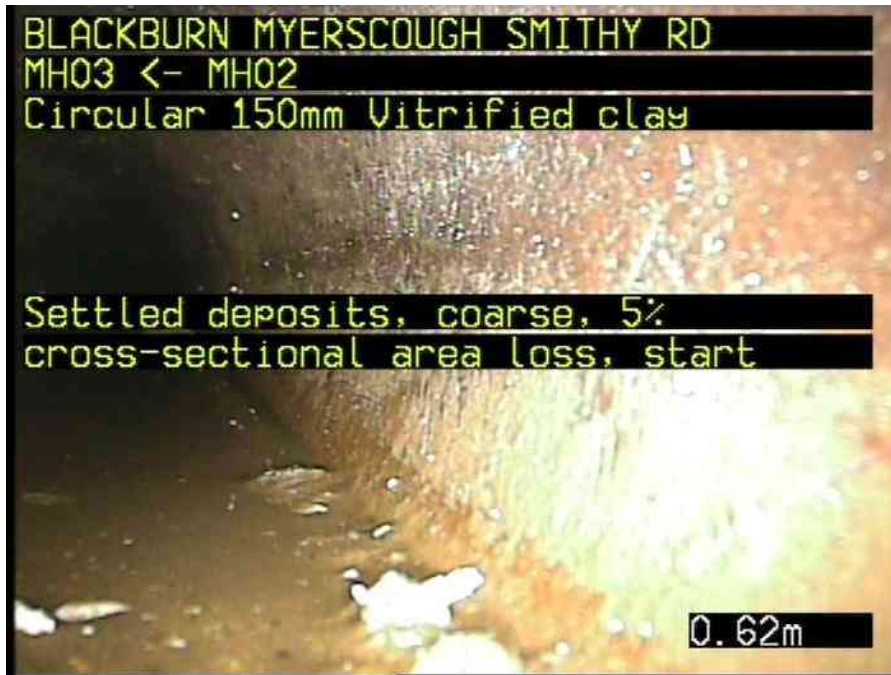
MH03X_U_13082025_1034_015.jpg, 00:00:19, 0.62 m Settled deposits, fine, 10% cross-sectional area loss, start
