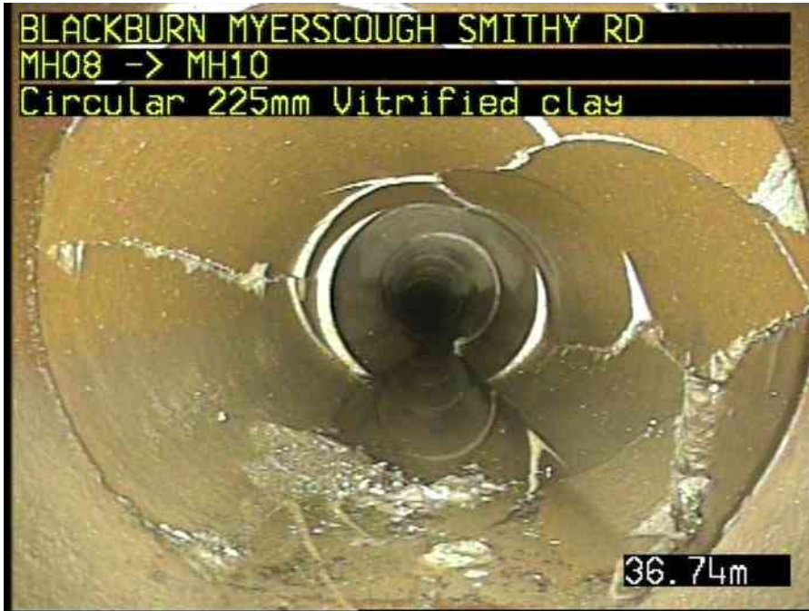
MH08X_D_14082025_1244_086.jpg, 00:06:57, 36.75 m Survey abandoned, UNABLE TO PROCEED WITH SURVEY DUE RISK OF EQUIPMENT OVER BROKEN PIPE
