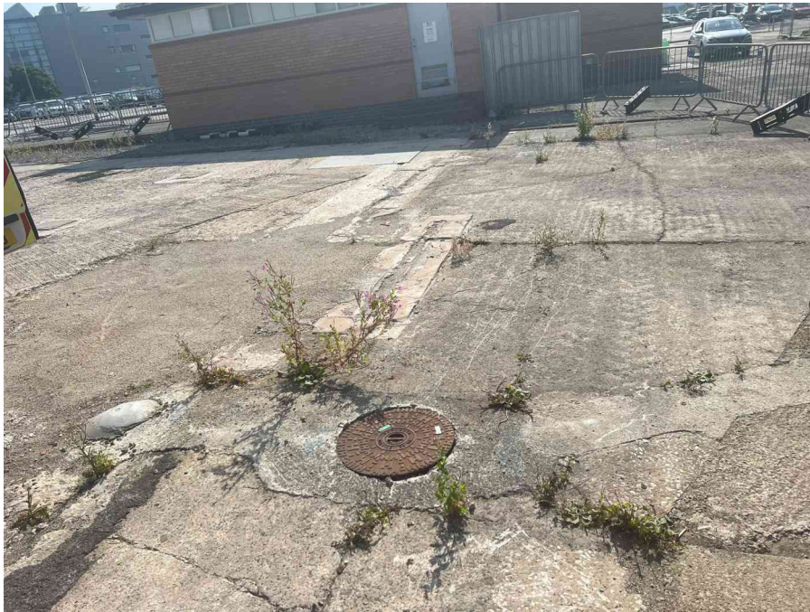
MH01X_D_13082025_0951_001.jpg, 00:00:00, 0.00 m Start node, inspection chamber, reference: MH01, IC LOCATED ADJACENT TO STAIRCASE
