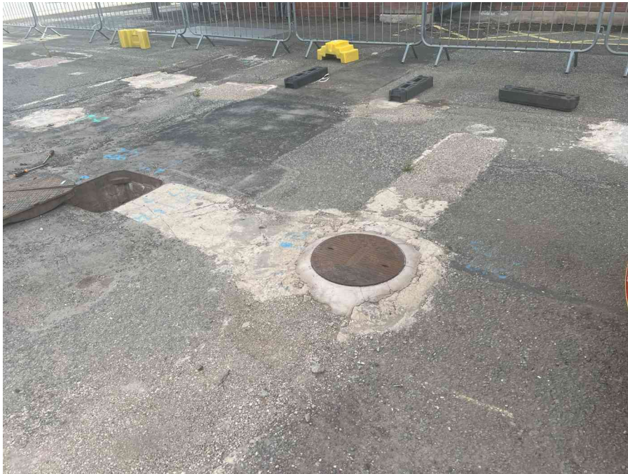
MH09X_D_14082025_1220_048.jpg, 00:00:00, 0.00 m Start node, inspection chamber, reference: MH09, IC LOCATED ADJACENT TO BAY DOORS
