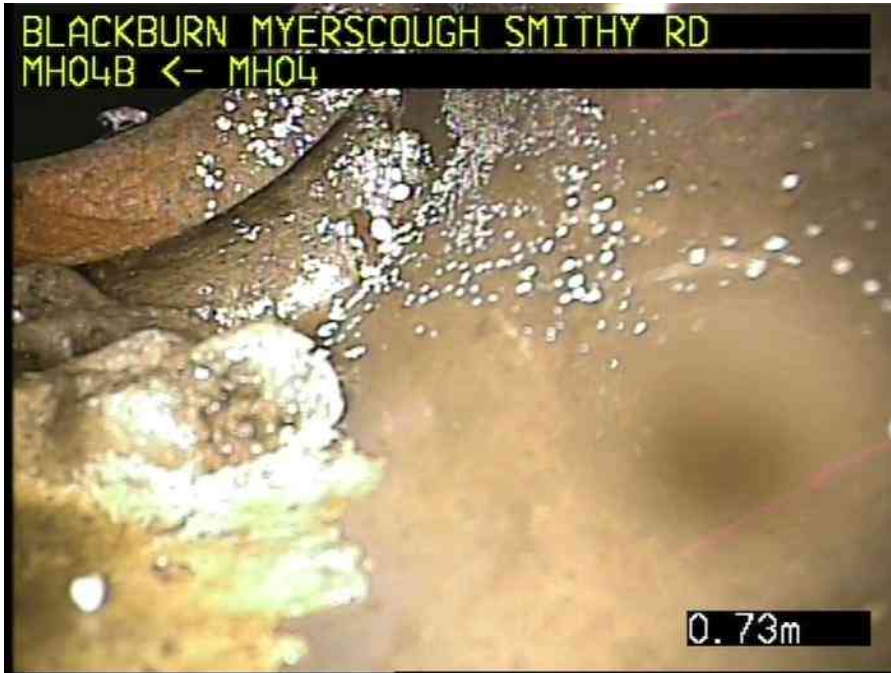
MH04BX_U_13082025_1225_047.jpg, 00:00:08, 0.60 m Joint displaced, large
