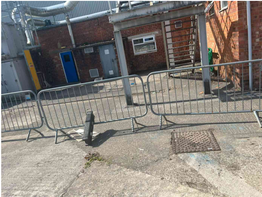
MH02AX_U_13082025_1026_011.jpg, 00:00:00, 0.00 m Start node, manhole, reference: MH02, MANHOLE LOCATED ADJACENT TO STAIR CASE
