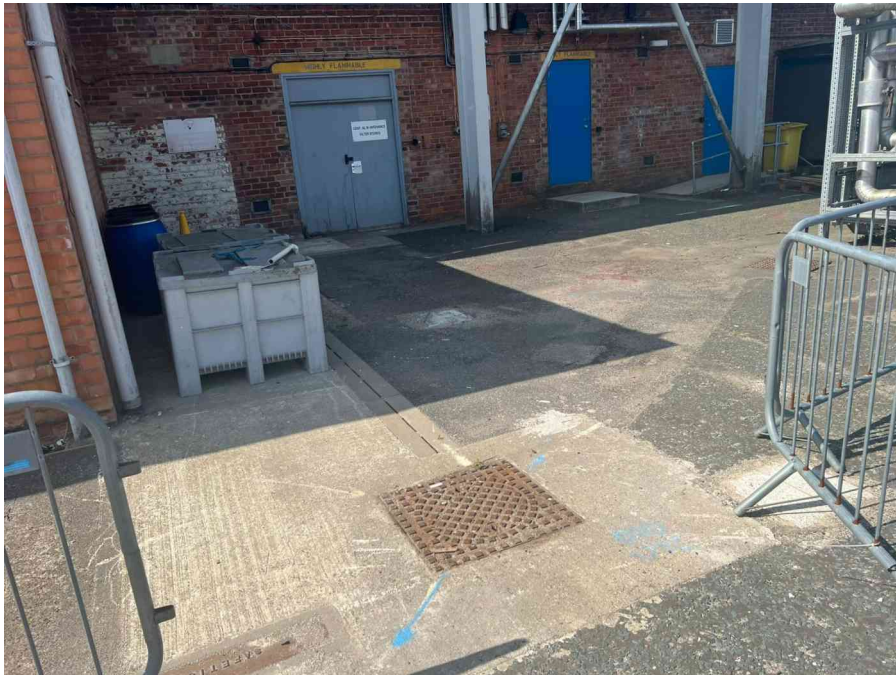
MH03X_U_13082025_1034_019.jpg, 00:01:47, 13.00 m Finish node, manhole, reference: MH03, MANHOLE LOCATED ADJACENT TO COOLING UNIT UTR
