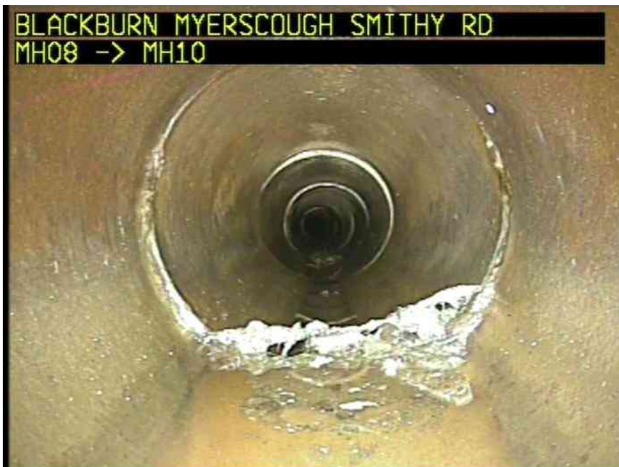
MH08X_D_14082025_1244_081.jpg, 00:06:03, 32.31 m Attached deposits, encrustation from 4 o'clock to 8 o'clock, 5% cross-sectional area loss
