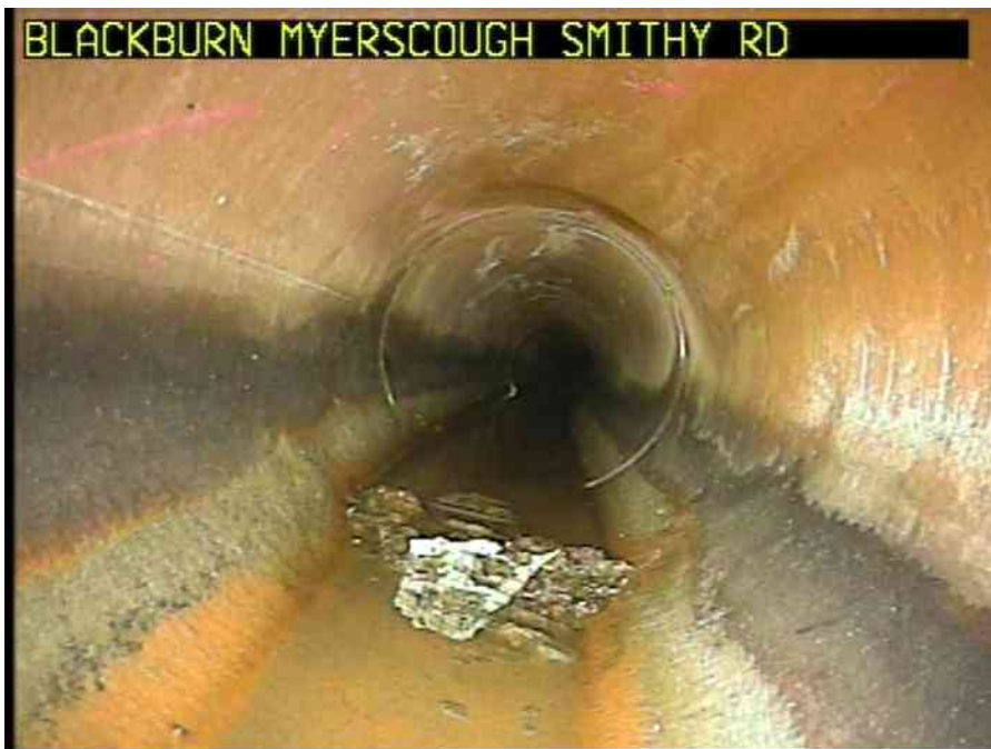
MH08AX_U_14082025_1232_066.jpg, 00:01:06, 11.17 m Settled deposits, coarse, 5% cross-sectional area loss
