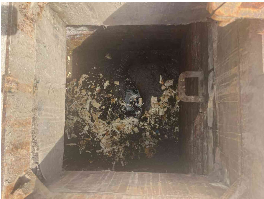
MH07X_D_14082025_1308_059.jpg, 00:00:00, 0.00 m Start node, manhole, reference: MH07, MANHOLE LOCATED ADJACENT TO COOLING STATION
