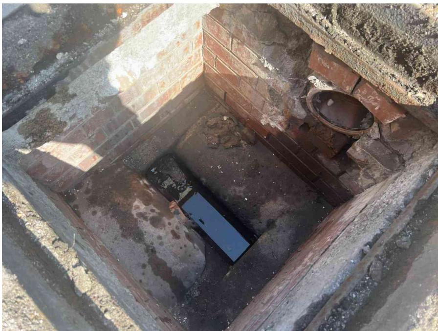
MH02AX_U_13082025_1026_012.jpg, 00:00:00, 0.00 m Start node, manhole, reference: MH02, MANHOLE LOCATED ADJACENT TO STAIR CASE
