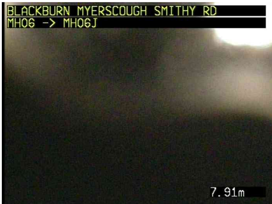
MH06X_D_13082025_1145_038.jpg, 00:00:57, 7.91 m Survey abandoned, CLEANSE REQ
