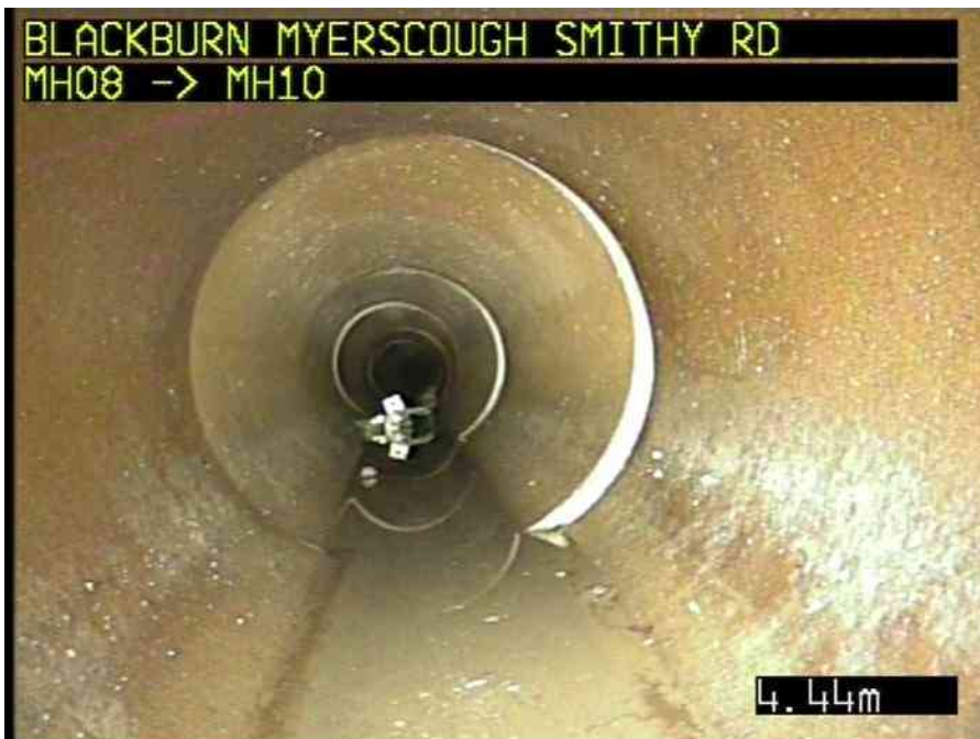
MH08X_D_14082025_1244_075.jpg, 00:00:53, 4.44 m Settled deposits, fine, 5% cross-sectional area loss, start
