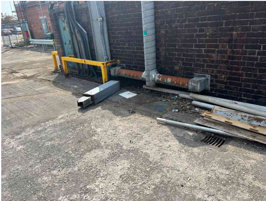
MH04BX_U_13082025_1225_045.jpg, 00:00:00, 0.00 m Start node, manhole, reference: MH04, MANHOLE LOCATED ADJACENT TO DUCTING
