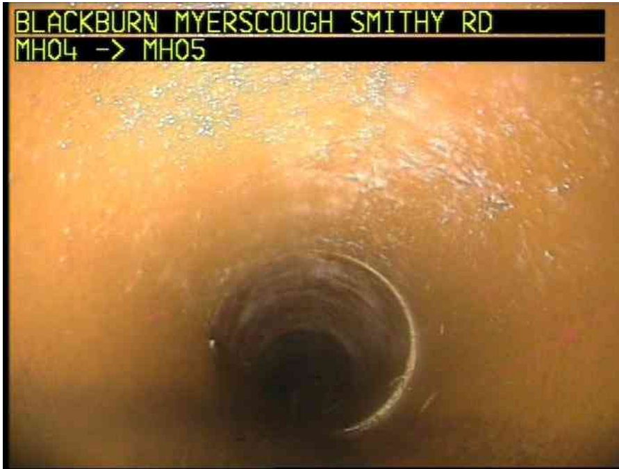
MH04X_D_13082025_1054_027.jpg, 00:00:29, 5.11 m Settled deposits, coarse, 5% cross-sectional area loss
