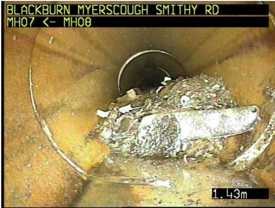
MH07X_U_14082025_1229_057.jpg, 00:00:25, 1.43 m Settled deposits, coarse, 50% cross-sectional area loss, CLEANSE REQ
