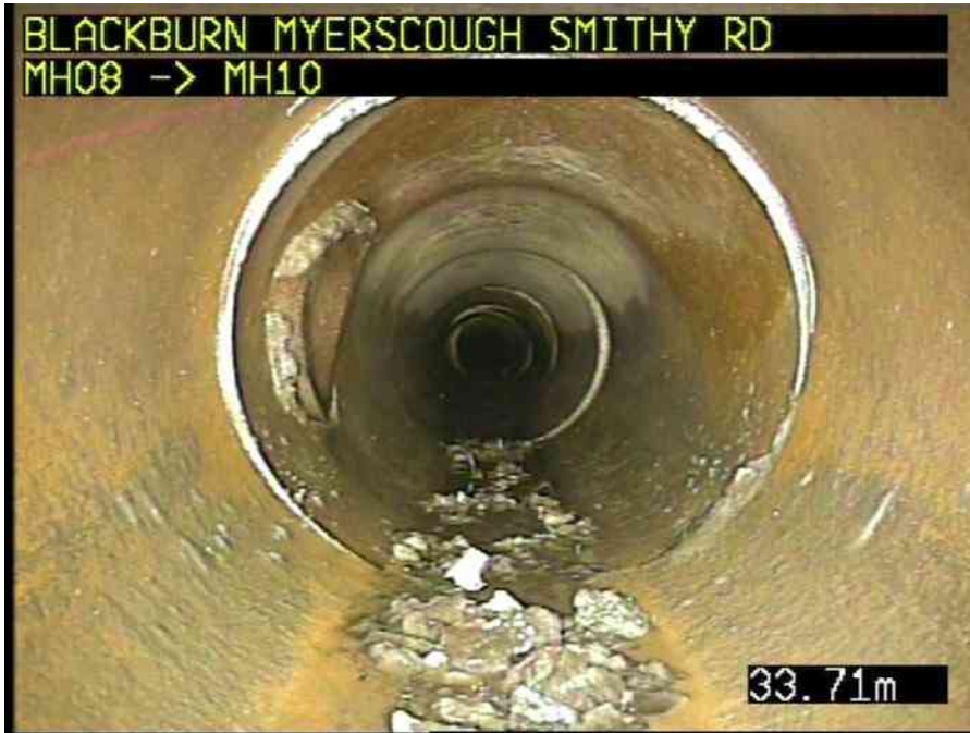
MH08X_D_14082025_1244_082.jpg, 00:06:15, 33.71 m Settled deposits, coarse, 5% cross-sectional area loss
