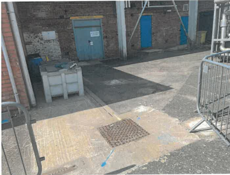
MH03X_U_13082025_1034_019.jpg, 00:01:47, 13.00 m Finish node, manhole, reference: MH03, MANHOLE LOCATED ADJACENT TO COOLING UNIT UTR
