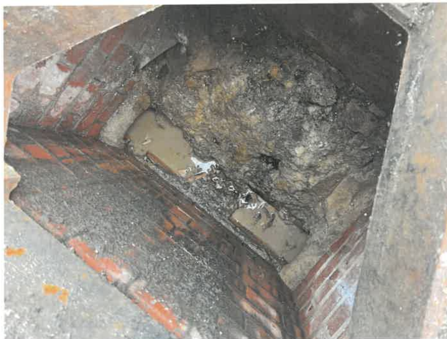
MH04X_D_13082025_1054_026.jpg, 00:00:00, 0.00 m Start node, manhole, reference: MH04, MANHOLE LOCATED ADJACENT TO DUCTING
