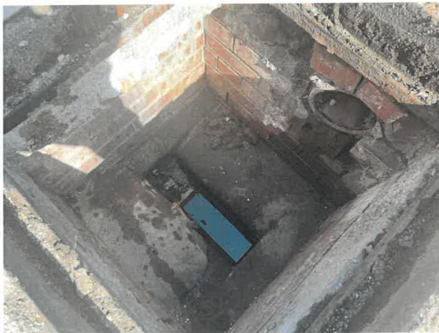
MH02X_D_13082025_1042_022.jpg, 00:00:00, 0.00 m Start node, manhole, reference: MH02, MANHOLE LOCATED ADJACENT TO STAIRCASE
