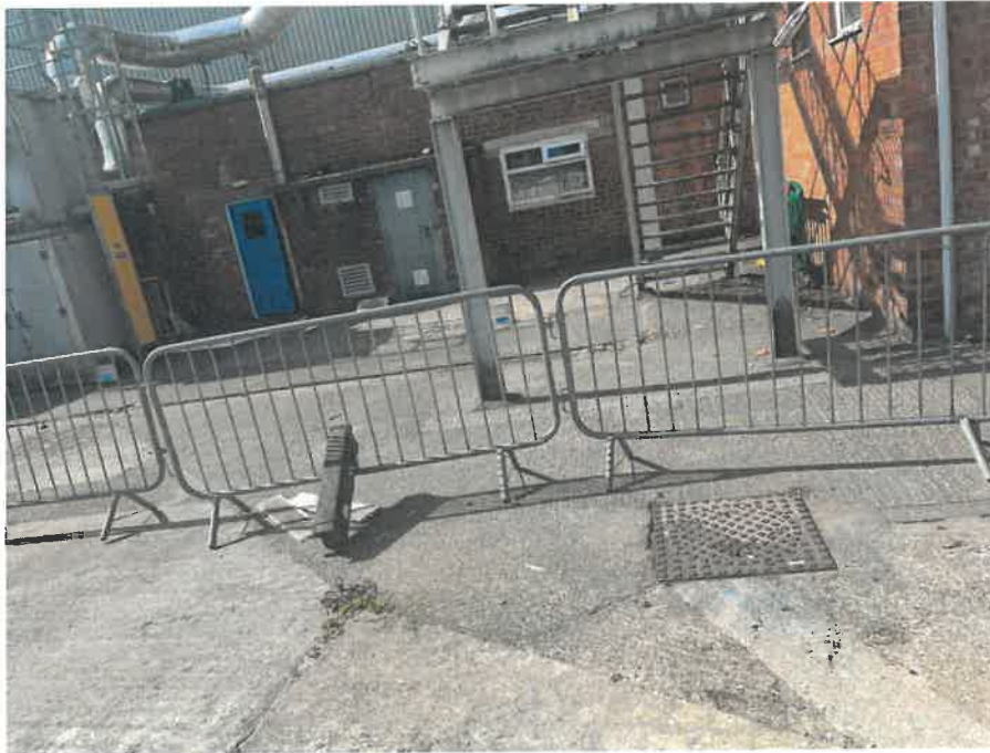
MH02X_D_13082025_1042_021.jpg, 00:00:00, 0.00 m Start node, manhole, reference: MH02, MANHOLE LOCATED ADJACENT TO STAIRCASE
