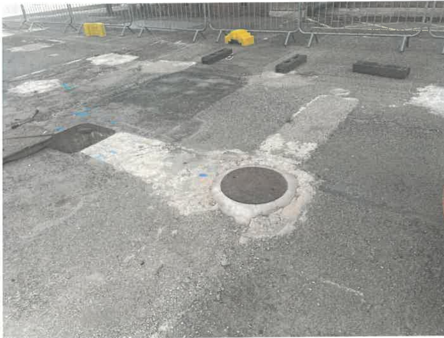
MH09X_D_14082025_1220_048.jpg, 00:00:00, 0.00 m Start node, inspection chamber, reference: MH09, IC LOCATED ADJACENT TO BAY DOORS
