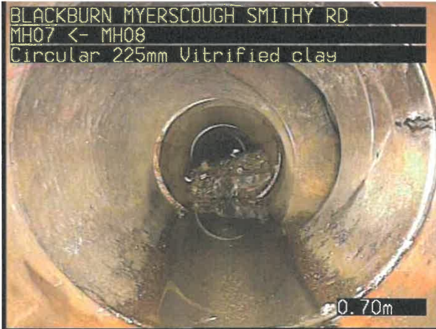
MH07X_U_14082025_1229_055.jpg, 00:00:11, 0.70 m Fracture, circumferential from 1 o'clock to 4 o'clock
