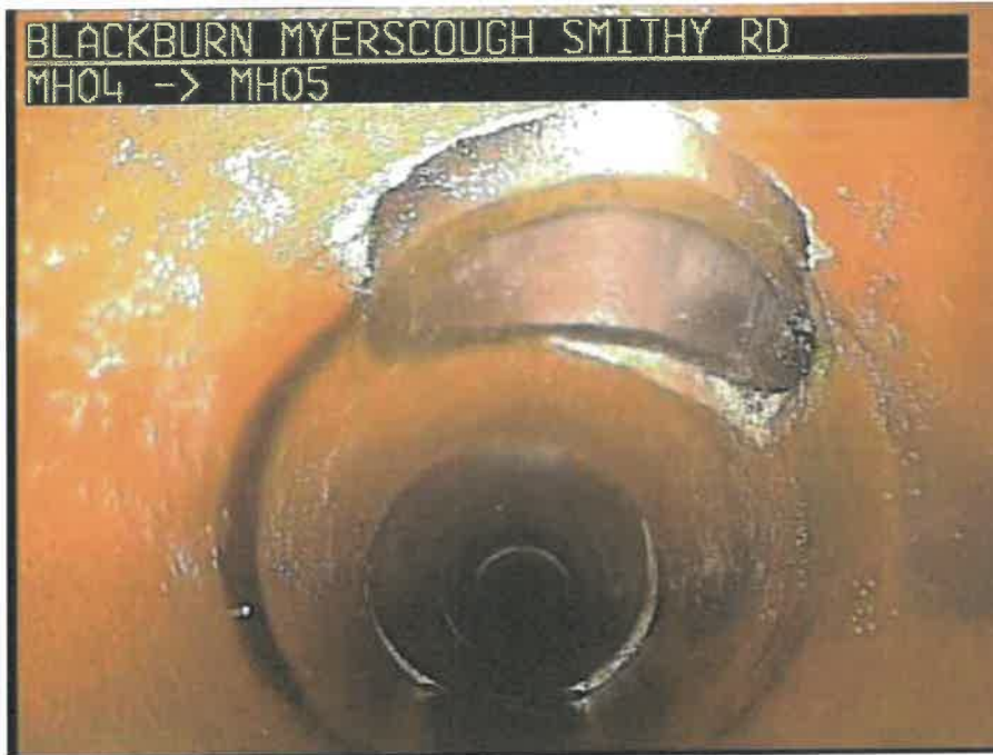
MH04X_D_13082025_1054_029.jpg, 00:00:54, 7.63 m Connection defective, connecting pipe is intruding at 12 o'clock, 100mm dia, intrusion: 5%
