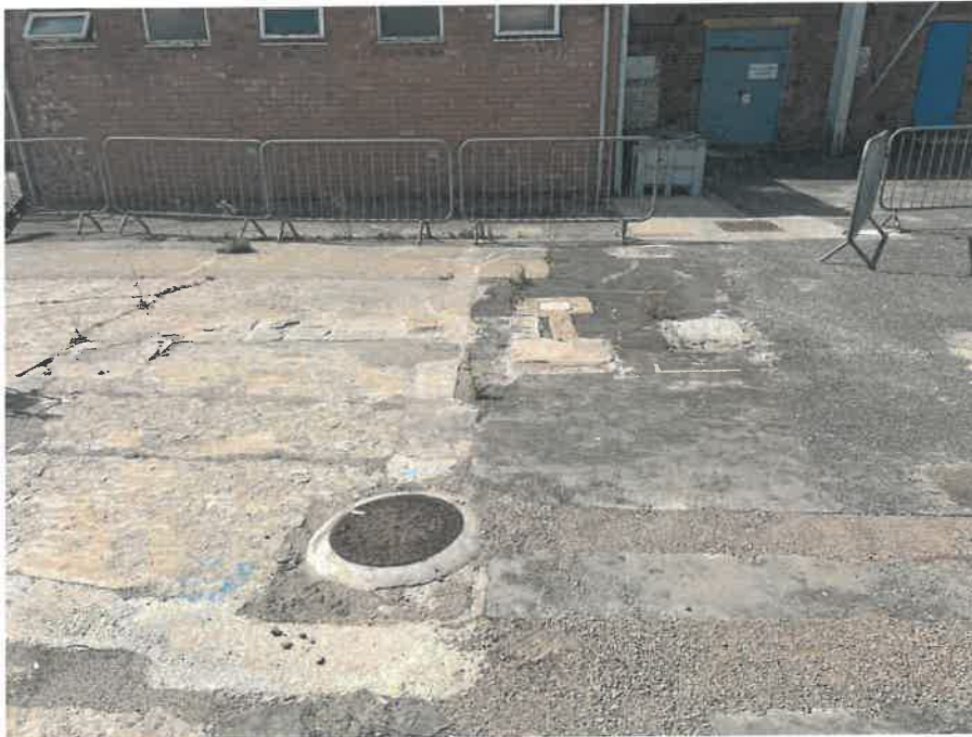
MH06X_D_13082025_1145_033.jpg, 00:00:00, 0.00 m Start node, inspection chamber, reference: MH06, IC LOCATED ADJACENT TO FILTER STORES
