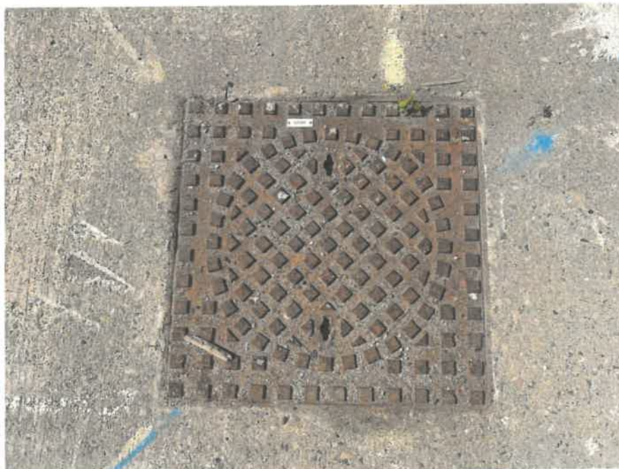
MH03X_U_13082025_1034_020.jpg, 00:01:47, 13.00 m Finish node, manhole, reference: MH03, MANHOLE LOCATED ADJACENT TO COOLING UNIT UTR
