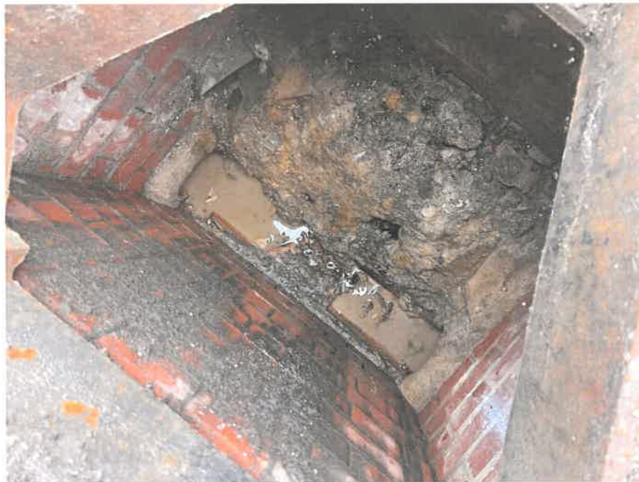
MH04BX_U_13082025_1225_046.jpg, 00:00:00, 0.00 m Start node, manhole, reference: MH04, MANHOLE LOCATED ADJACENT TO DUCTING
