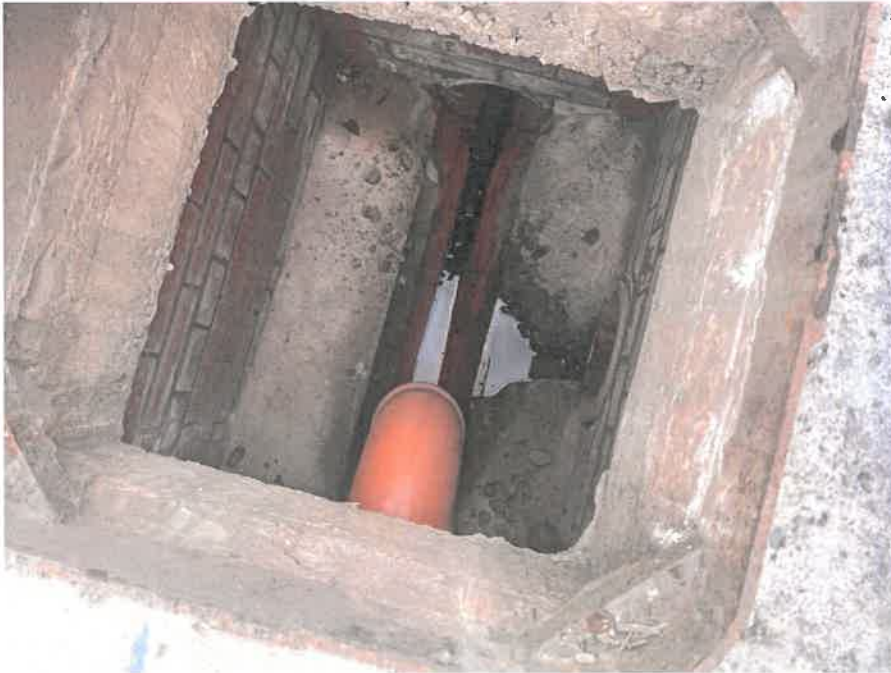
MH08AX_U_14082025_1232_063.jpg, 00:00:00, 0.00 m Start node, manhole, reference: MH08, MANHOLE LOCATED ADJACENT TO LOADING BAY
