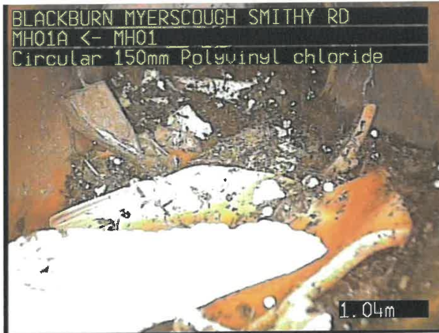
MH01AX_U_13082025_0954_010.jpg, 00:00:27, 1.02 m Settled deposits, fine, 10% cross-sectional area loss
