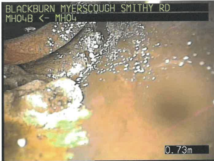
MH04BX_U_13082025_1225_047.jpg, 00:00:08, 0.60 m Joint displaced, large
