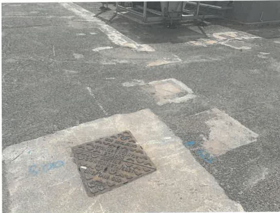
MH07X_D_14082025_1308_058.jpg, 00:00:00, 0.00 m Start node, manhole, reference: MH07, MANHOLE LOCATED ADJACENT TO COOLING STATION
