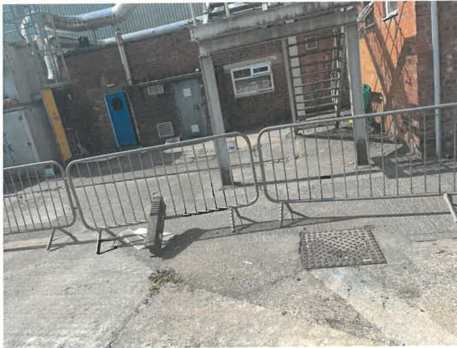
MH02AX_U_13082025_1026_011.jpg, 00:00:00, 0.00 m Start node, manhole, reference: MH02, MANHOLE LOCATED ADJACENT TO STAIR CASE
