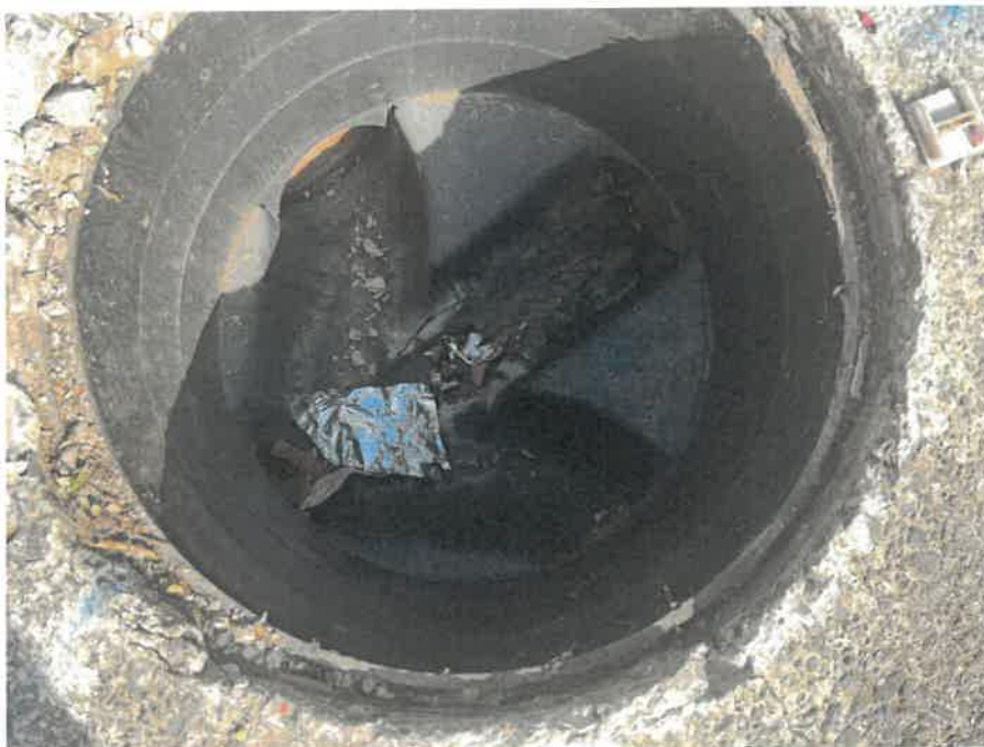
MH01X_D_13082025_0951_002.jpg, 00:00:00, 0.00 m Start node, inspection chamber, reference: MH01, IC LOCATED ADJACENT TO STAIRCASE
