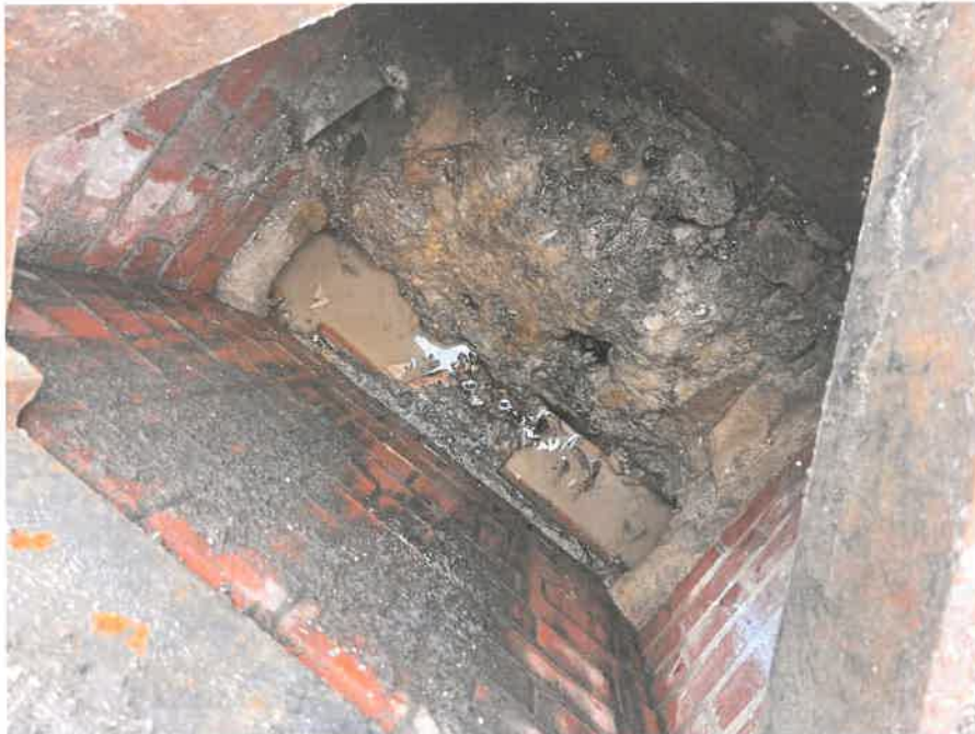
MH04AX_U_13082025_1217_040.jpg, 00:00:00, 0.00 m Start node, manhole, reference: MH04, MANHOLE LOCATED ADJACENT TO DUCTING
