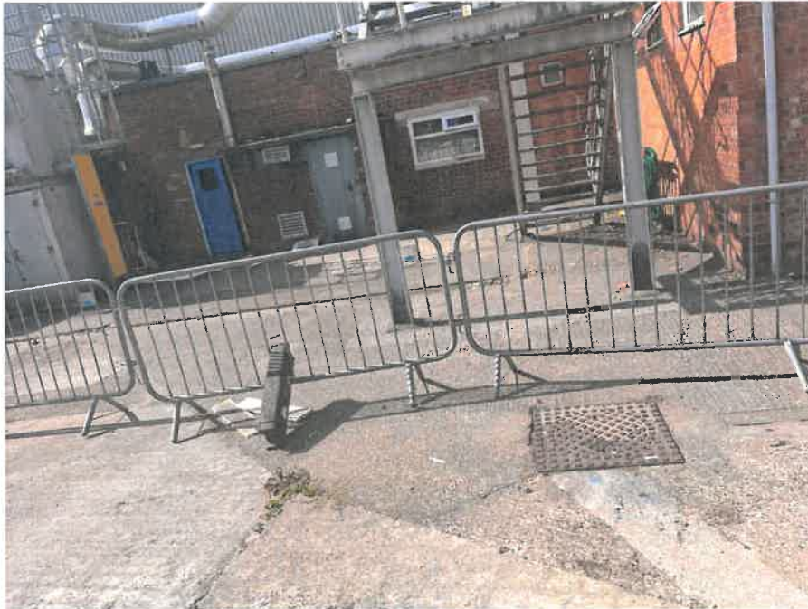
MH03X_U_13082025_1034_013.jpg, 00:00:00, 0.00 m Start node, manhole, reference: MH02, MANHOLE LOCATED ADJACENT TO STAIRCASE
