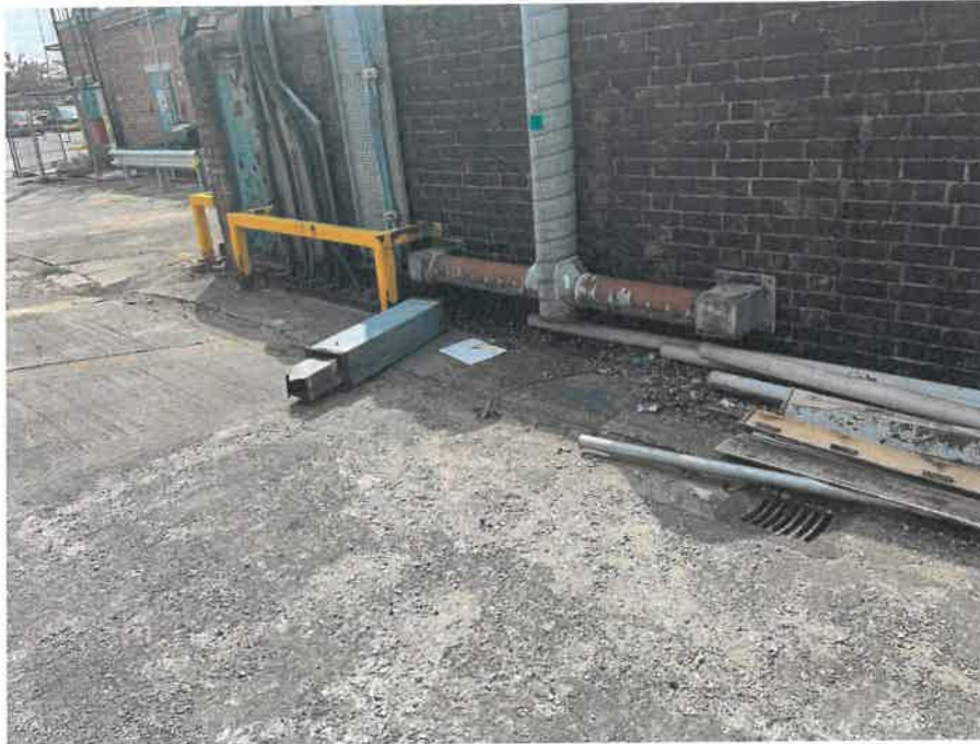
MH04X_D_13082025_1054_025.jpg, 00:00:00, 0.00 m Start node, manhole, reference: MH04, MANHOLE LOCATED ADJACENT TO DUCTING
