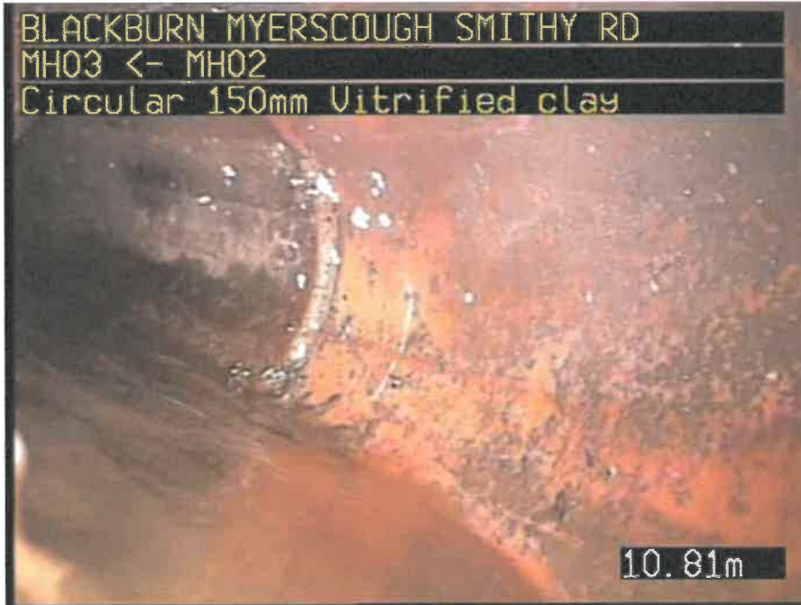
MH03X_U_13082025_1034_017.jpg, 00:01:45, 11.28 m Settled deposits, fine, 10% cross-sectional area loss, finish
