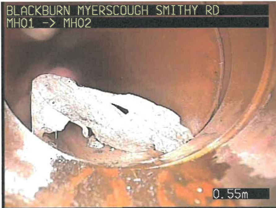
MH01X_D_13082025_0951_003.jpg, 00:00:14, 0.55 m Settled deposits, other, 5% cross-sectional area loss, DEBRIS
