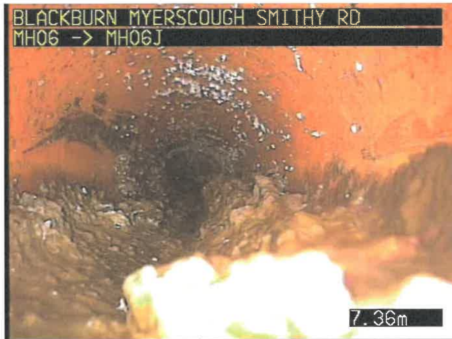
MH06X_D_13082025_1145_036.jpg, 00:00:39, 7.36 m Settled deposits, fine, 20% cross-sectional area loss, change
