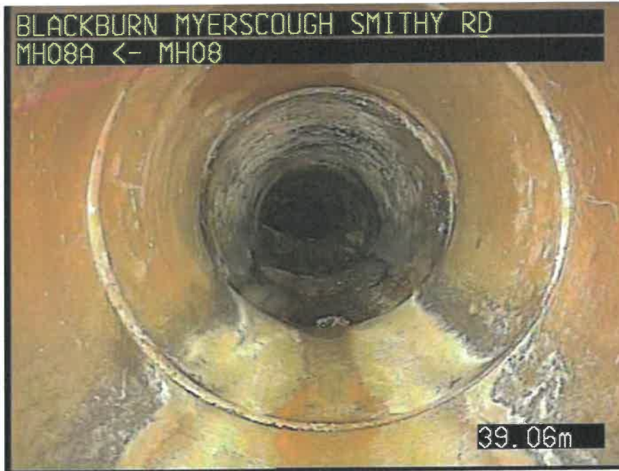
MH08AX_U_14082025_1232_069.jpg, 00:04:59, 39.06 m Crack, longitudinal at joint at 3 o'clock
