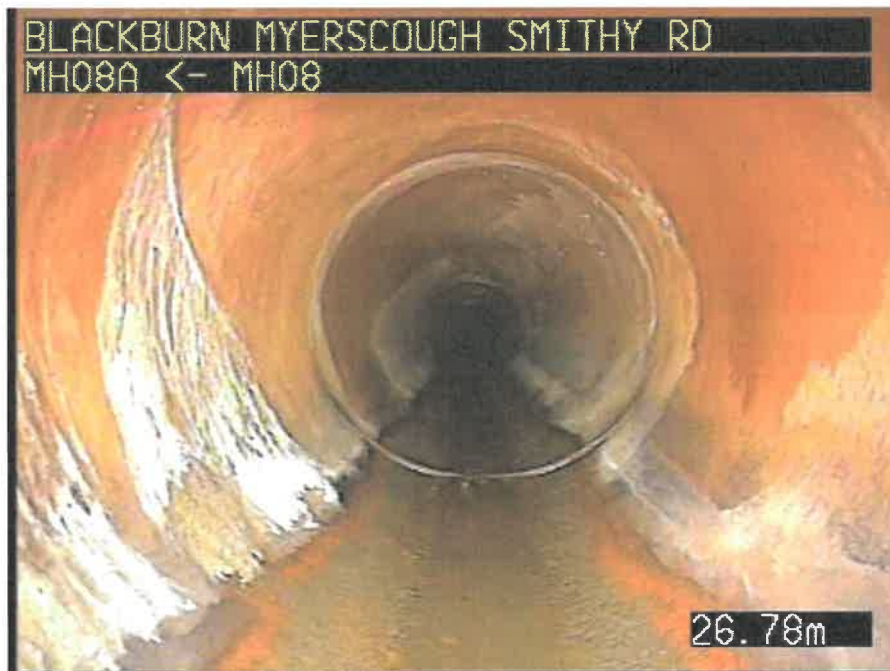
MH08AX_U_14082025_1232_068.jpg, 00:02:36, 26.78 m Attached deposits, encrustation from 9 o'clock to 11 o'clock, 5% cross-sectional area loss
