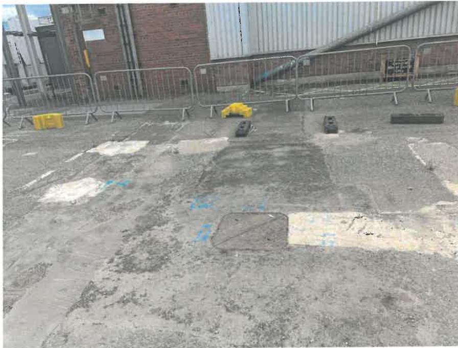
MH07X_U_14082025_1229_053.jpg, 00:00:00, 0.00 m Start node, manhole, reference: MH08, MANHOLE LOCATED ADJACENT TO LOADING BAY
