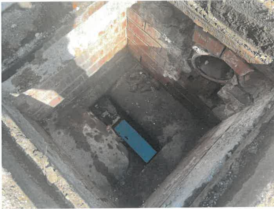
MH01X_D_13082025_0951_005.jpg, 00:00:30, 2.99 m Finish node, manhole, reference: MH02, MANHOLE LOCATED ADJACENT TO STAIRCASE
