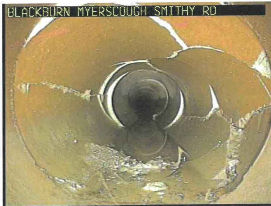
MH08X_D_14082025_1244_083.jpg, 00:06:41, 36.62 m Broken pipe from 12 o'clock to 12 o'clock
