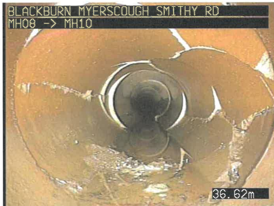
MH08X_D_14082025_1244_085.jpg, 00:06:47, 36.62 m Settled deposits, fine, 5% cross-sectional area loss, finish
