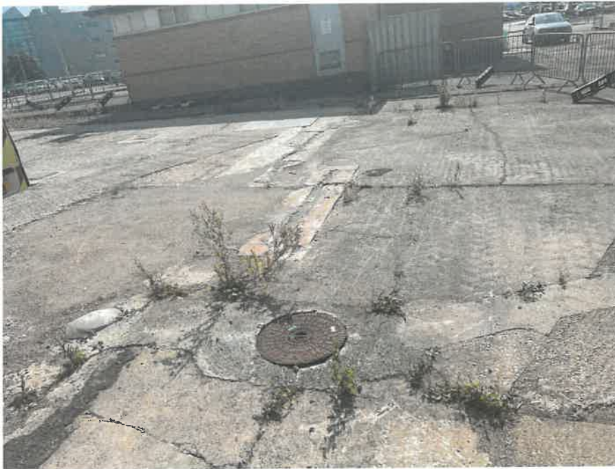
MH01X_D_13082025_0951_001.jpg, 00:00:00, 0.00 m Start node, inspection chamber, reference: MH01, IC LOCATED ADJACENT TO STAIRCASE
