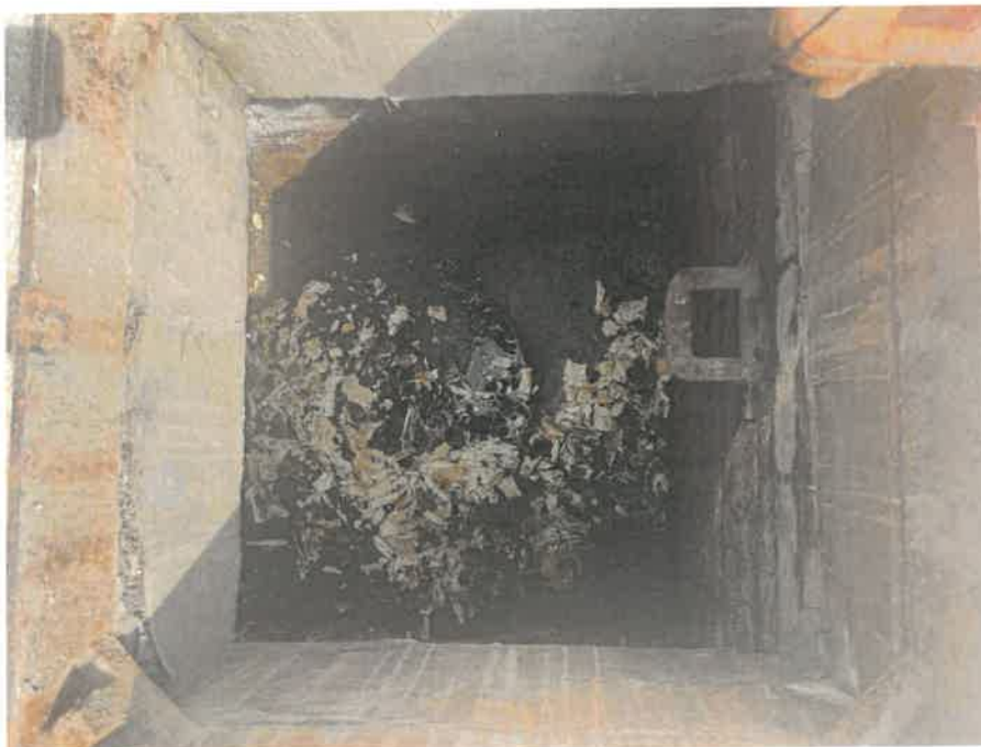
MH07X_D_14082025_1308_059.jpg, 00:00:00, 0.00 m Start node, manhole, reference: MH07, MANHOLE LOCATED ADJACENT TO COOLING STATION
