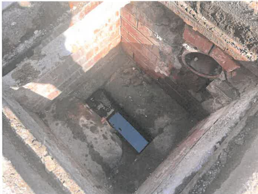
MH03X_U_13082025_1034_014.jpg, 00:00:00, 0.00 m Start node, manhole, reference: MH02, MANHOLE LOCATED ADJACENT TO STAIRCASE
