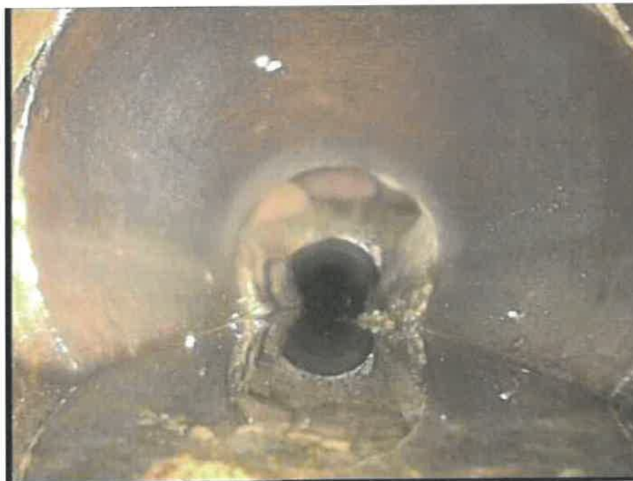
MH04X_D_13082025_1054_030.jpg, 00:01:27, 13.31 m Settled deposits, fine, 5% cross-sectional area loss
