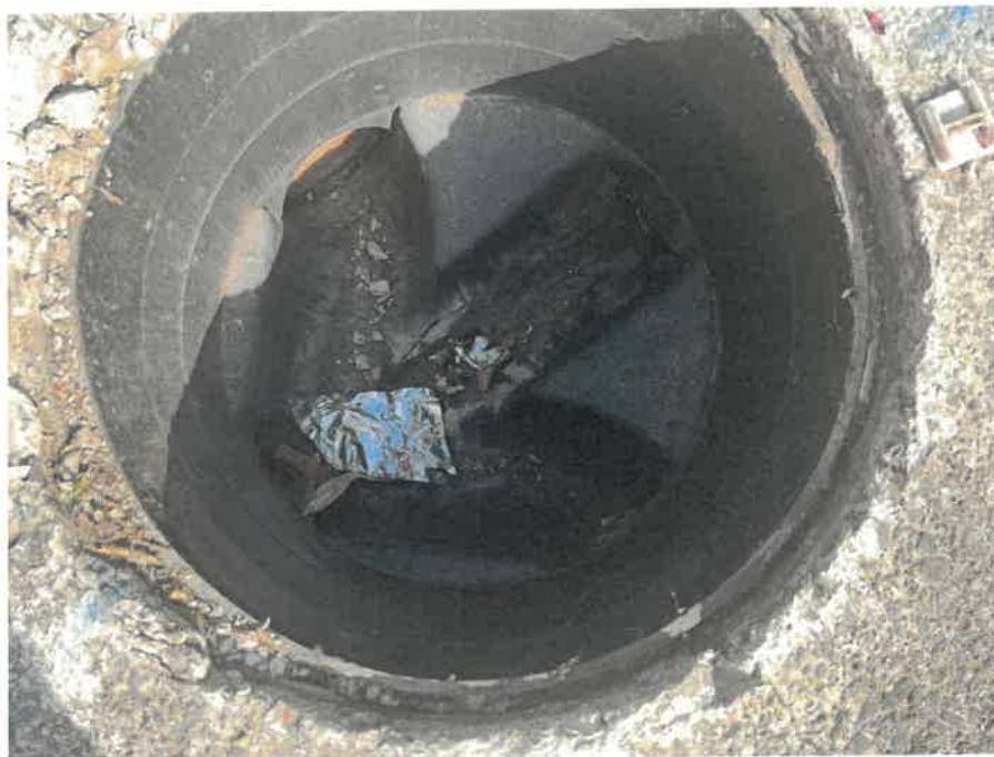
MH01AX_U_13082025_0954_007.jpg, 00:00:00, 0.00 m Start node, inspection chamber, reference: MH01, IC LOCATED ADJACENT TO STAIR CASE
