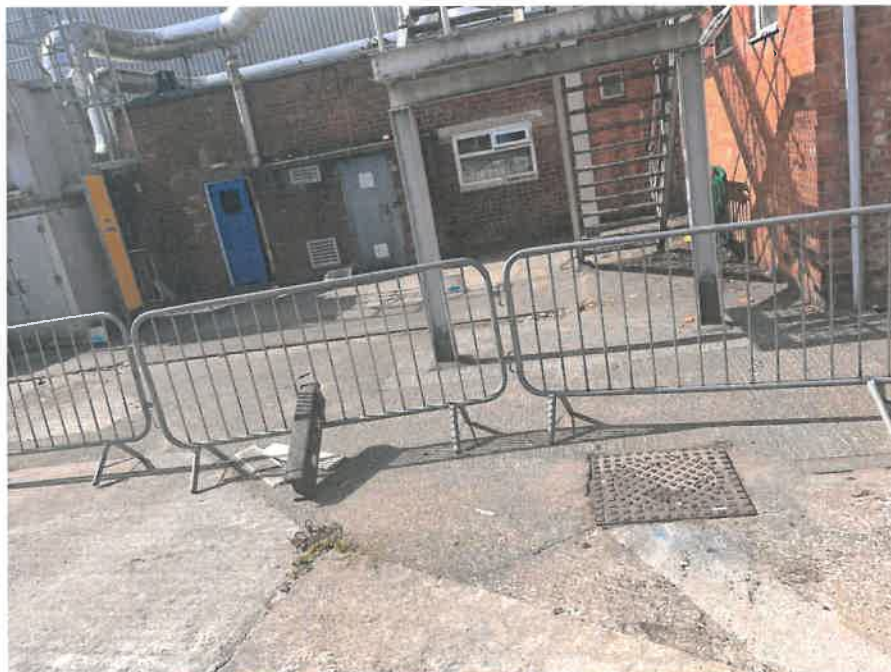
MH01X_D_13082025_0951_004.jpg, 00:00:30, 2.99 m Finish node, manhole, reference: MH02, MANHOLE LOCATED ADJACENT TO STAIRCASE
