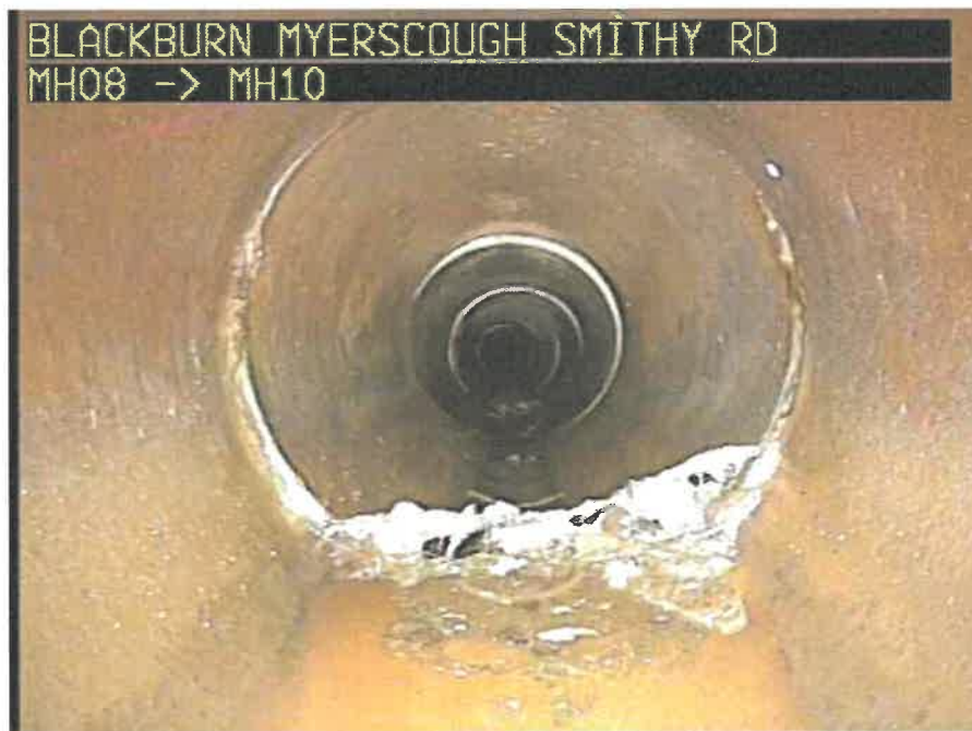
MH08X_D_14082025_1244_081.jpg, 00:06:03, 32.31 m Attached deposits, encrustation from 4 o'clock to 8 o'clock, 5% cross-sectional area loss
