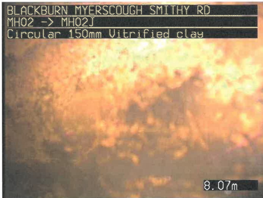
MH02X_D_13082025_1042_024.jpg, 00:01:15, 8.05 m Settled deposits, fine, 5% cross-sectional area loss, finish
