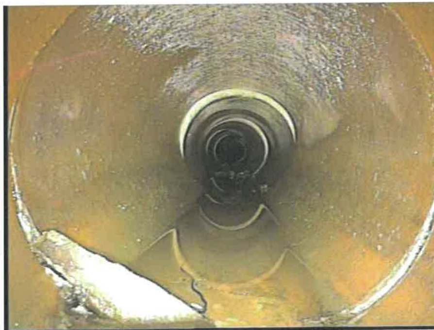
MH08X_D_14082025_1244_079.jpg, 00:03:47, 15.33 m Fracture, longitudinal at joint at 6 o'clock
