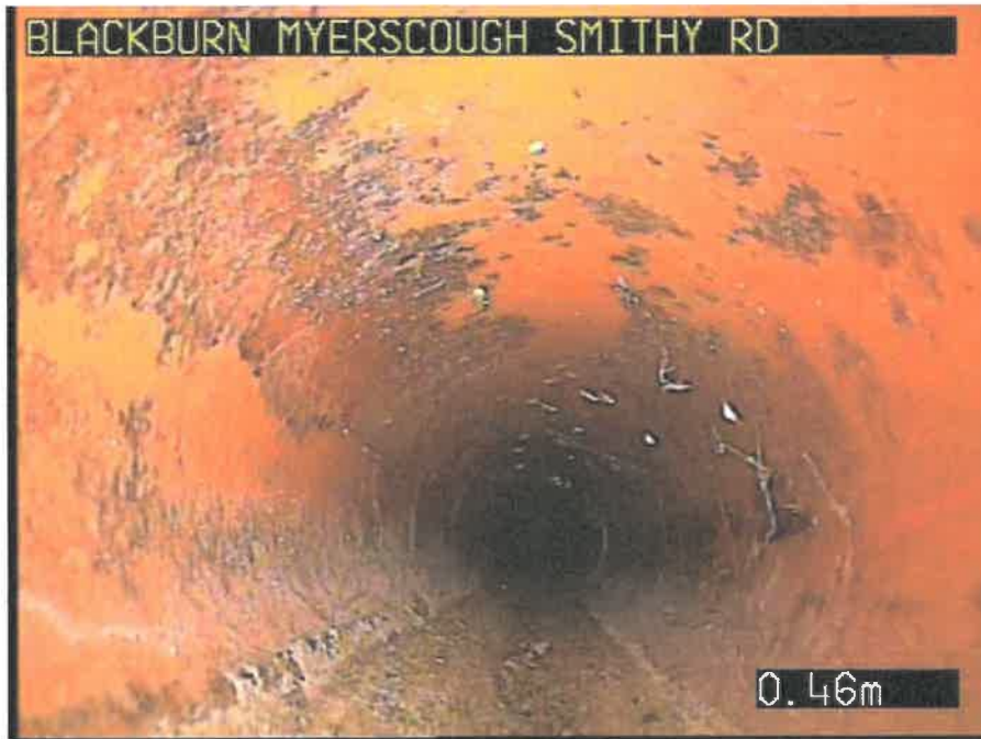
MH06X_D_13082025_1145_035.jpg, 00:00:05, 0.44 m Settled deposits, fine, 5% cross-sectional area loss, start
