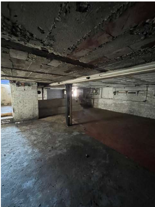
Internal photo of Lower Ground Floor. Floor constructed of steel beams with concrete floor supported between
