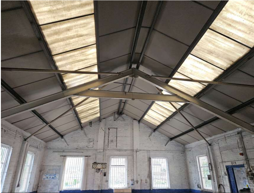
Internal photo of Ground Floor showing steel truss and purlins/ cladding rails supporting profiled roof cladding. Painted brickwork internally.
