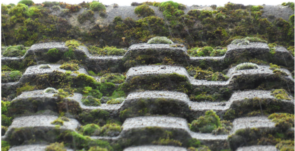
3 – Roof and ridge tiles are in good condition with no suitable gaps.
