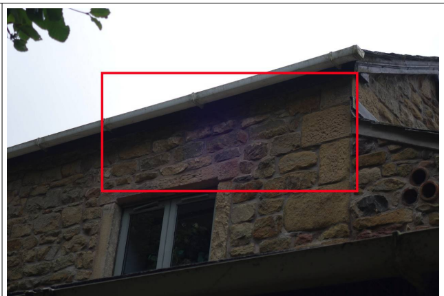
Location of bat droppings on eastern facade
