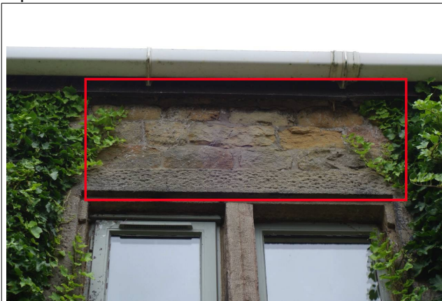
Location of bat droppings on western facade
