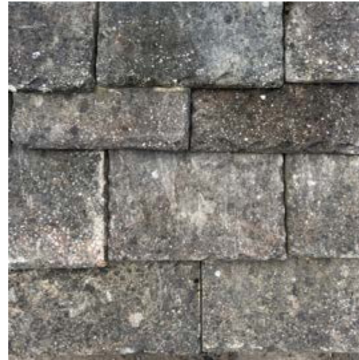
STONE ROOF PAVING FLAGS - RECLAIMED - To re roof front and rear elevations, numbering and reusing original roof flags wherever possible, topping up if required with reclaimed stone flags
