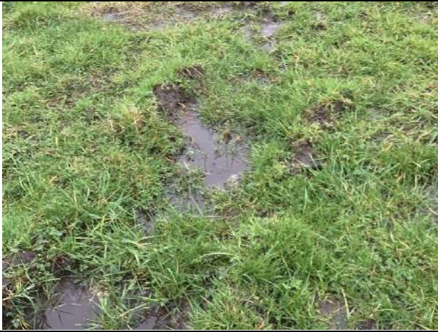
P7: Small amounts of standing water across the site.
