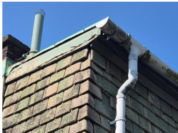
Photo 16: PRF at lifted hanging tile on extension
