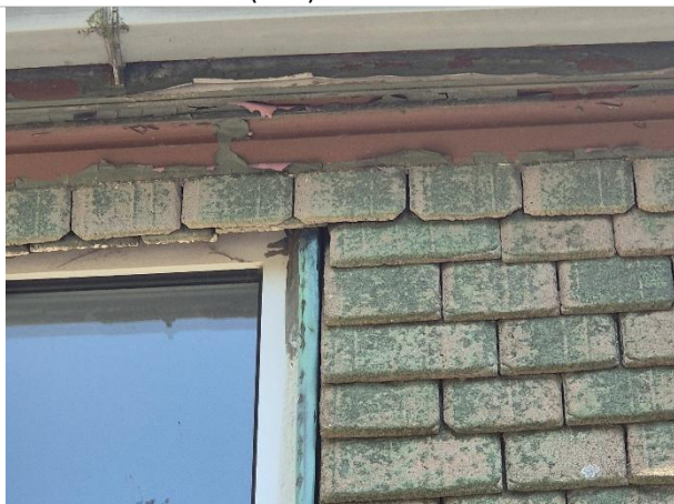
Photo 15: Gap / potential roost features (PRF) at frame between hanging tiles and window frame
