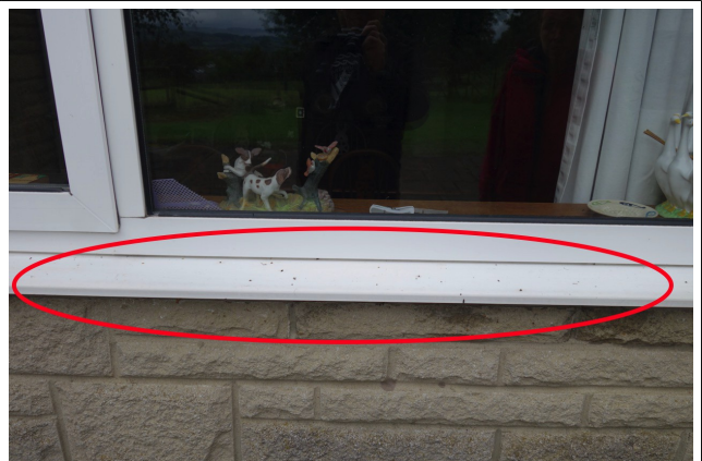
Pipistrelle droppings on window ledge on the northern gable end.
