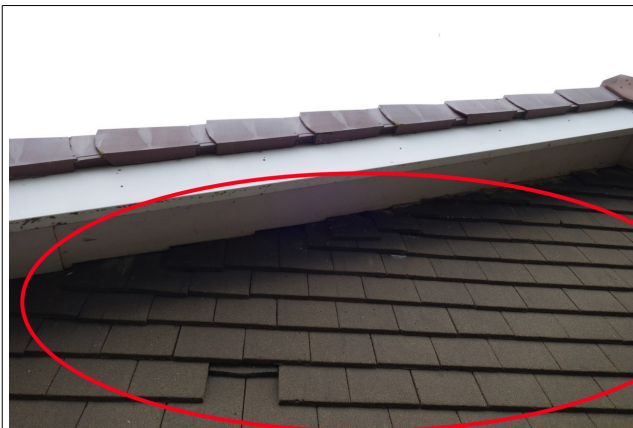
Pipistrelle droppings adhering to hanging tiles on the northern gable end.
