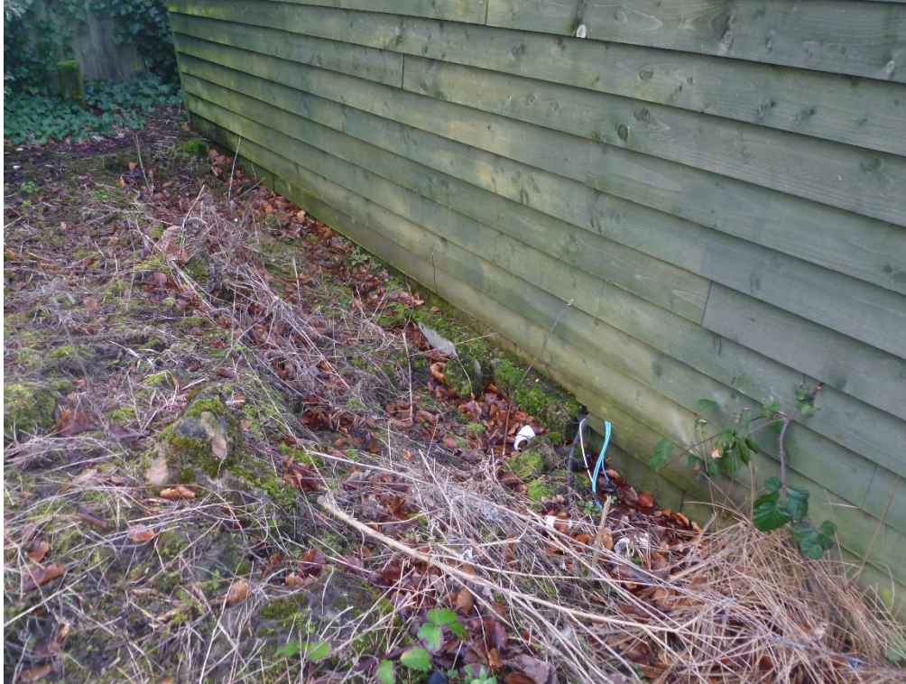
Photo 3 – High ground levels at the rear of the property
