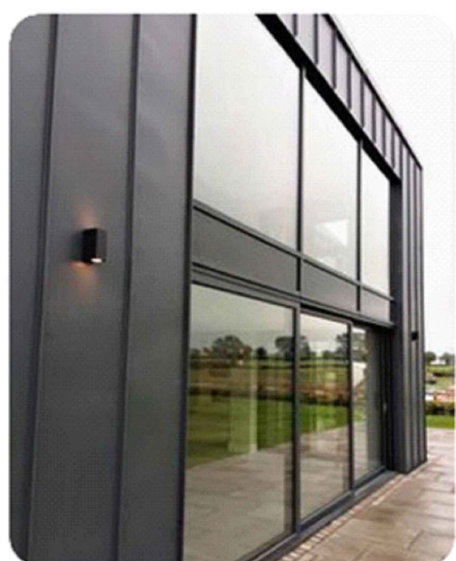
Wall cladding: Catnic - SSR2 Standing Seam Cladding - To Entrance Canopy, steel colour coated (colour tbc).
