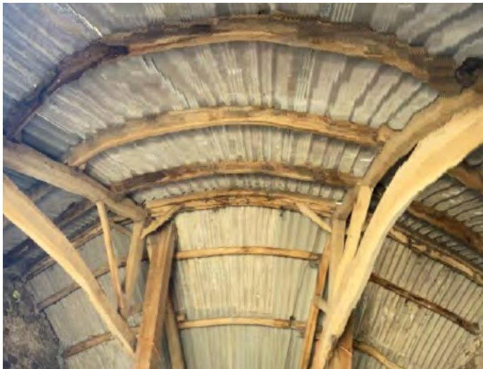
26. Central bay of main barn south slope to the top and north slope to the
