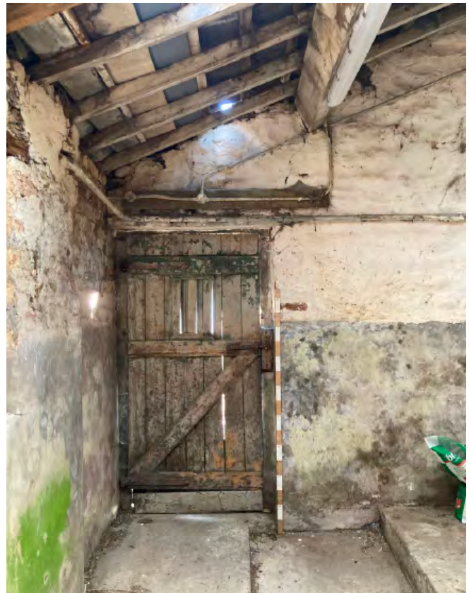
23. Doorway to east side of north shippon. Note board to base of the door covering rotten vertical boards
