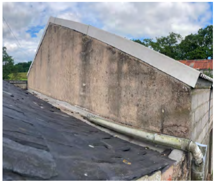
13. Lower section of shippon roof showing abutment with adjoining C20th barn. Note valley gutter appears to have no outlet.
