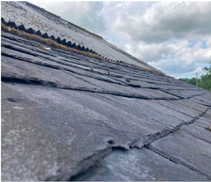
12. Slate roof to the north shippon with asbestos and cement fibre roof sheets to main barn above.
