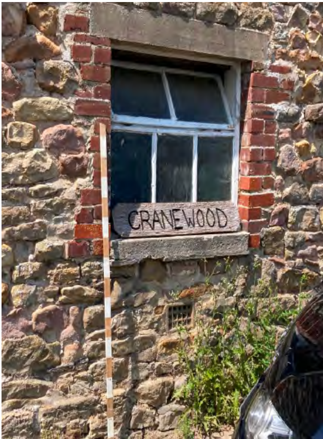
8. South window to east elevation showing concrete head, cill and roughly built brickwork to the jambs.
