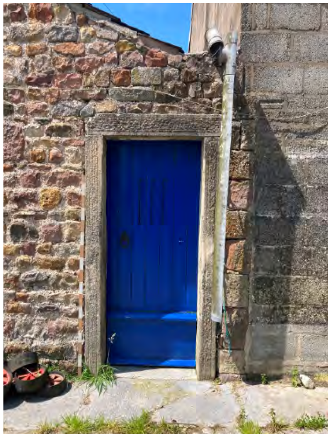
11. Doorway to east side of northern shippon with original stone surround. Note board to the base of the door covering rotten vertical boards.
