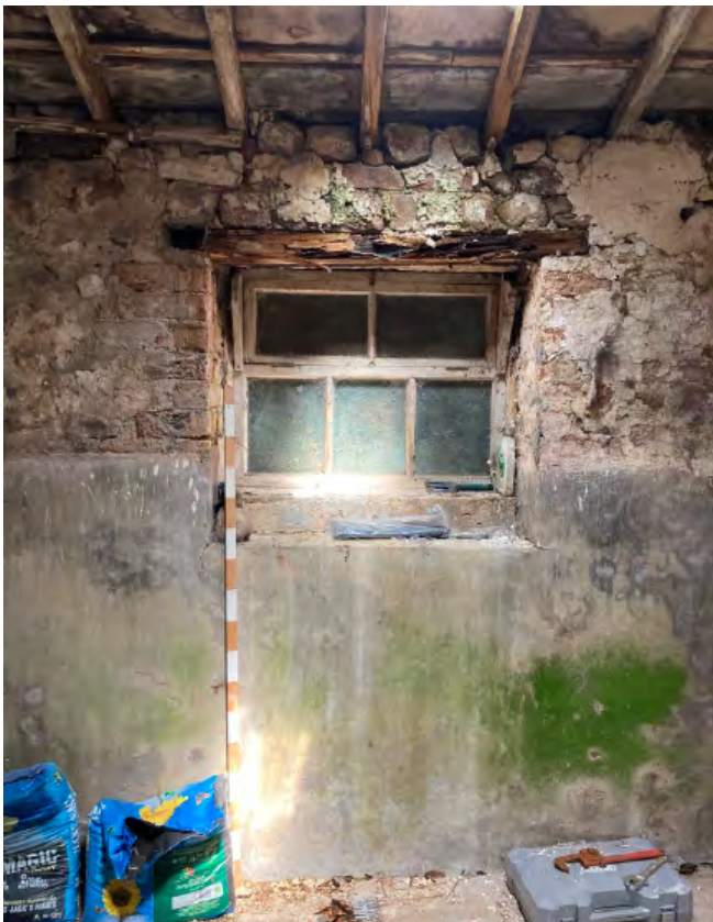
22. Window to north wall of north shippon with lower cementitious plaster and limewash above. Also note decay to the timber lintel.
