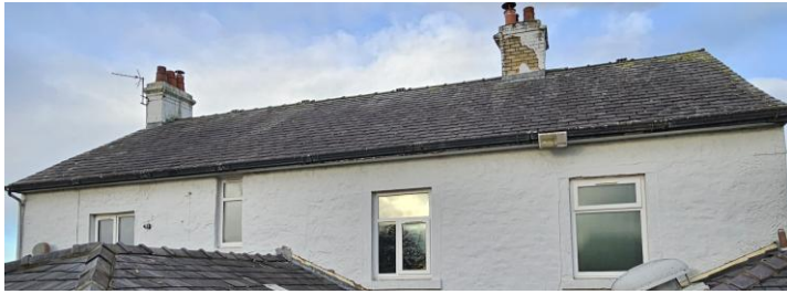
The first-floor rear elevation of the main building being retained (southeast elevation)
